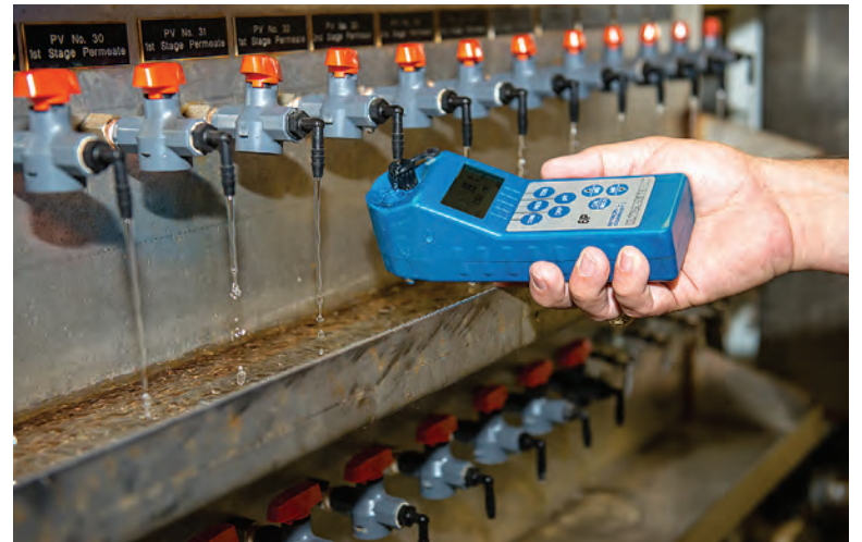
Team members use an Ultrameter II (Myron L Company) to measure the total dissolved solids in the RO system's individual pressure vessels.
