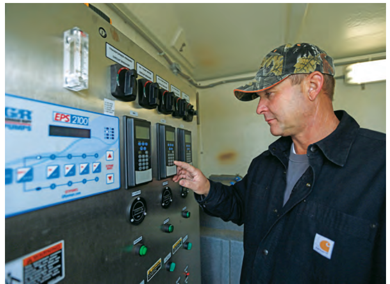
Jeff Smith checks on a lift station (pumps from Gorman-Rupp Co.).
