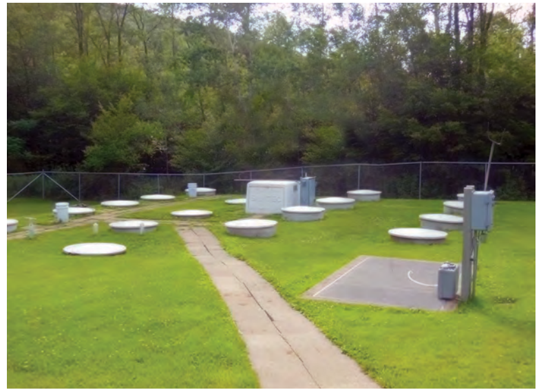
Hamilton Township (Pennsylvania) Wastewater Treatment Plant.
