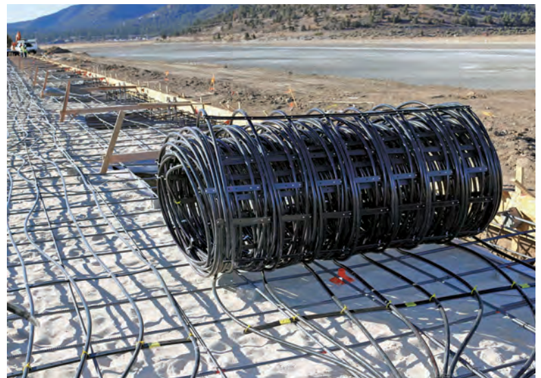
The size of the slab made the project well suited for the Viega Climate Mat system for slabs 10,000 square feet and larger.
