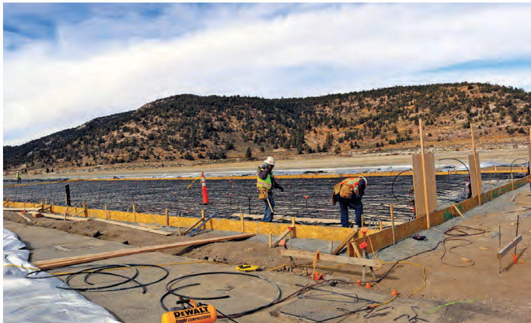
Workers lay the tubing that will carry hot water for radiant heating of the slab in the building in which biosolids are dried.
