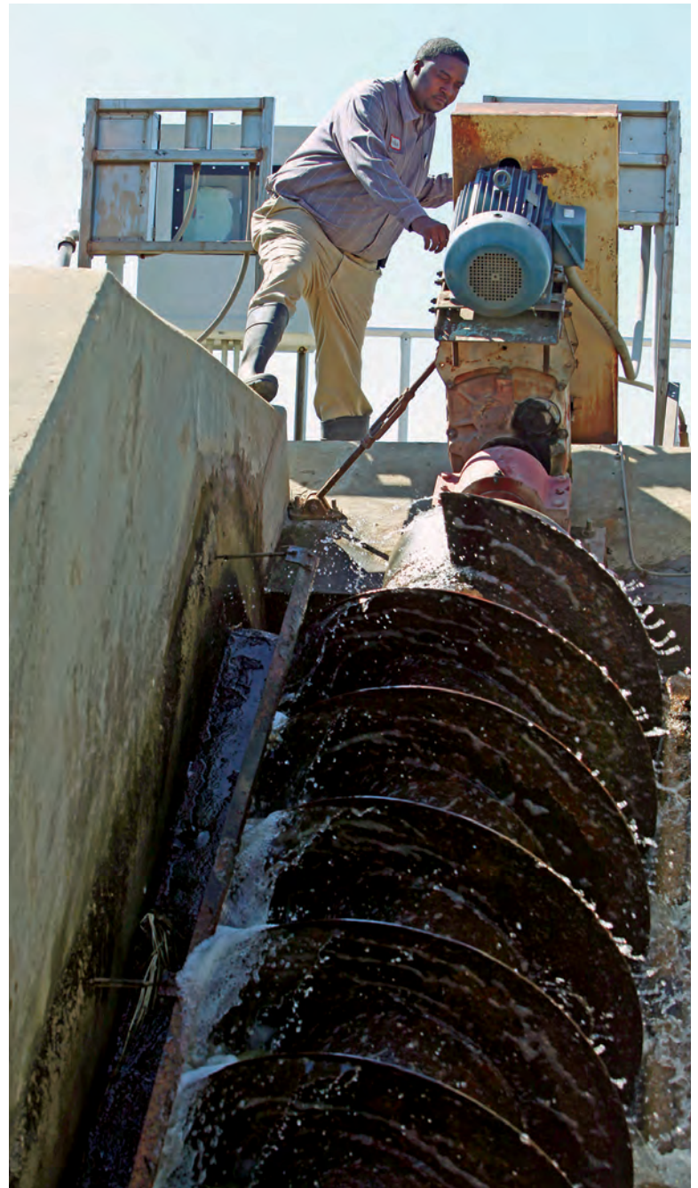
Kelvin Brooks at the wastewater treatment plant's effluent pump station.
