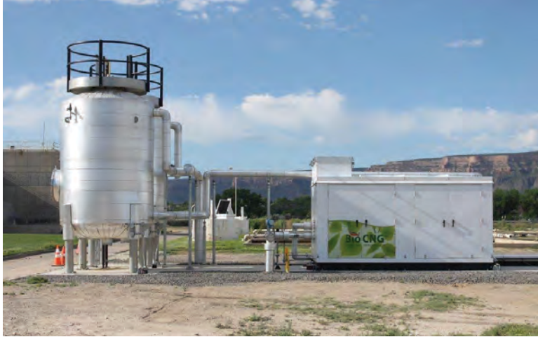
After biogas is cleaned and compressed, it is piped to a CNG fueling station so employees don’t waste fuel and time driving 6 miles to the wastewater treatment plant.
