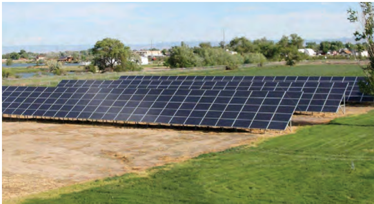
The Persigo plant also uses renewable energy with a 98 kW Sunsense solar photovoltaic system installed in 2011.
