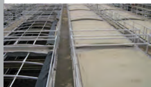
Retractable covers from Geomembrane Technologies
