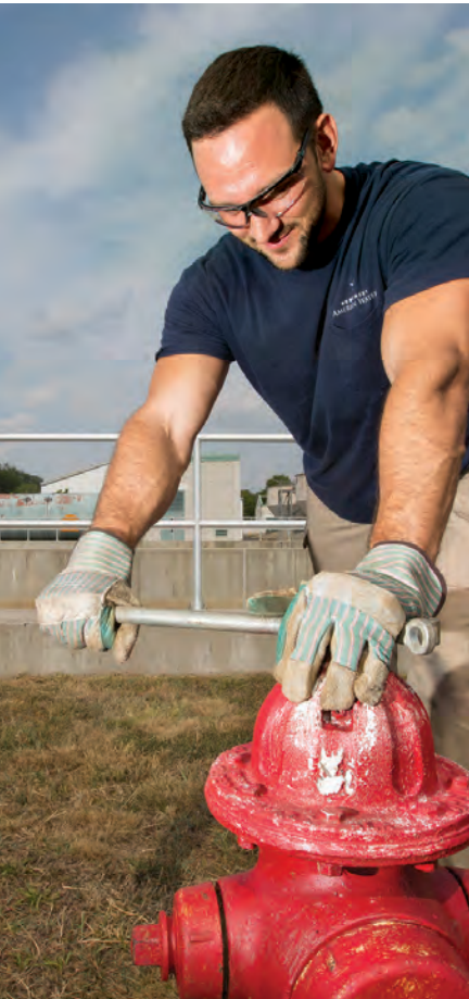
David Soltis flushes a hydrant as part of the town's distribution system maintenance program.
