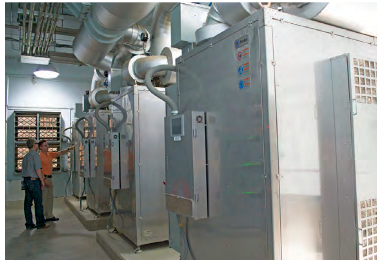
New blowers from Aerzen save the facility about $100,000 per year in energy costs.
