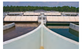
Closed-loop reactor process from Lakeside Equipment Corporation
