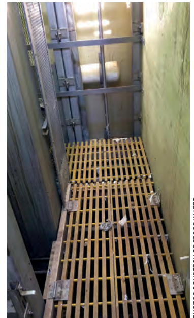
The new ladder and grating inside the lift station vault enables safe entry for workers.
