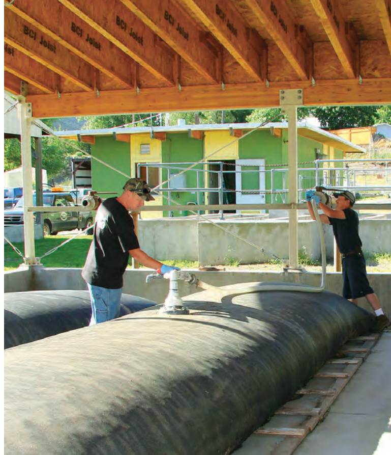
The plant uses Geotube technology (TenCate) for biosolids dewatering.
