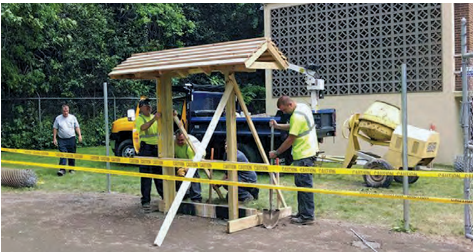
Brunswick Sewer District employees construct a new kiosk at the entrance to the town’s Water Street pump station.
