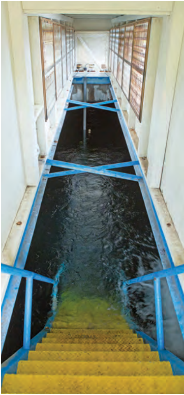
Finished water in the clearwell typically has 0.05 NTU turbidity.
