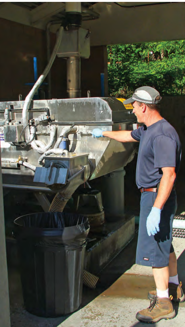
Ross Campbell, with the facility’s Salsnes Filter system for liquid-solids separation.
