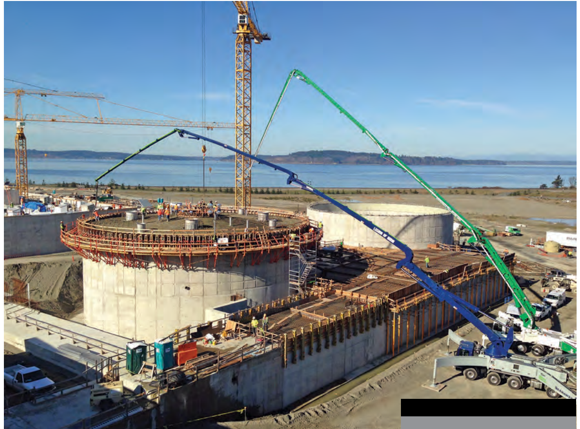
The Chambers Creek Regional Wastewater Treatment Plant is shown during the recent expansion project.
