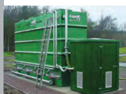
SAF (Submerged Aerated Filter) from PWTech
