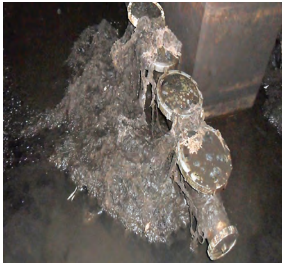
Rags clogging a basin’s aeration system.
