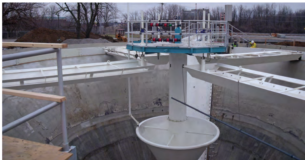
The clarifier project required a coating system with strong edge retention on submerged and wetted surfaces to help extend service life.
