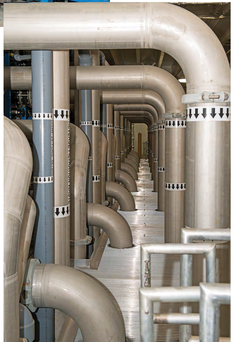
Outflow tubes from the membrane racks that send the water through the primary disinfection treatment pipeline.
