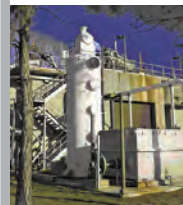
ZABOCS Bio-Trickling Filter system from Evoqua Water Technologies
