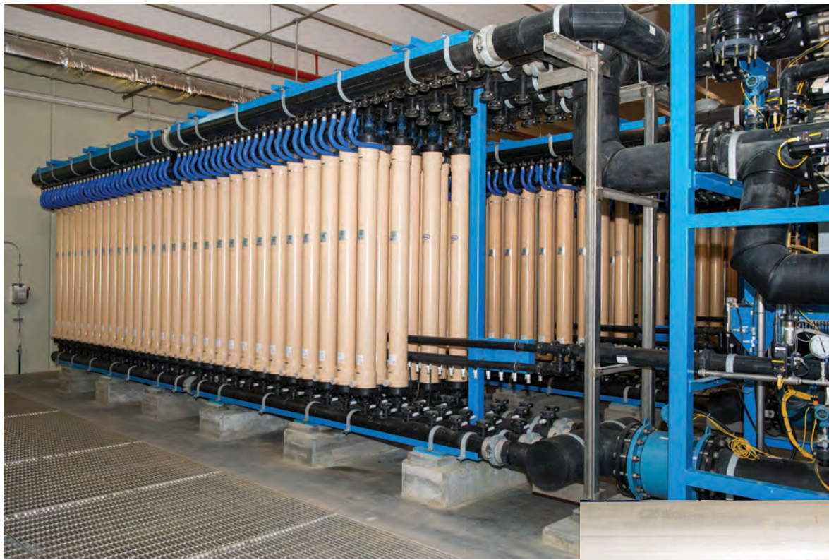
The membrane treatment system uses Microza UNA-620A membrane modules (Pall Corporation). Each membrane rack can hold 150 modules.
