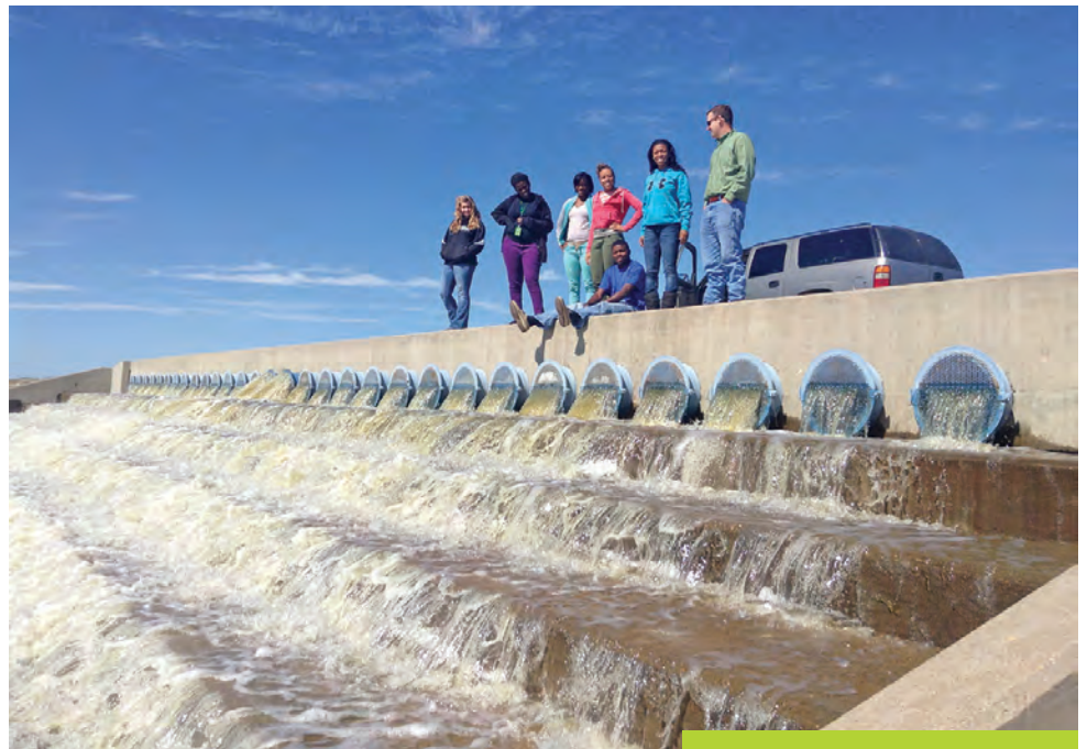
Members of a high school group at the finished water discharge into Richland-Chambers Reservoir.
