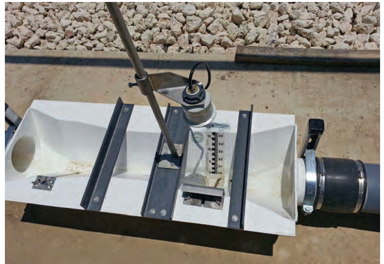
A Plasti-Fab flume with Hach ultrasonic sensor meters flow to the sewer.
