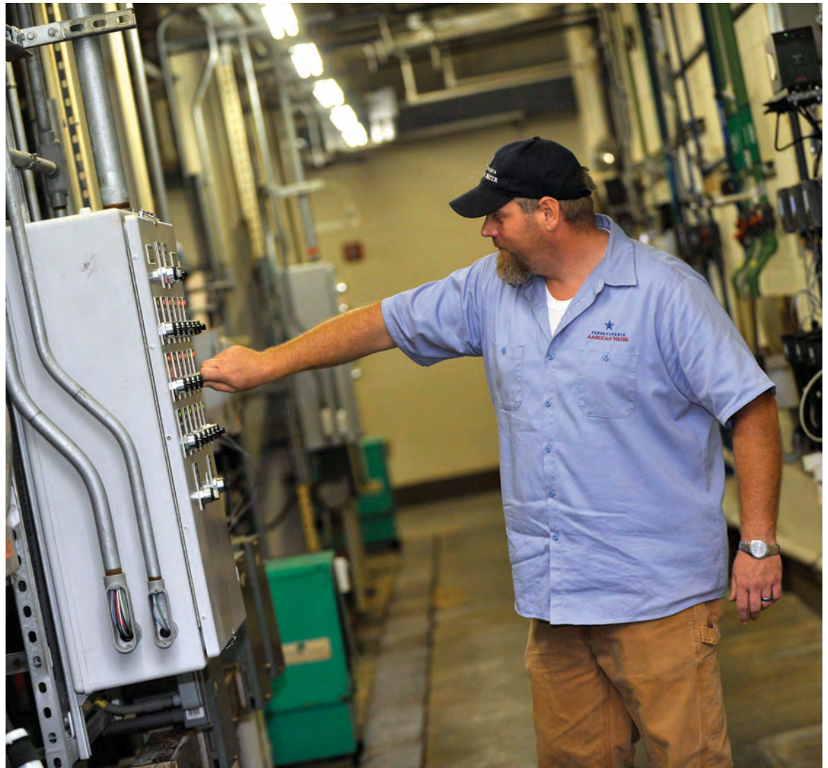
Harry Foster, maintenance/relief operator, checks the valve panel.
