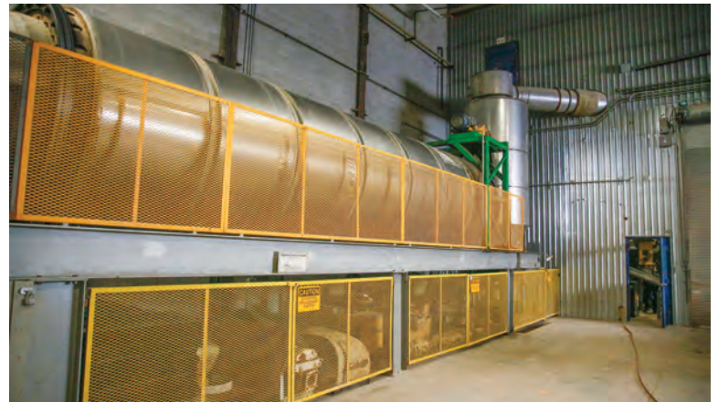
The rotary dryer (Uzelac Industries) receives material at 45-50 percent solids, pulls some 15,000 cfm of air through the drying chamber, and evaporates about 10 tons of water an hour.
