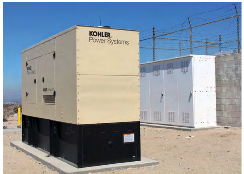
An electrical upgrade at the East Valley plant included a new vertical turbine motor, permanent generator, motor controls, and SCADA network connections.
