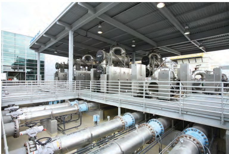
UV and hydrogen peroxide disinfection are used in the Groundwater Replenishment System. Its end product supplements the drinking-water supply of semi-arid Orange County.
