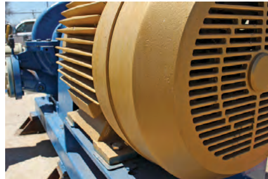
To make the best use of an existing pipeline and site space, the facility team installed a new split-case pump and motor (Nidec Motor Corp.), designed to run 10 hours per day during the summer.
