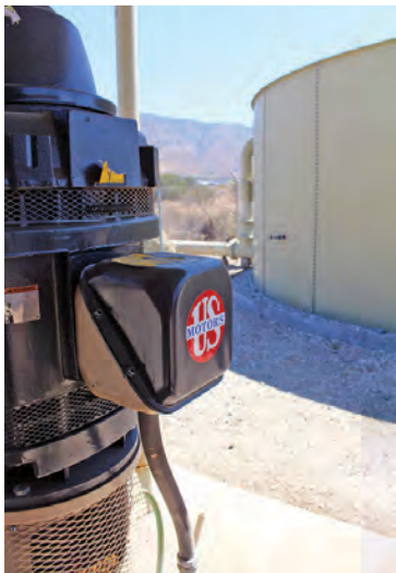
Four wells like this one pump to a newly constructed reservoir. This site received a downsized well designed to run more efficiently for longer durations.
