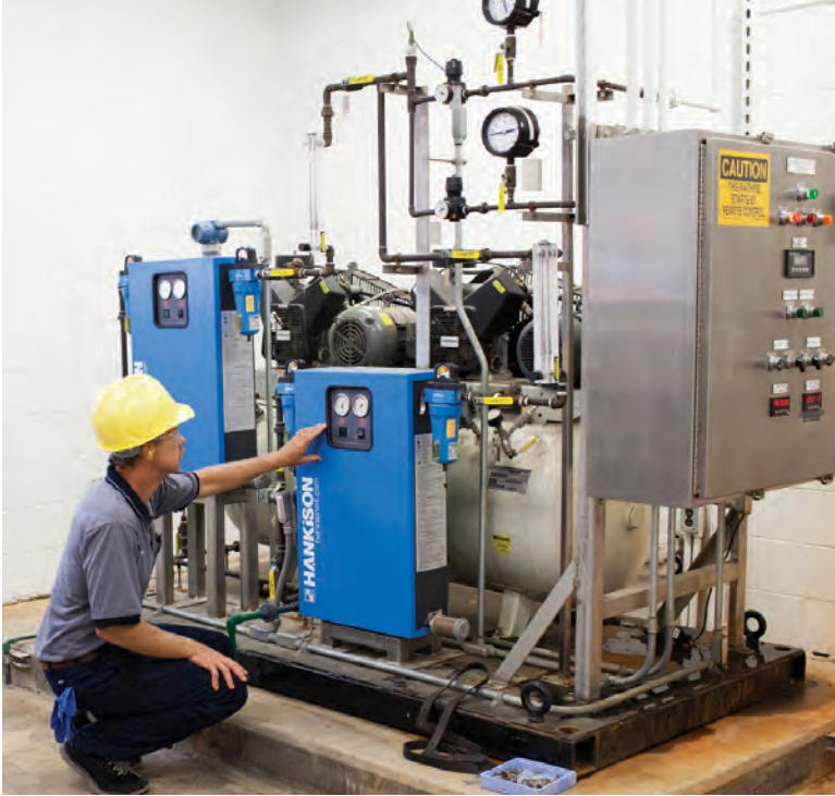
Steve Patelski checks the Hankison nitrogen boost system (SPX) that operates in conjunction with the plant's ozone generation process.
