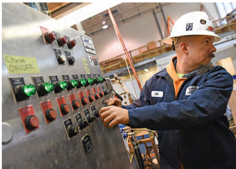
Victor Ward works on the facility’s belt press (BDP Industries).
