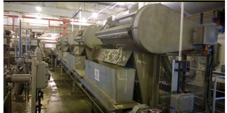
Four (4) 6' wide by 14'-6" deep catenary screens. Operating at Bucklin Point WWTP in East Providence, RI since 2002.
