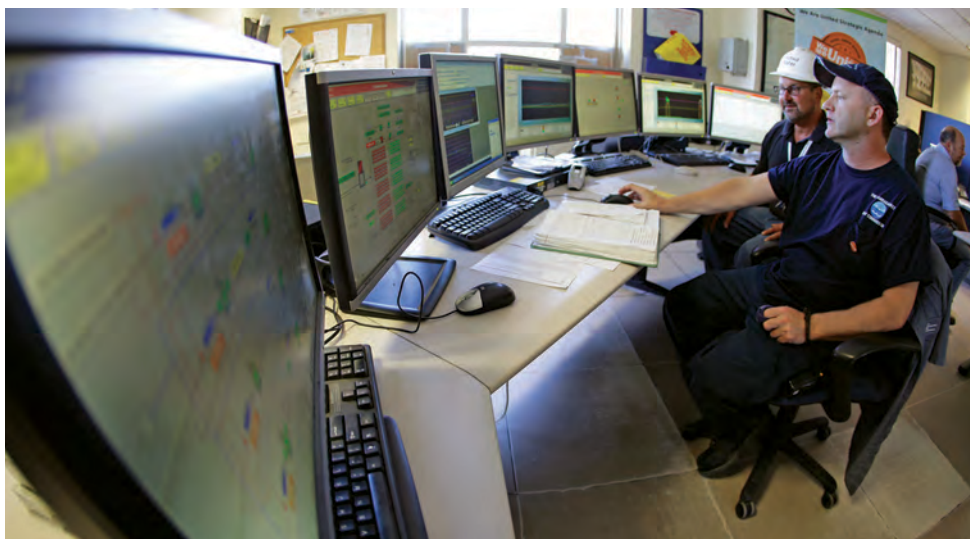
Marc Pariseault, assistant superintendent (left), and Bill Dolan, operator, in the Bucklin Point facility's SCADA center.
