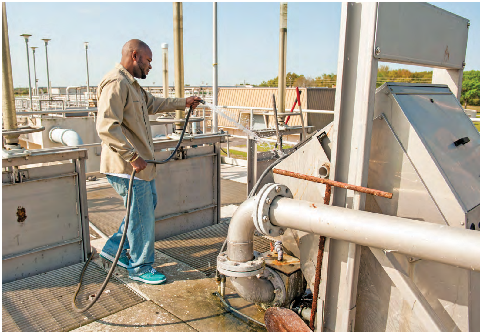
Marcus Hamilton, Class C wastewater operator, cleans a bar screen (Huber Technology) in the plant headworks.
