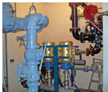
This process water pump system enables use of reclaimed effluent for in-plant purposes, saving 4 million gallons of potable water per year.
