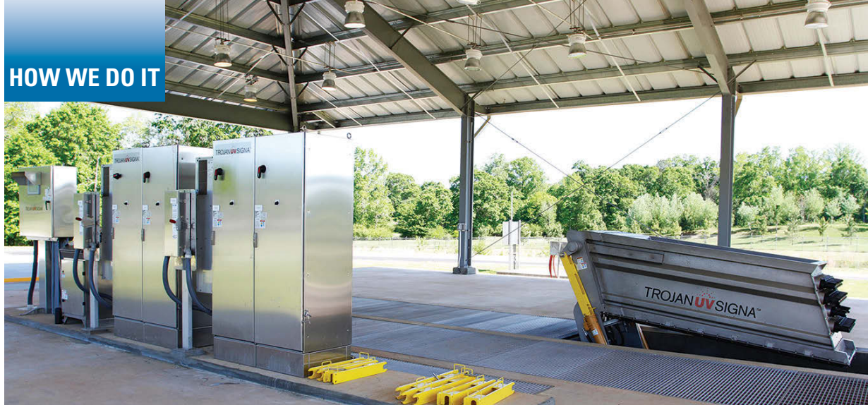
A UV system replaced gaseous chlorine disinfection at the H.C. Morgan Water Pollution Control Facility in Auburn, Ala.
