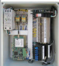
ScalableSCADA from Revere Control Systems
