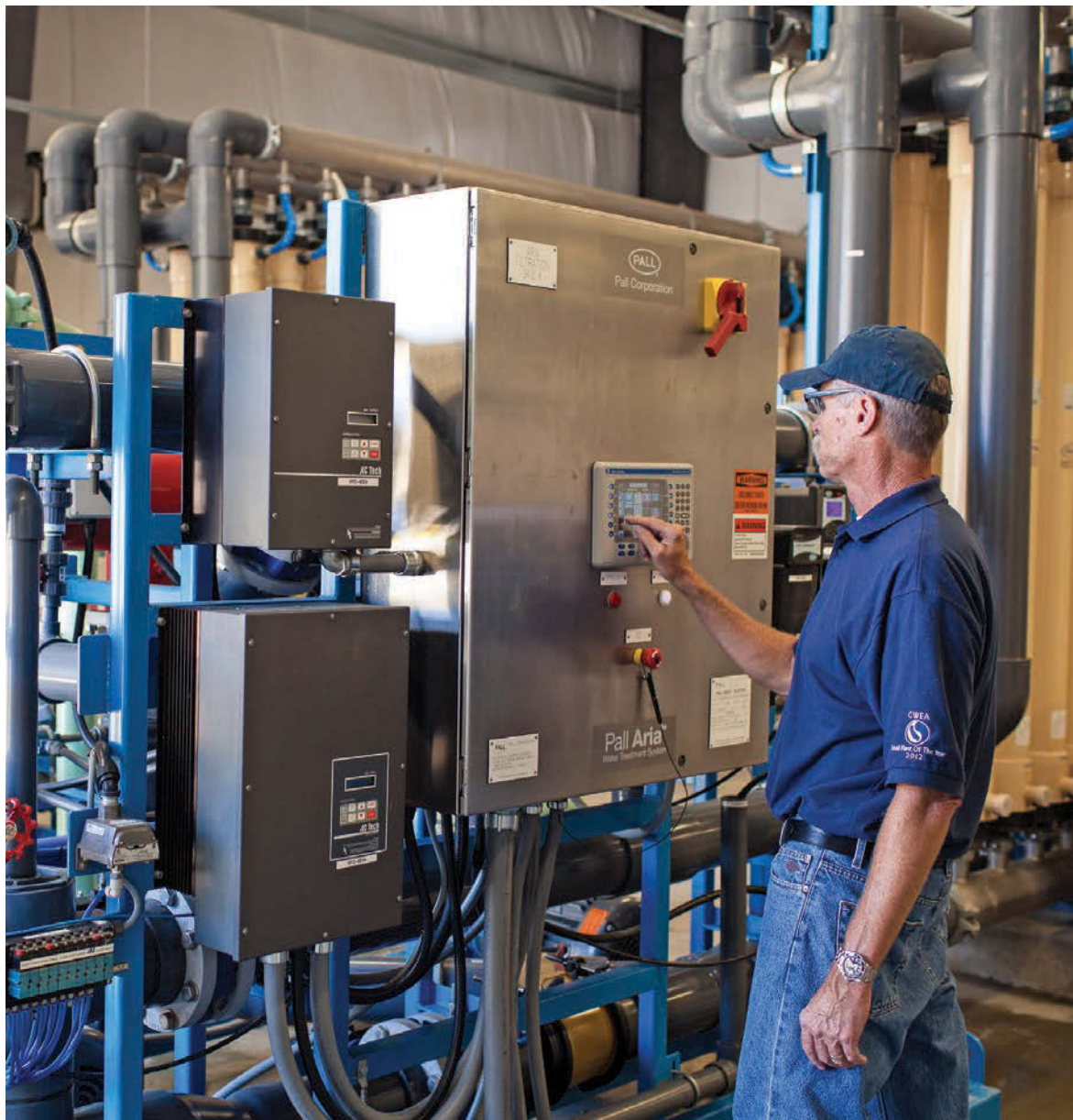
Bob Bobik performs a quick systems check of the Aria microfiltration system (Pall Corp.) using the PanelView Plus 700 control panel (Allen-Bradley/Rockwell Automation). The system has a 1 mgd capacity.
