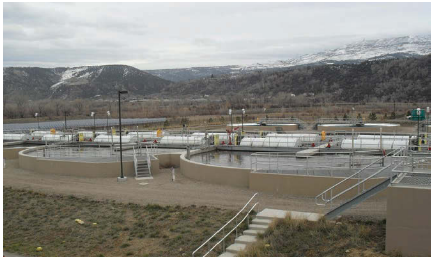
The oxidation ditches at the Rifle Regional Wastewater Reclamation Plant.
