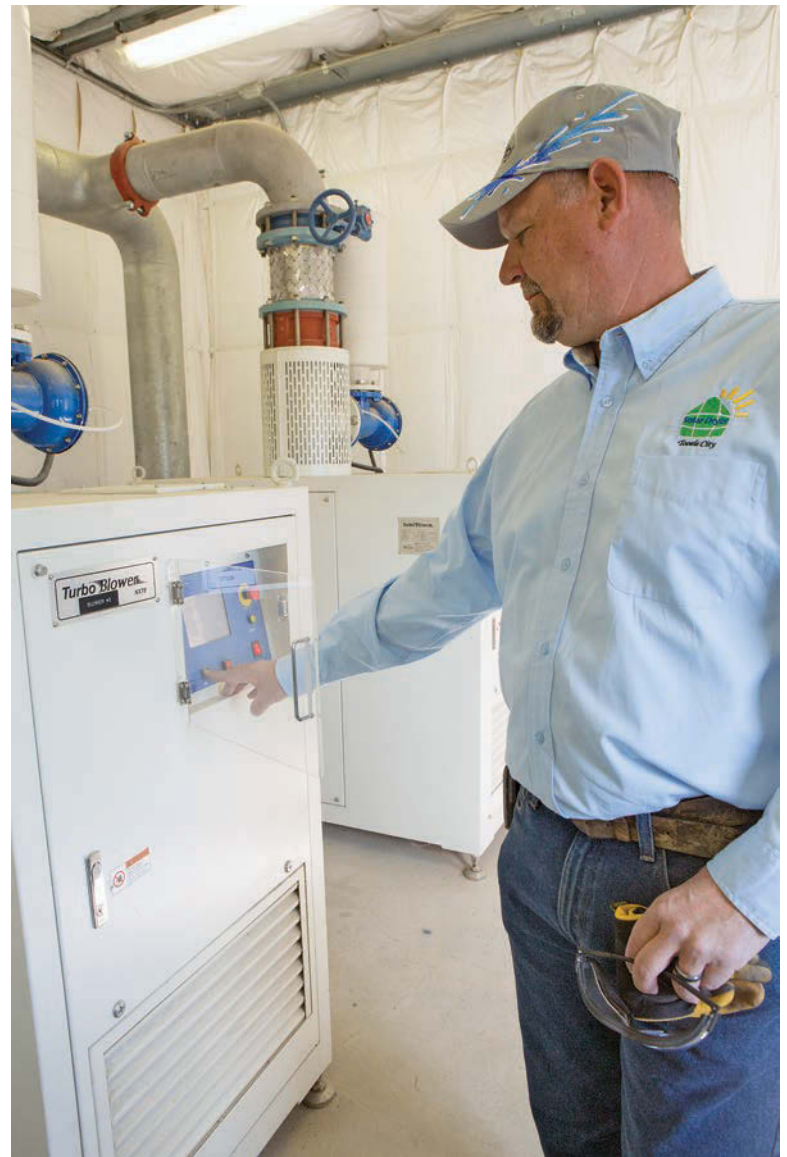
Scott Von Hatten checks one of the three 75 hp turbo blowers (APG-Neuros) that supply air to the plant's oxidation ditch (Kruger).
