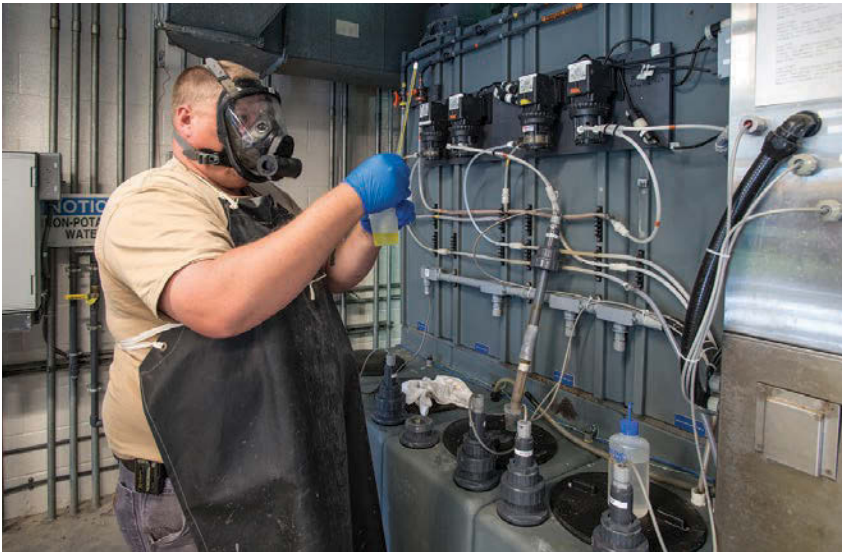
Jesse Wilkesman calibrates pH and ORP on wet chemical fowl air scrubbers at the control panel of the ATAD system (Evoqua Water Technologies).
