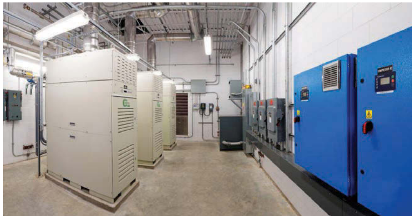
The combined heat and power system uses three 65 kW Capstone microturbines.
