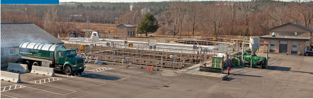
An overview of the Allenstown treatment plant. The small building on the right was the only plant addition needed to double capacity by way of the BioMag System.
