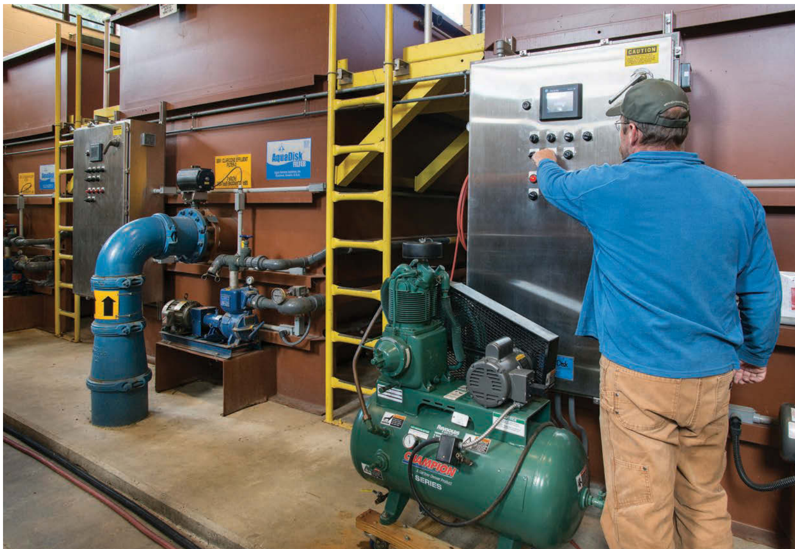
Mark Stirewalt adjusts control panels for the AquaDisk cloth media disc filters (Aqua-Aerobic Systems) in the UV/filter building. (Champion R-Series compressor from Gardner Denver.)
