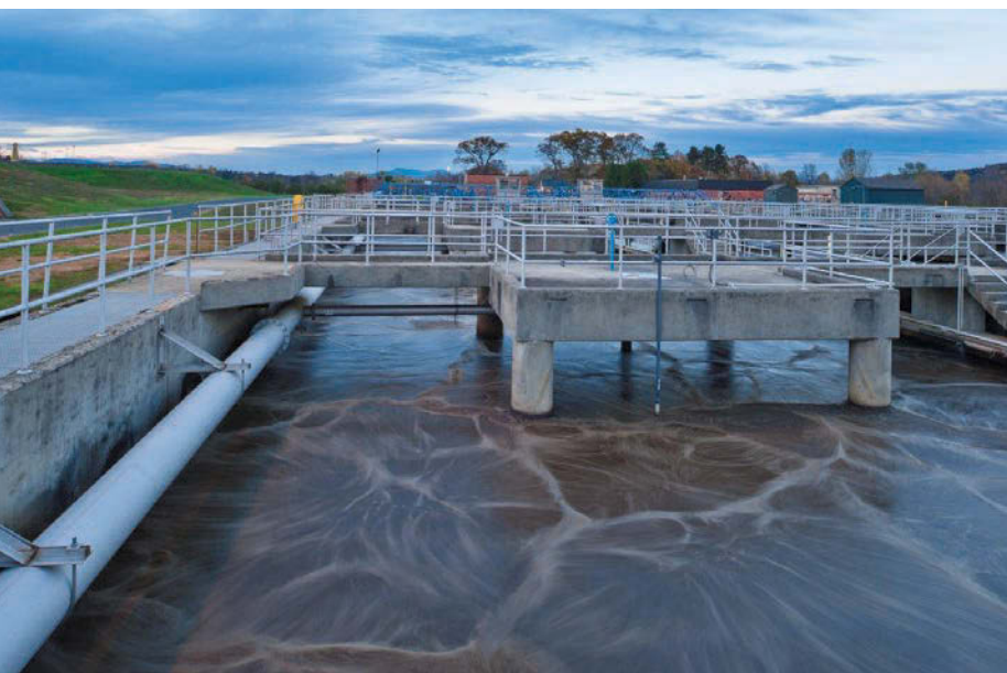
Aeration basins at the Pittsfield treatment facility now use 150 kW turbo blowers (HSI Blowers) and fine-bubble aeration (Sanitaire).
