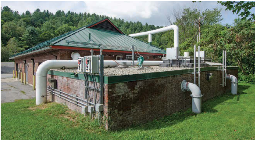
The ATAD process (tank and operations building shown here) uses heat released by microorganisms during digestion to kill pathogens.
