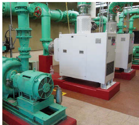
Two APG-Neuros turbo blowers (background) replaced two old centrifugal blowers to help cut energy consumption.
