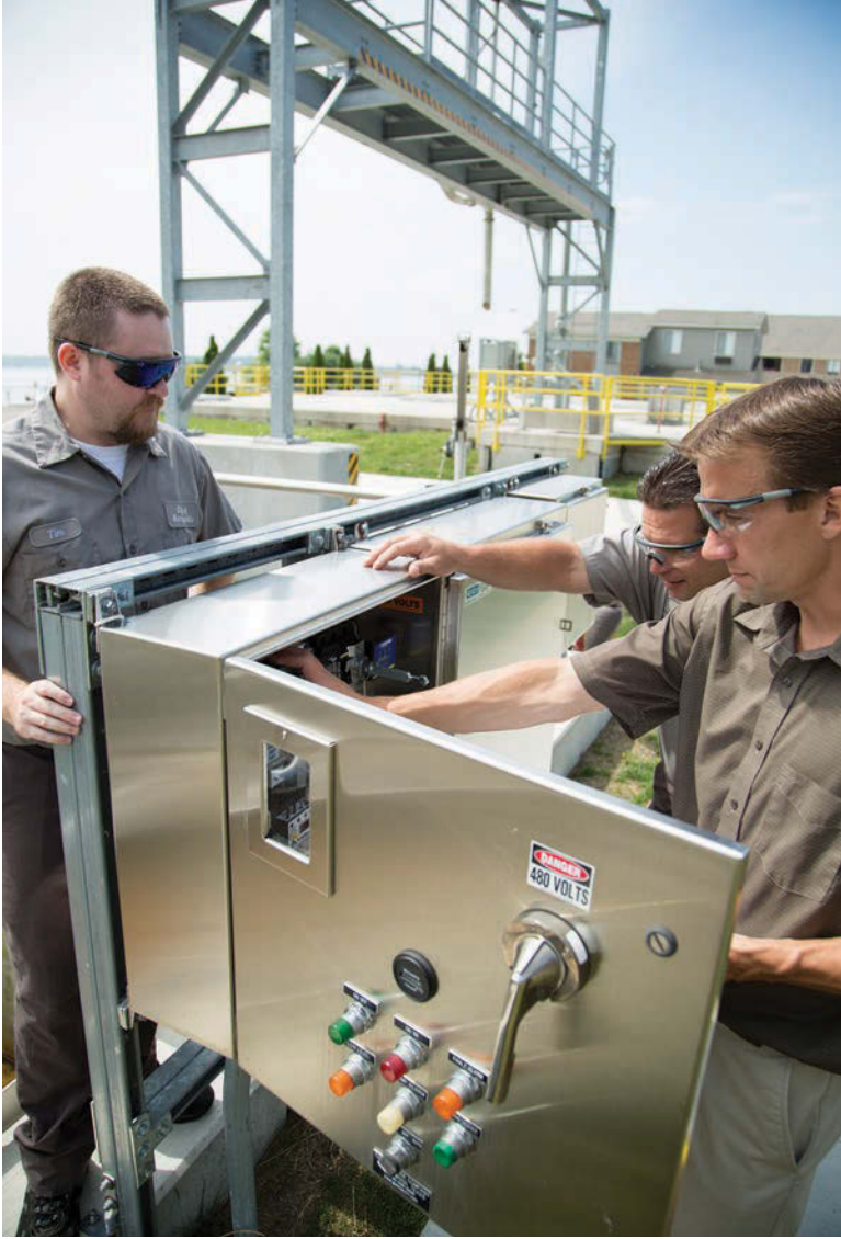
Bari Wrubel (right) inspects the chlorine diffuser panel with operators Tim Giles (left) and Jim Mieksztyn. The biosolids discharge trestle is above in the background.
