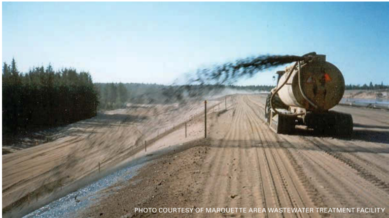
PHOTO COURTESY OF MARQUETTE AREA WASTEWATER TREATMENT FACILITY
