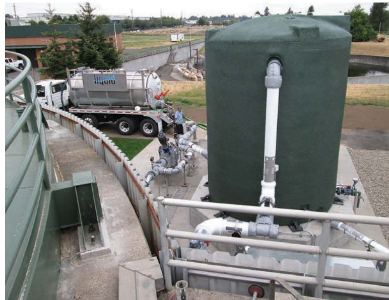
ABOVE: A hauler unloads at the Gresham FOG receiving station. Three haulers have contracted with the plant. RIGHT: Fine-bubble diffusers were installed in all aeration basins at the plant as one of several energy conservation projects.
