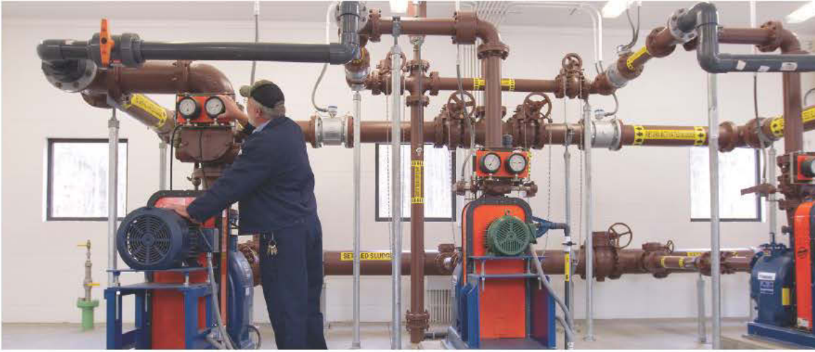
Keith Jackson examines a return activated sludge pump (Super T Series, Gorman-Rupp Co.).
