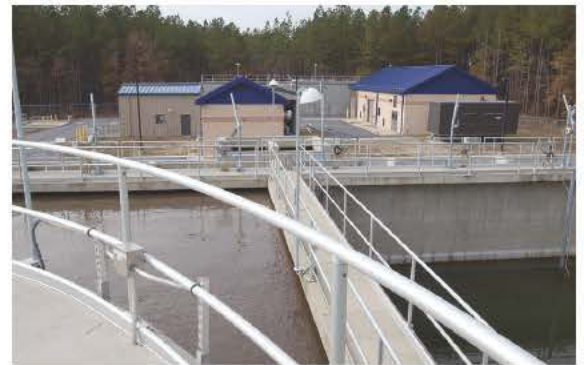
The previous facility was prone to overflows from I&I and high water in the receiving stream. The new facility includes oxidation ditches and new buildings that house a dewatering centrifuge and step screen.
