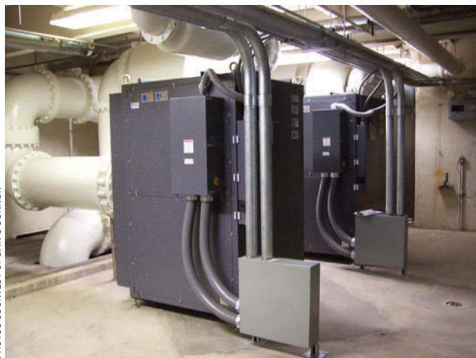
New K-Turbo (since purchased by Aerzen) blowers will save the New Ulm plant about $100,000 a year on electricity.
