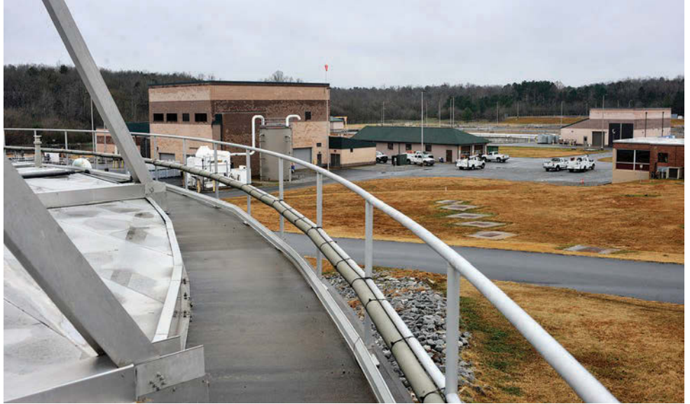
The Fairforest Wastewater Treatment Plant is one of eight water reclamation facilities operated by Spartanburg Water. (Photography by Michael Justus)
