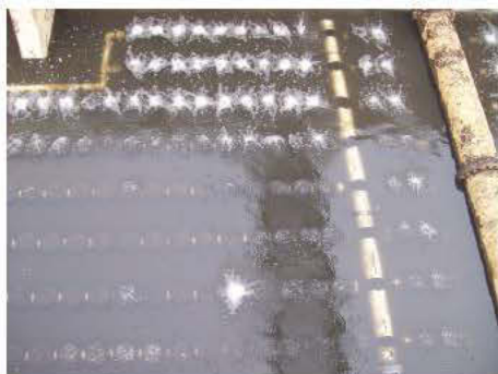
New diffusers are providing uniform oxygen dispersion throughout the aeration tanks and have eliminated dead spots.
