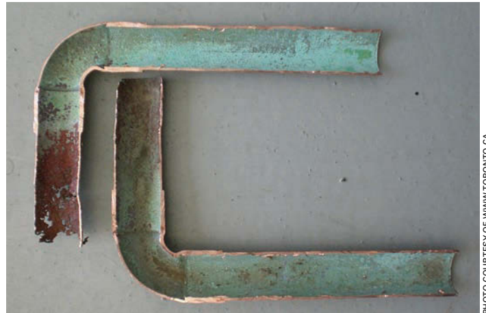
FIGURE 1: Interior of corroded copper pipe commonly used in older house plumbing.
