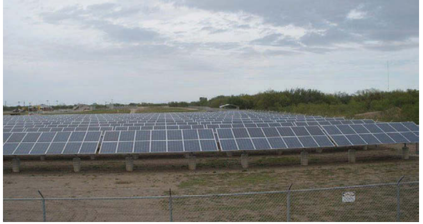
The City of Weslaco's South Wastewater Treatment Plant was chosen as the solar array site because it is highly visible to the public and demonstrates a commitment to efficiency and sustainability.
