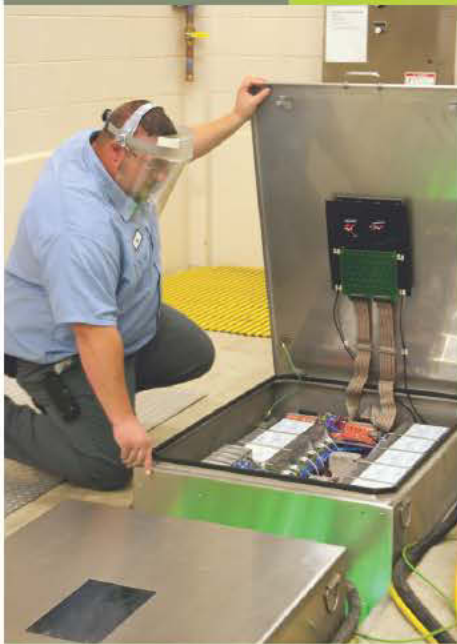
Tom Wood, operator II, checks the plant's UV disinfection system, supplied by Siemens Water Technologies. (Photography by Brian Masserman)
