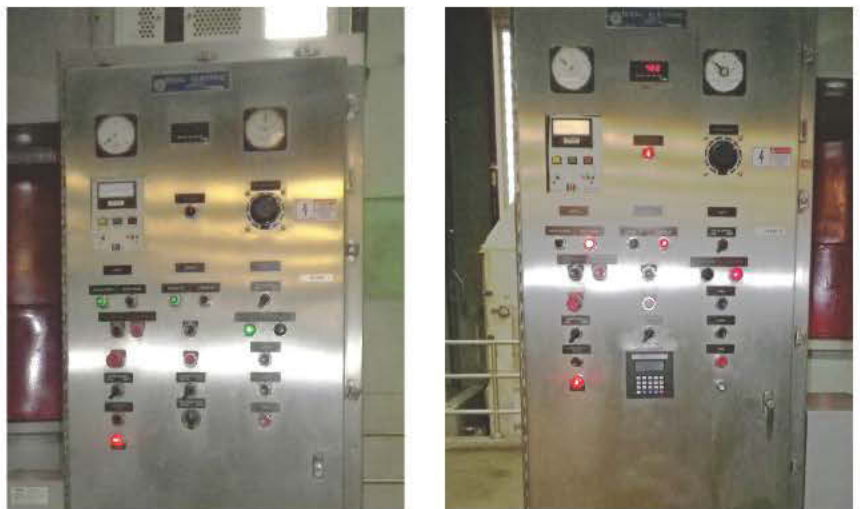
LEFT: The control panel for a 1,650 hp centrifugal Peerless pump before modification. RIGHT: Technicians added the Dynamatic keypad to the control panel and changed out the speed potentiometer, enabling operators to switch between automatic and manual modes.
