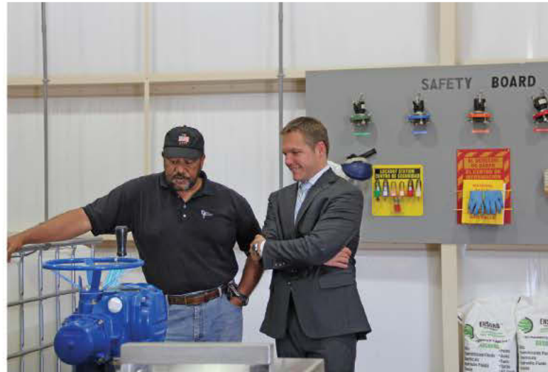
BCR Environmental CEO Aaron Zahn and vice-mayor Roy Tyler at the polymer control pump system at the Haines City Wastewater Treatment Plant.
