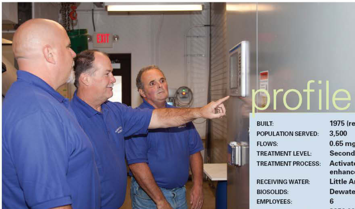
From left, operator Wayne Kennedy, chief operator Paul Lowe and operator Barry Lambert check the programmable logic control panel (Allen-Bradley/Rockwell Automation). (Photos by Stacey Damon)
