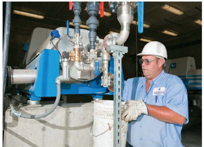
Warren Weber with the centrifuge (Andritz) at the Missouri plant.
