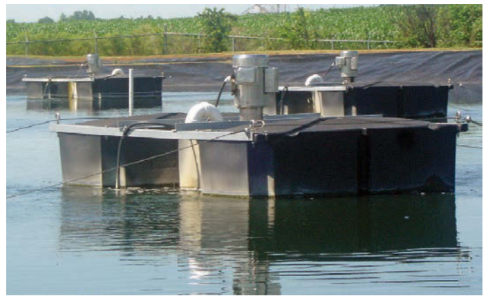
Floats on either side support the fusion aerator/mixers.
