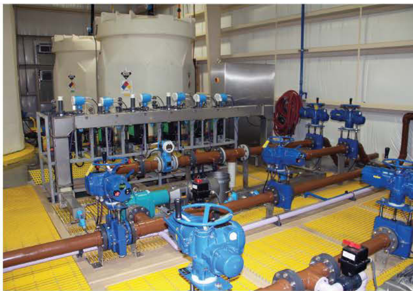
The chemical systems automatically inject a mixture of sulfuric acid, sodium chlorite, sodium hydroxide, ferric chloride and sodium nitrite in two processing steps.
