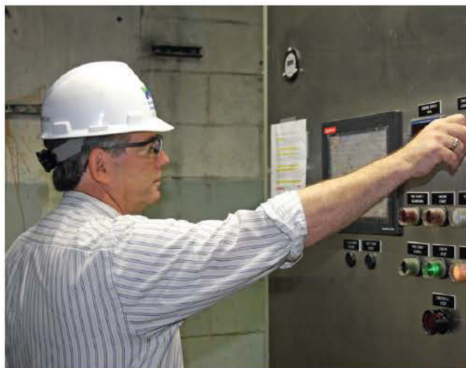
Plant superintendent Steve Askew checks the QuickPanel View engine pump control panel (GE Intelligent Platforms). (Photos by Sonny Maxon)
