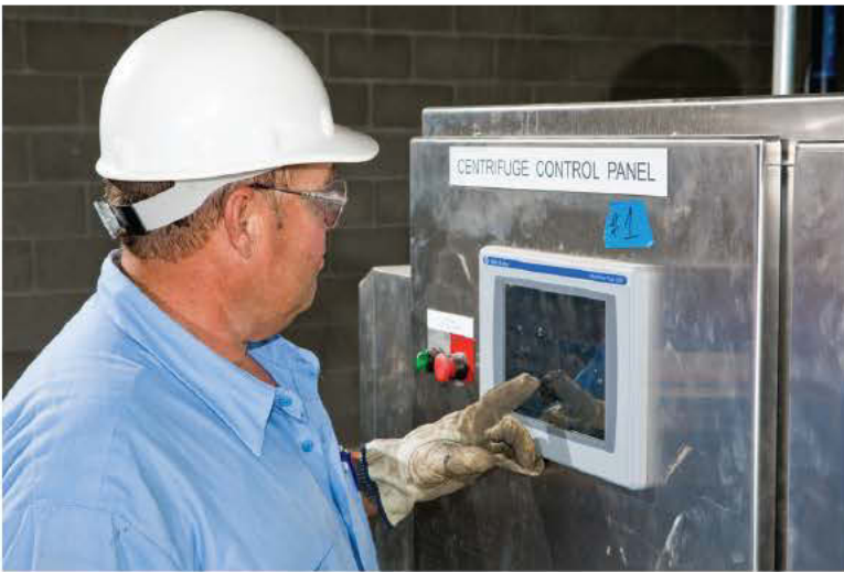
Operations residual coordinator Warren Weber checks the Allen-Bradley control panel (Rockwell Automation) of the centrifuge operation.
