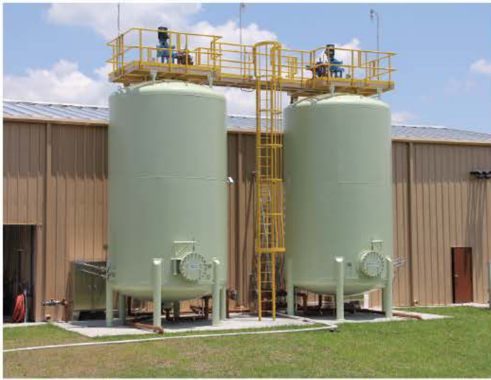
The Neutralizer batch processing tanks at the Haines City facility.
