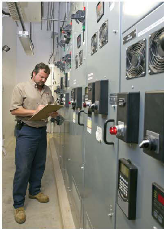
Project manager Roger Wilkes takes daily readings on the motor control center (Allen-Bradley/Rockwell Automation).
