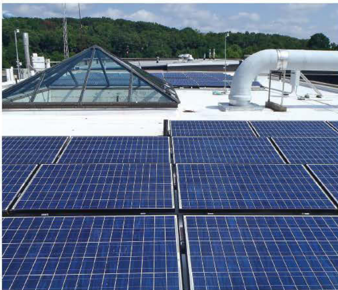
Two photovoltaic systems on building roofs are expected to save more than $3,000 a year in electricity costs.
