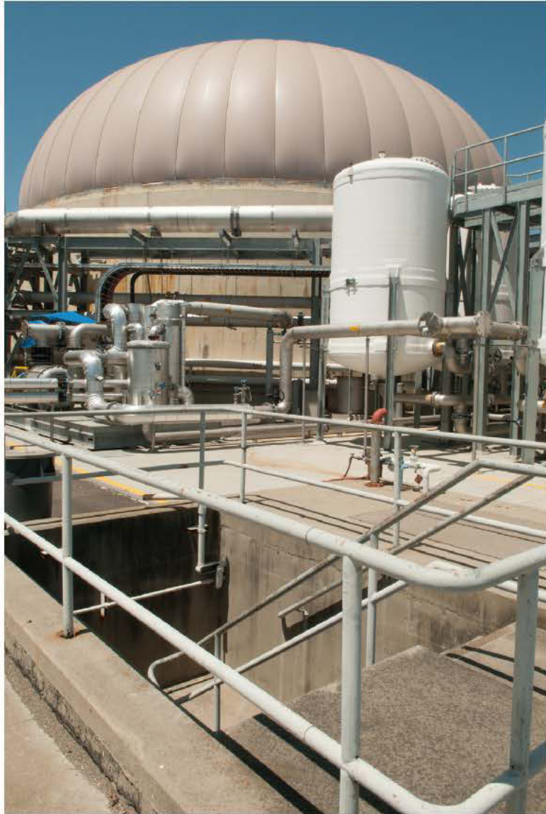
The EBMUD digesters use Dystor gas holding systems (Siemens Water Technologies).
