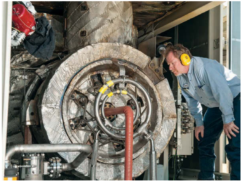
Neil Marvin checks one of the biogas-driven turbine generators (Solar Turbines) that convert biogas to electricity.
