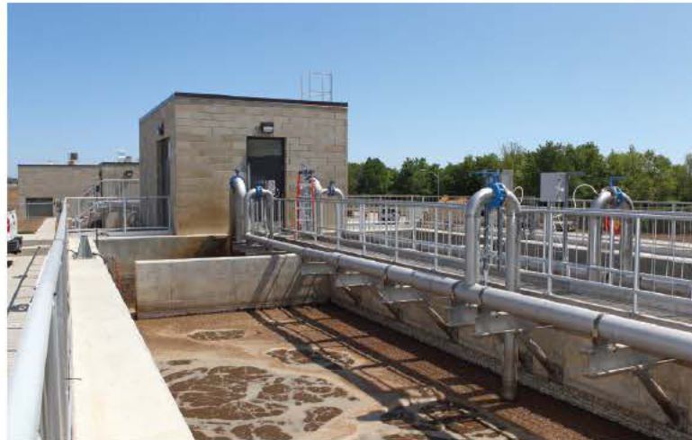
The aeration process at the Port Rowan plant has to handle tough wastes like septage and landfill leachate.
