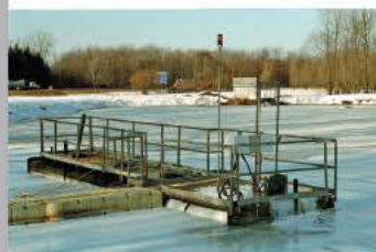
Floating BioReactor system from TVT-Bio
