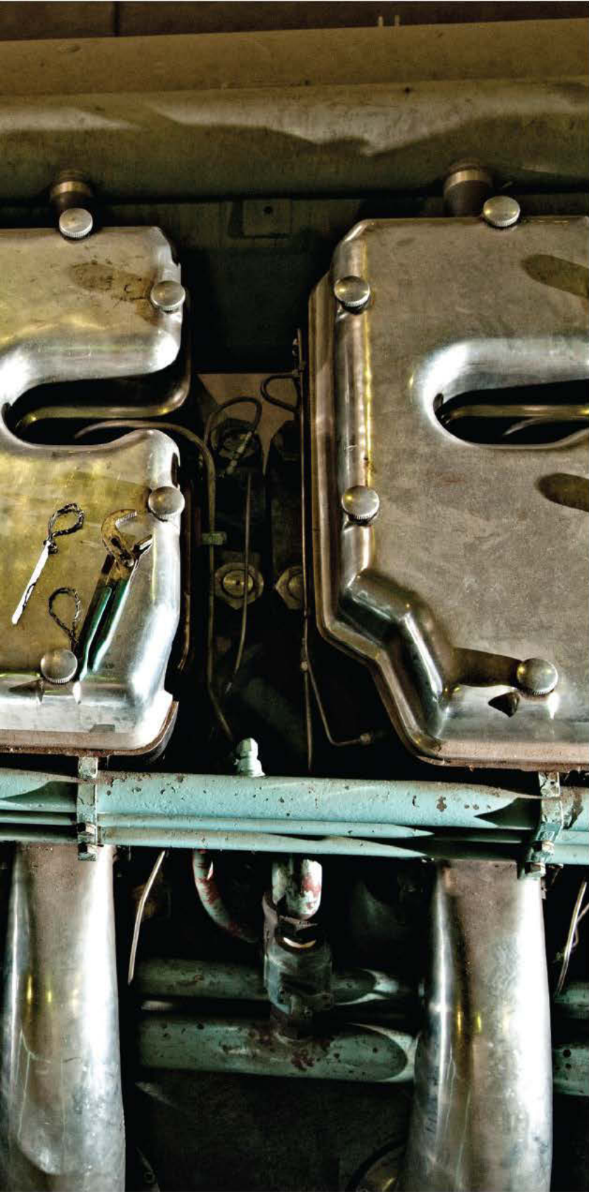
Power plant mechanic/operator Neil Marvin services one of four diesel engines at the East Bay Municipal Utility District wastewater treatment plant. (Photography by Keith Dixon)
