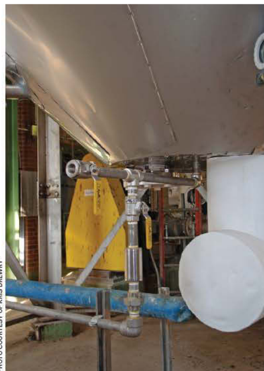
The air supply line to the Hydro-Pulse bubble-forming plate in the 10,000-gallon grease storage tank is easy to access.
