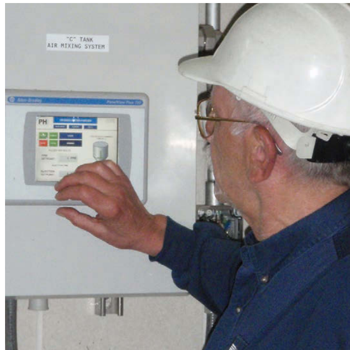
Shift supervisor Rich Bluemel at the Easterly Wastewater Treatment Plant adjusts the PHi mixing controller (Allen-Bradley PanelView Plus 700 terminal from Rockwell Automation).
