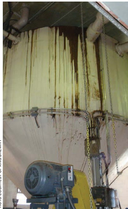
Overflows from the heated 10,000-gallon grease storage tank resembled liquid peanut butter but had the consistency of wax when cooled.
