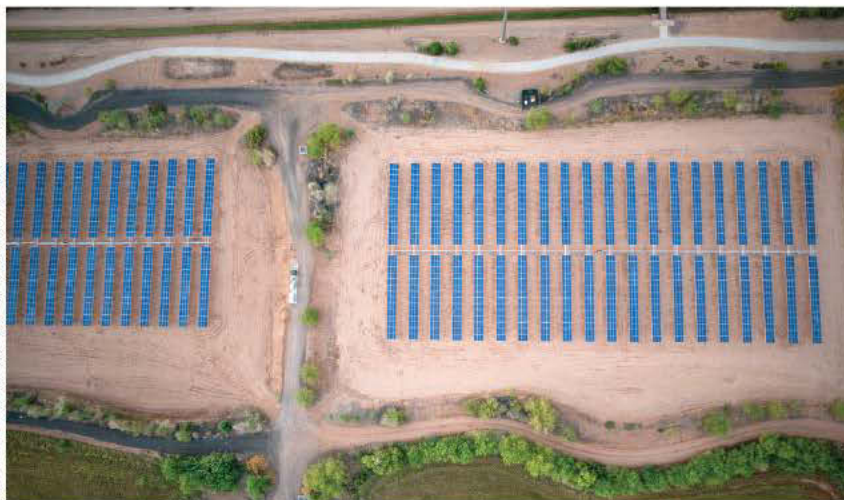
The 8,000 solar panels on the SPG Solar SunSeeker system at the Neely Wastewater Reclamation Plant are mounted on 6.5-foot-tall beams. The system will generate about 44 percent of the plant's electricity.
