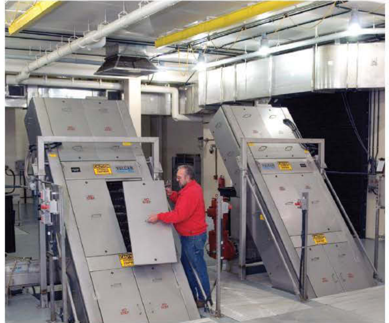
Maintenance mechanic Paul Marcus checks the fine step screens (Vulcan).
