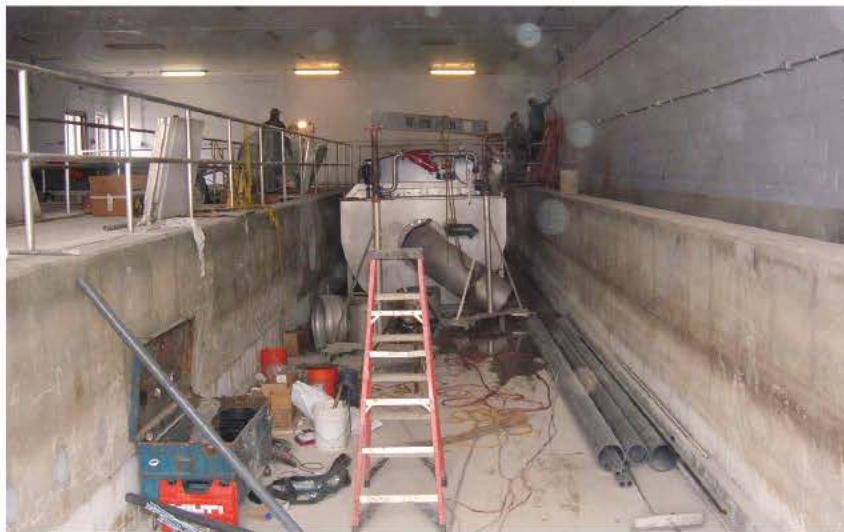
Workers from Manusos General Contracting in Fox Lake, Ill., install a SuperDisc filter assembly in Bay 2.
