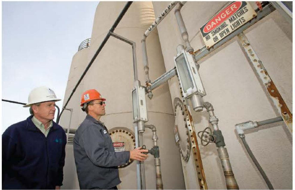
Wastewater Division manager Dan Thompson, left, and daily shift operator Bill Shaw control the oxygen flow in the anaerobic stage. (Photography by Jim Bryant)
