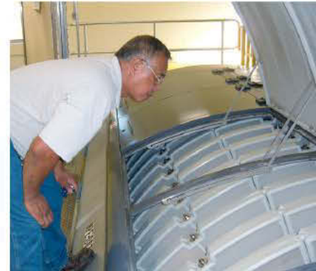
Lead operator Al Fajardo inspects the filter cartridges on a SuperDisc filter.
