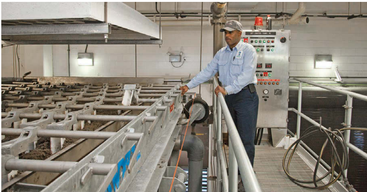
Operator III Warren Harris at the belt filter press (Andritz) in the dewatering facility.
