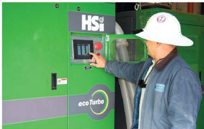
Grade 4 operator Jodey Lane checks the new high-efficiency blowers from HSI. Replacing the blowers earned the plant an $86,300 rebate from the local electric utility.
