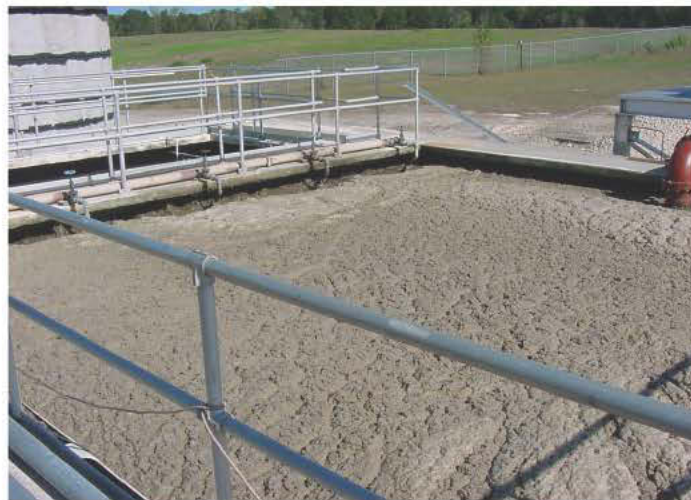
FIGURE 1 – Viscous foam formed a thick scum on the clarifiers, covering the entire surface and flowing into the scum boxes, which pumped to the aerobic digesters.
