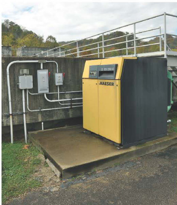
The Kaeser Com-paK Plus design features lower noise levels, more instrumentation, better maintenance access, and higher wire-to-air efficiency.
