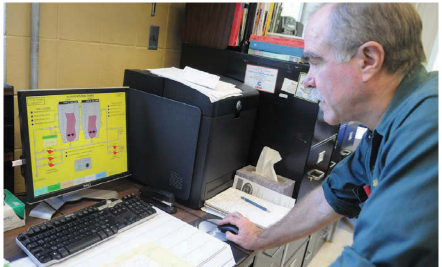
Robert Trombley checks data on the supervisory control and data acquisition (SCADA) system in the main office (GE iFIX).
