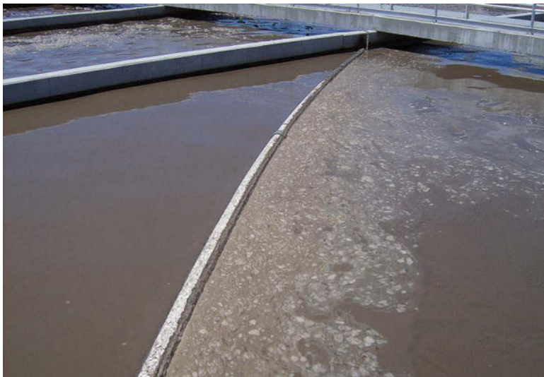
Figure 3 – A 4-inch PVC pipe, capped on both ends and supported by chains, floats on the oxidation ditch surface near the tank's outlet weir. This barrier corrals the foam to the weir, where the foam then flows into the clarifier.
