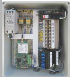
ScalableSCADA from Revere Control Systems
