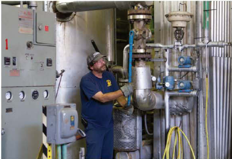
Operator Steve Dombek checks the Siemens-Zimpro PACT regeneration system. To the left is a control panel for a Vapor Power Modulatic steam generator. The tall, cylindrical tube is the reactor vessel and the rectangular structures on the right are the heat exchangers for the carbon regeneration process.
