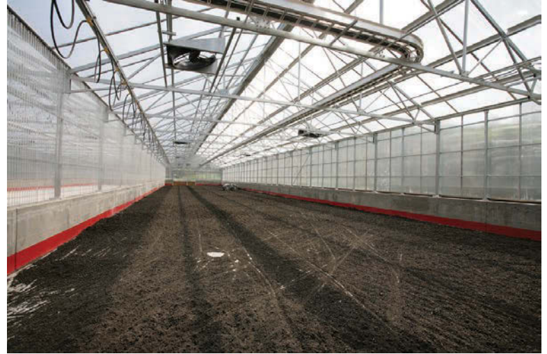
The Thermo-System active solar biosolids drying “greenhouses” from Parkson Corp.
