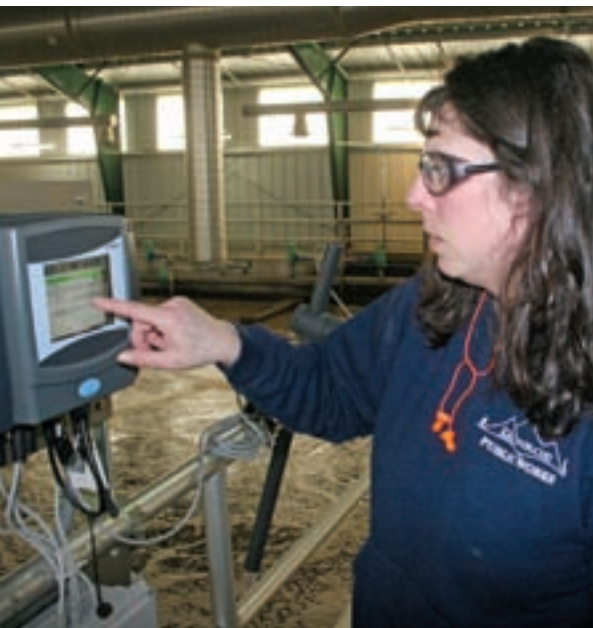
Theresa Davis calibrates the probes on the Hach sc1000 control unit. She stands over one of the aeration basins, which are indoors for odor control.
