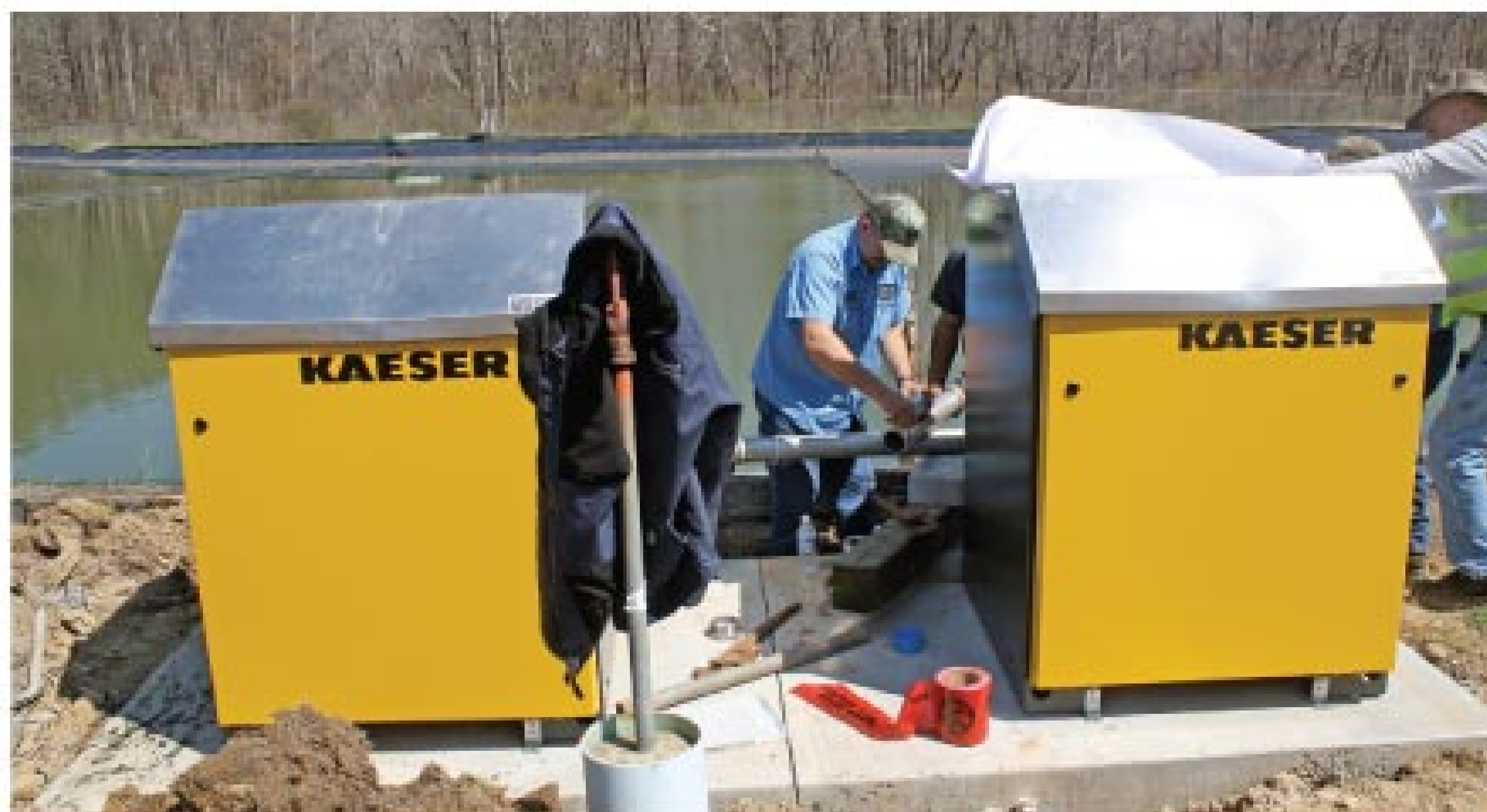
A city employee tightens the stainless steel header connecting the Kaeser blowers to the aeration units.
