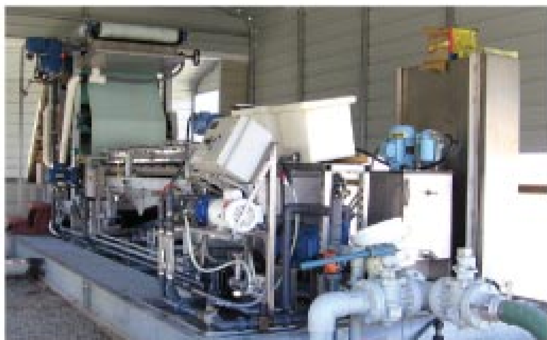
Skid Mounted System Thunder Bay Casino Sacramento, CA Tel: 209-483-4118
