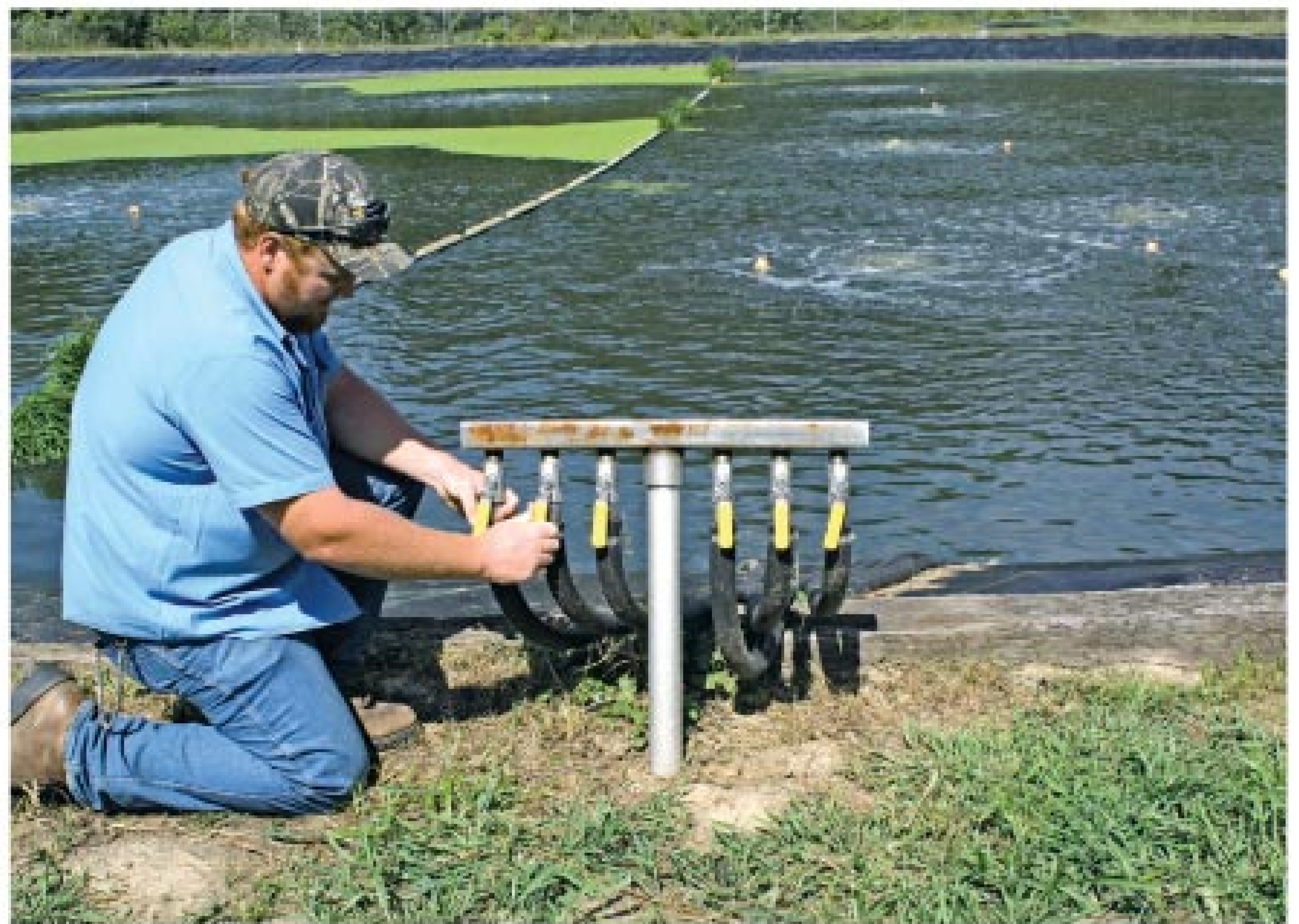
A city employee controls the airflow to each MARS unit in cell one by way of a stainless steel ball valve connected to a stainless steel air manifold.
