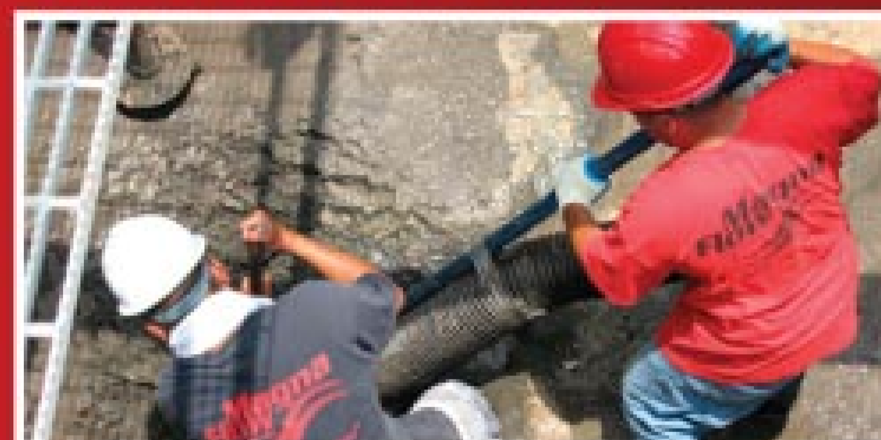
Total Plant Cleanouts
