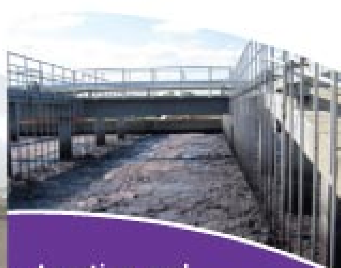
Aeration and Aerobic Digestion Systems
