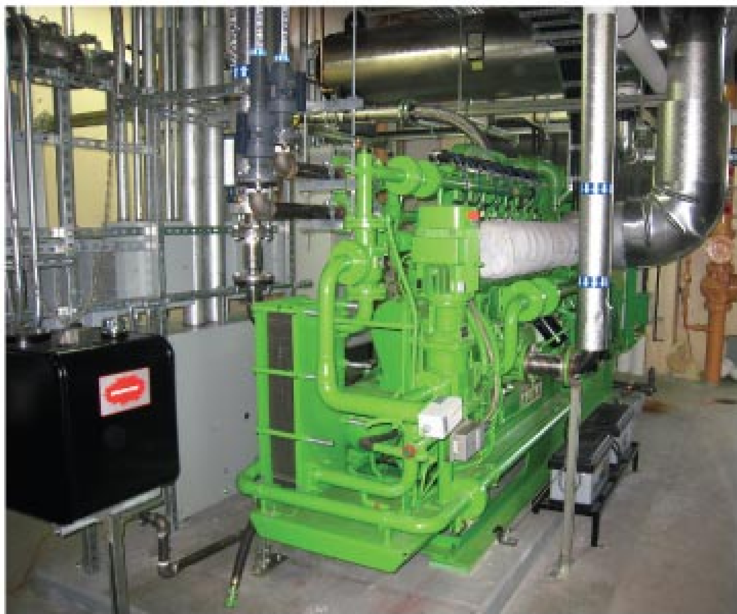
This GE Jenbacher reciprocating engine provides power and heated water for the Budd Inlet Water Treatment Plant, the LOTT Regional Services Building, and the new Hands On Children's Museum across the street.
