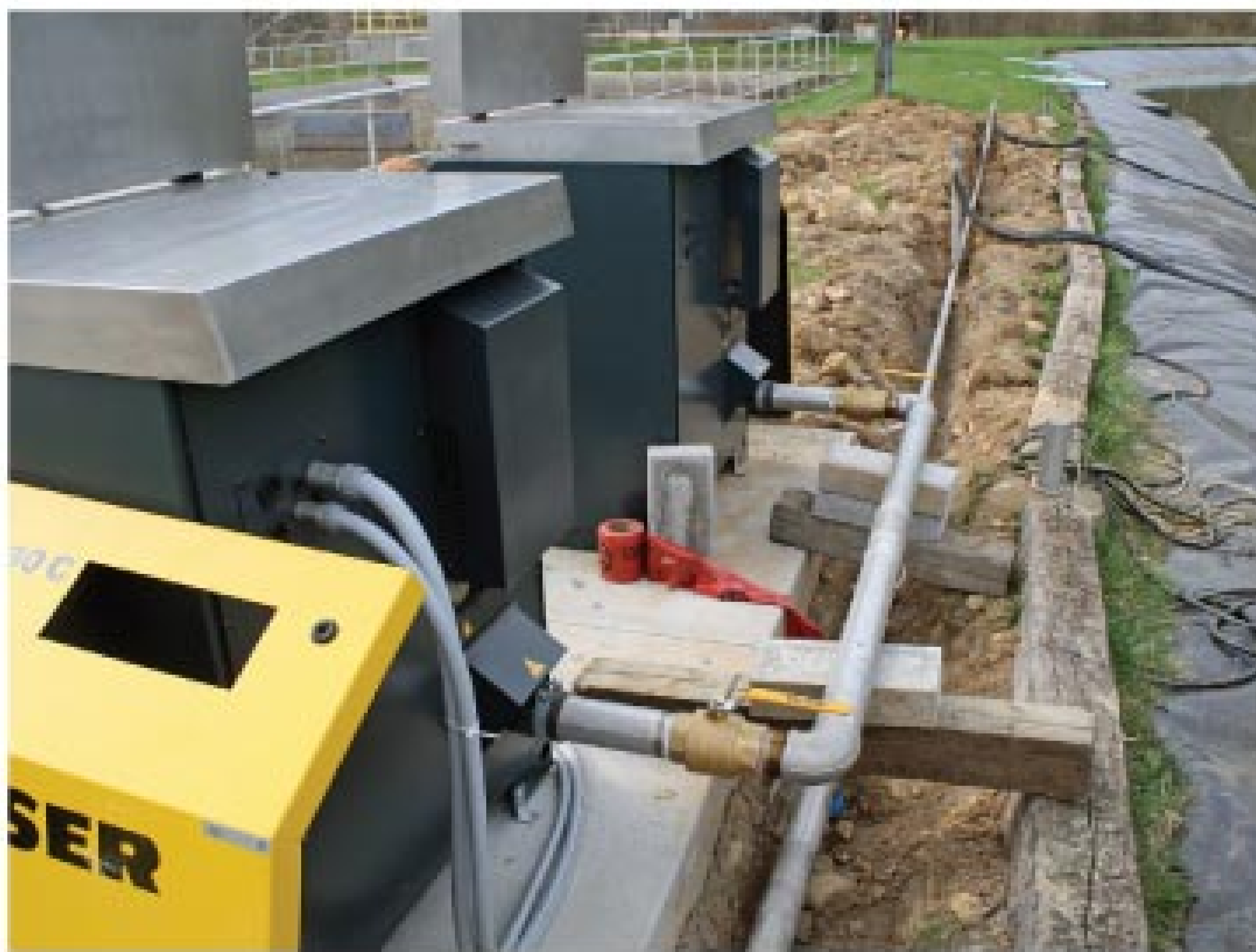
Two Kaeser CB 130C blowers and their header are tested for leaks before backfilling of the trench.
