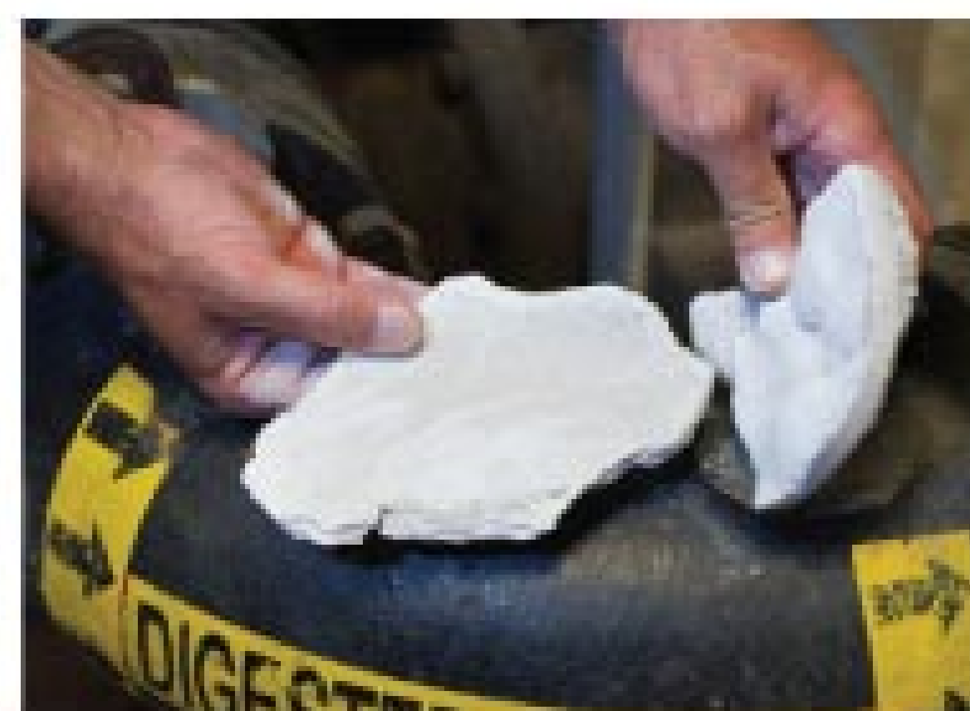
A sample of struvite (magnesium ammonium hydroxide) removed from piping in the treatment plant.
