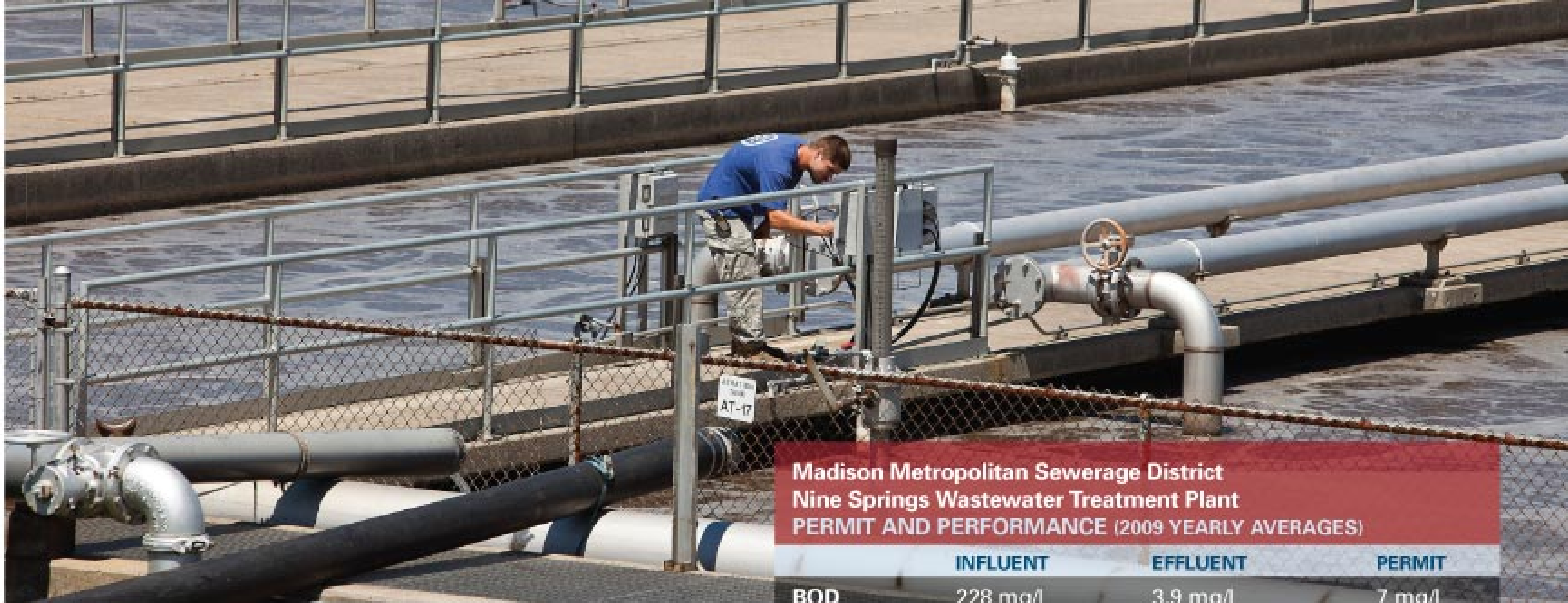
Nathaniel Heiden, relief operator, inspects equipment used to test dynamic wet pressure on the aeration diffusers.
