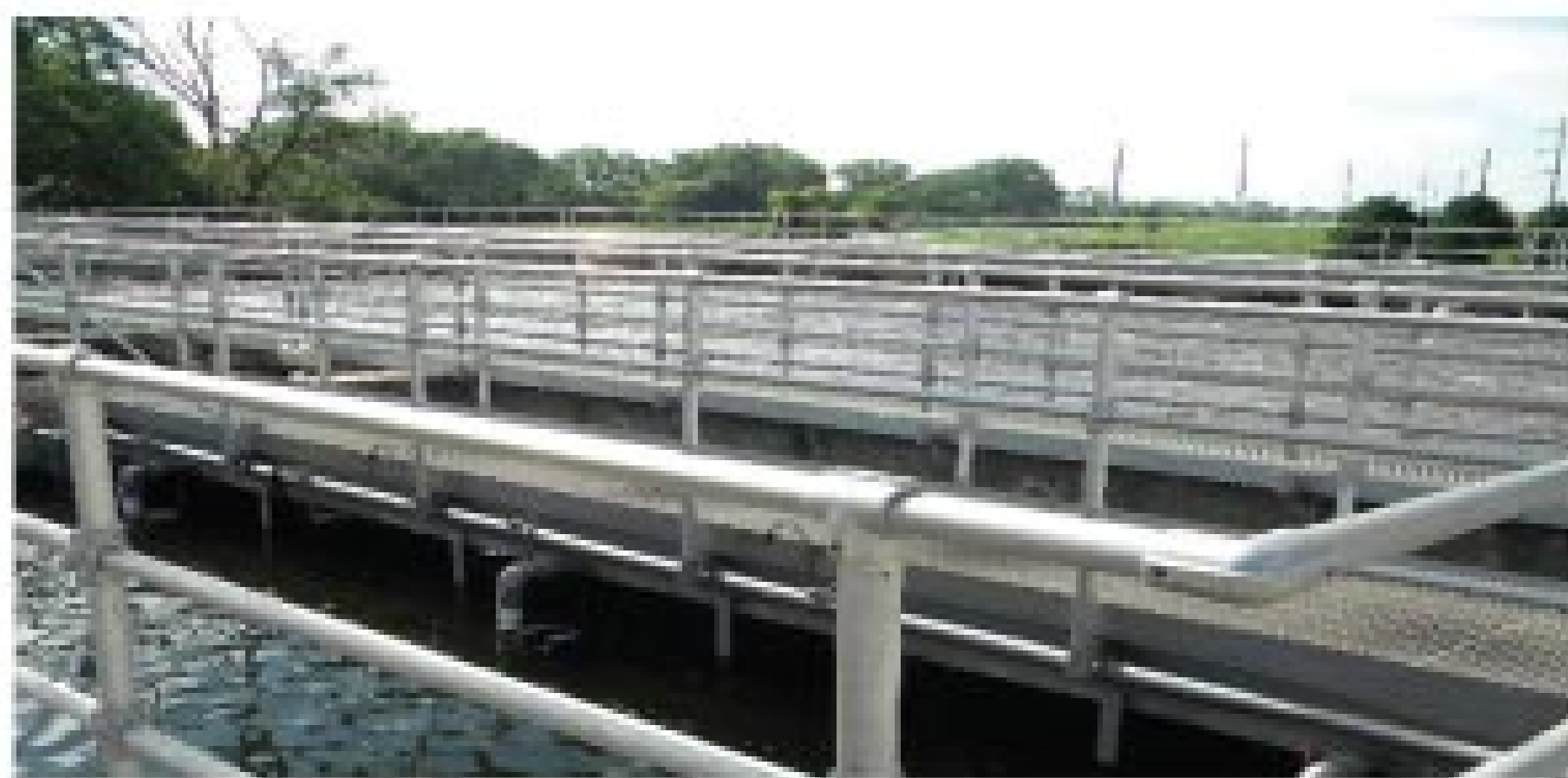
The City of Maize treatment plant, a 0.5 mgd extended aeration activated sludge facility, accommodates the ethanol plant process water without upsets.
