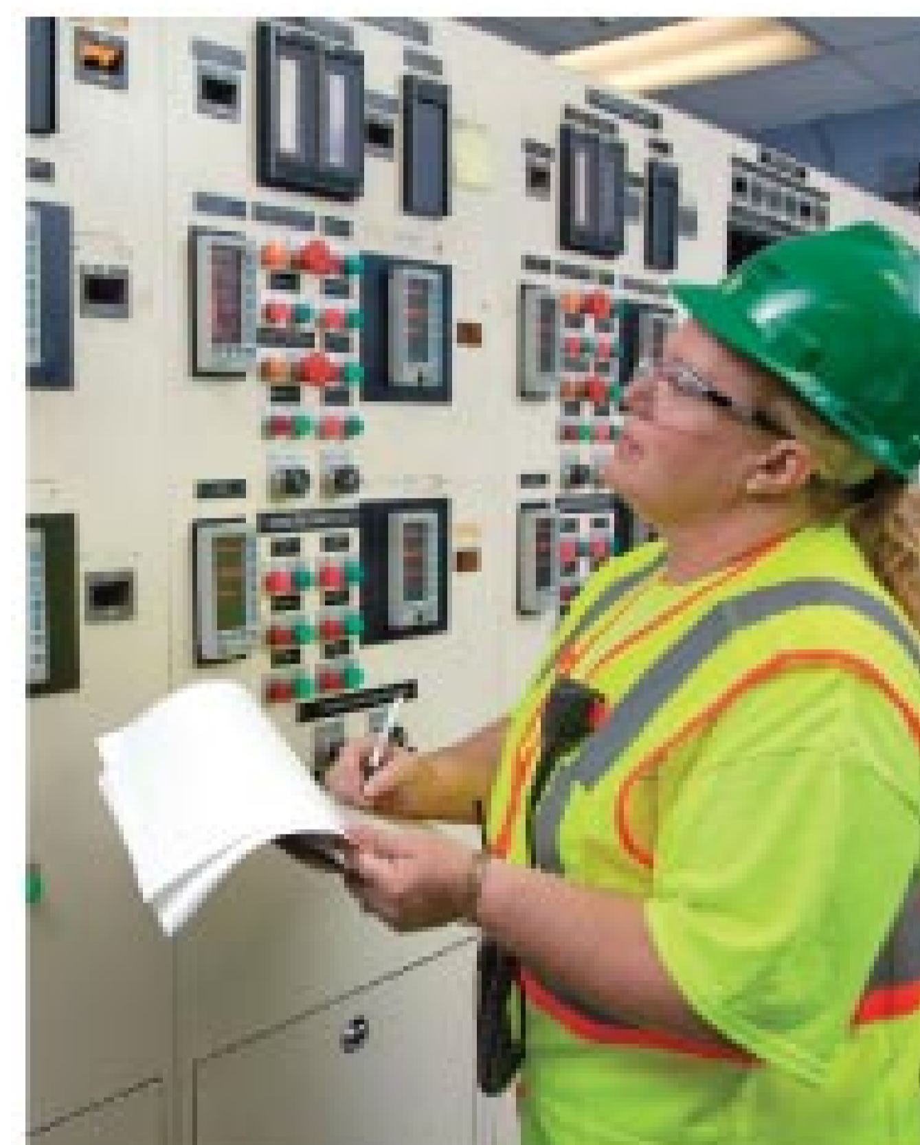
Dewatering operator Dana Vollmerhausen monitors the control panel.
