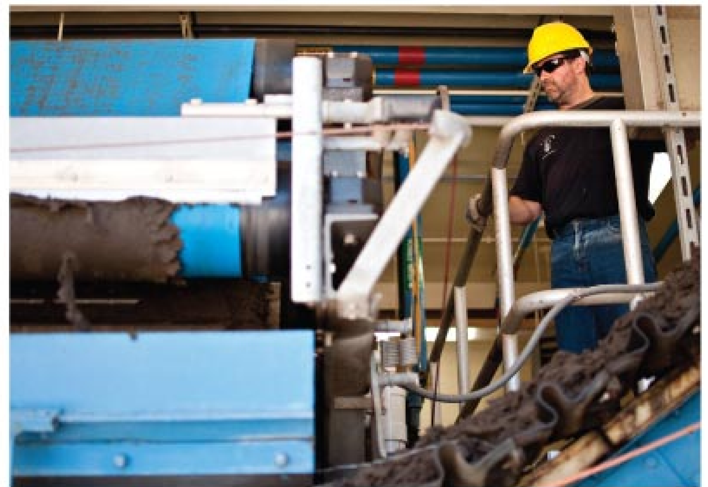
Wastewater operator Randall Frake adjusts the sludge feed on an Ashbrook belt filter press.
