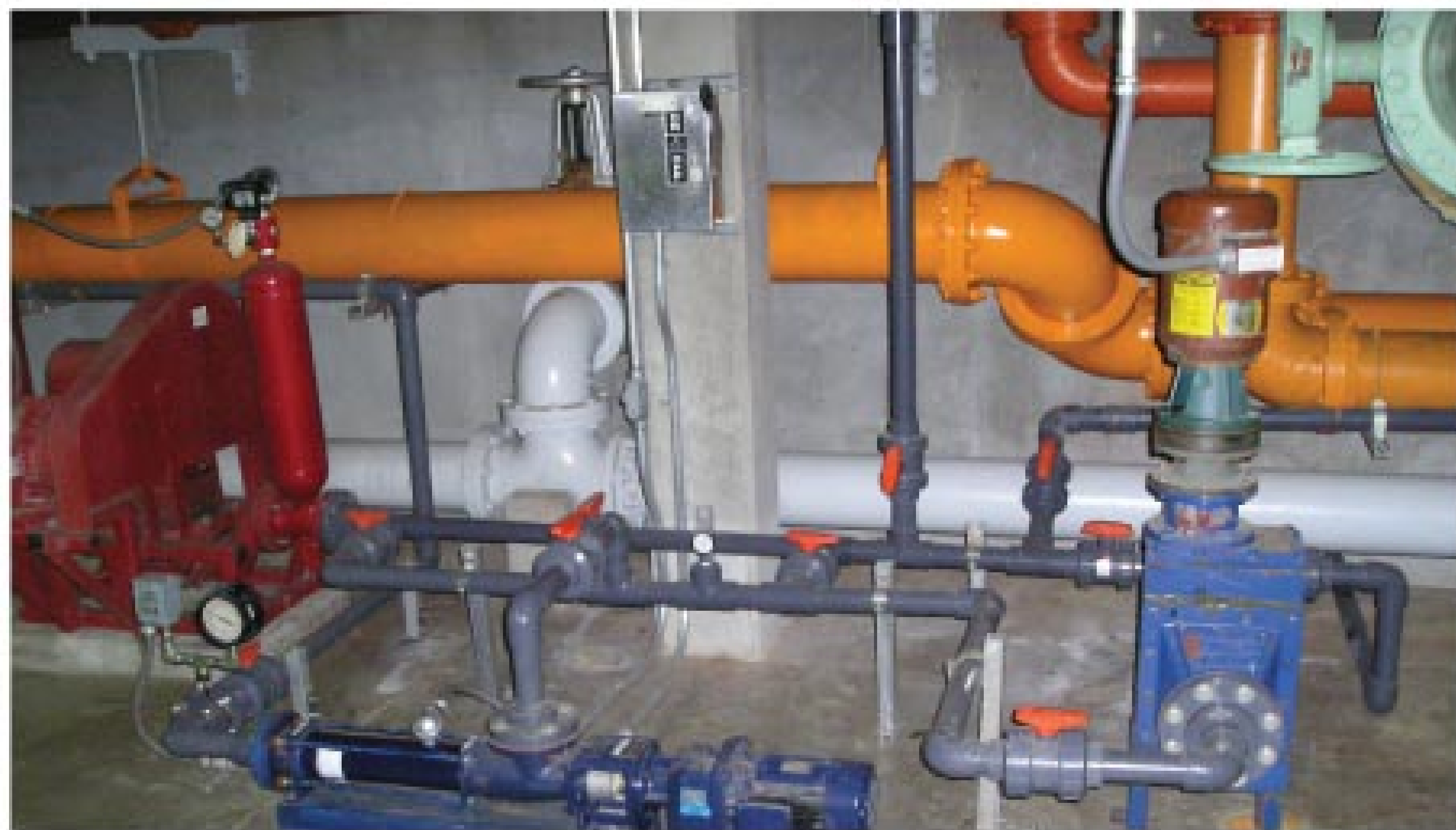
The ChemScan pump and grinder at the West Hickman Creek Wastewater Treatment Plant.
