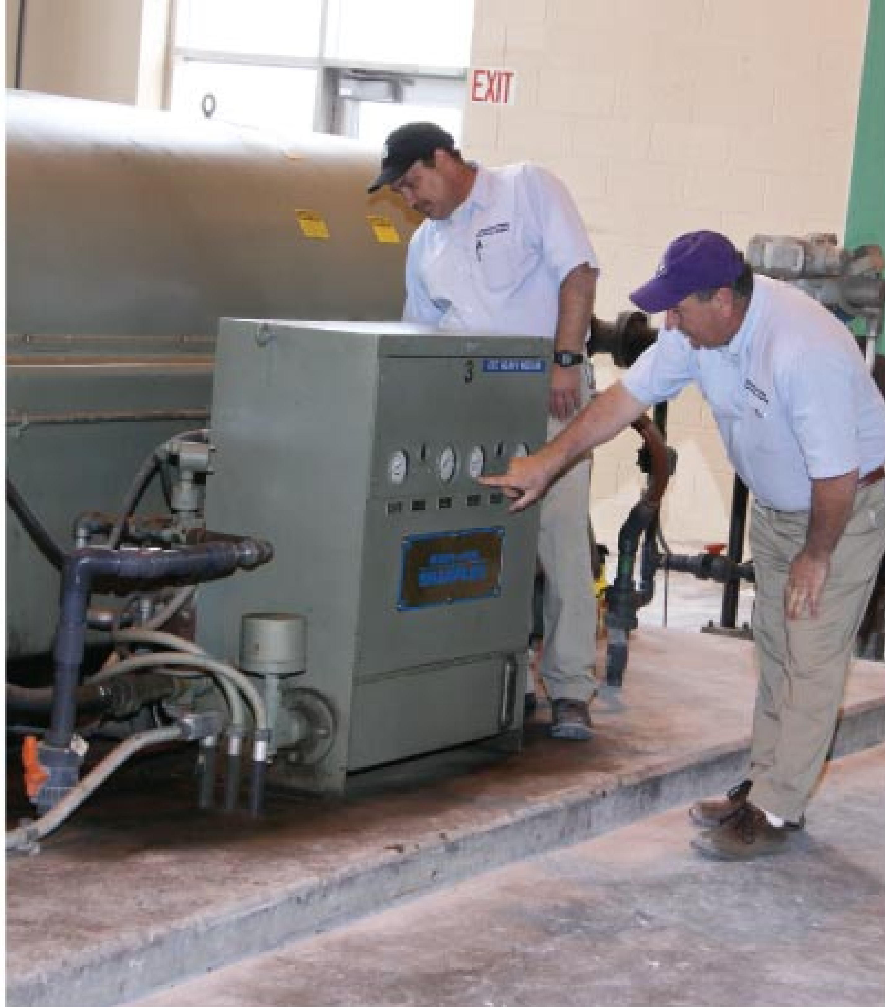
Chuck Zambito, maintenance supervisor (left) and Joe Hines, electrical supervisor, discuss the operating pressure of the Sharples (Alfa Laval) centrifuge.
