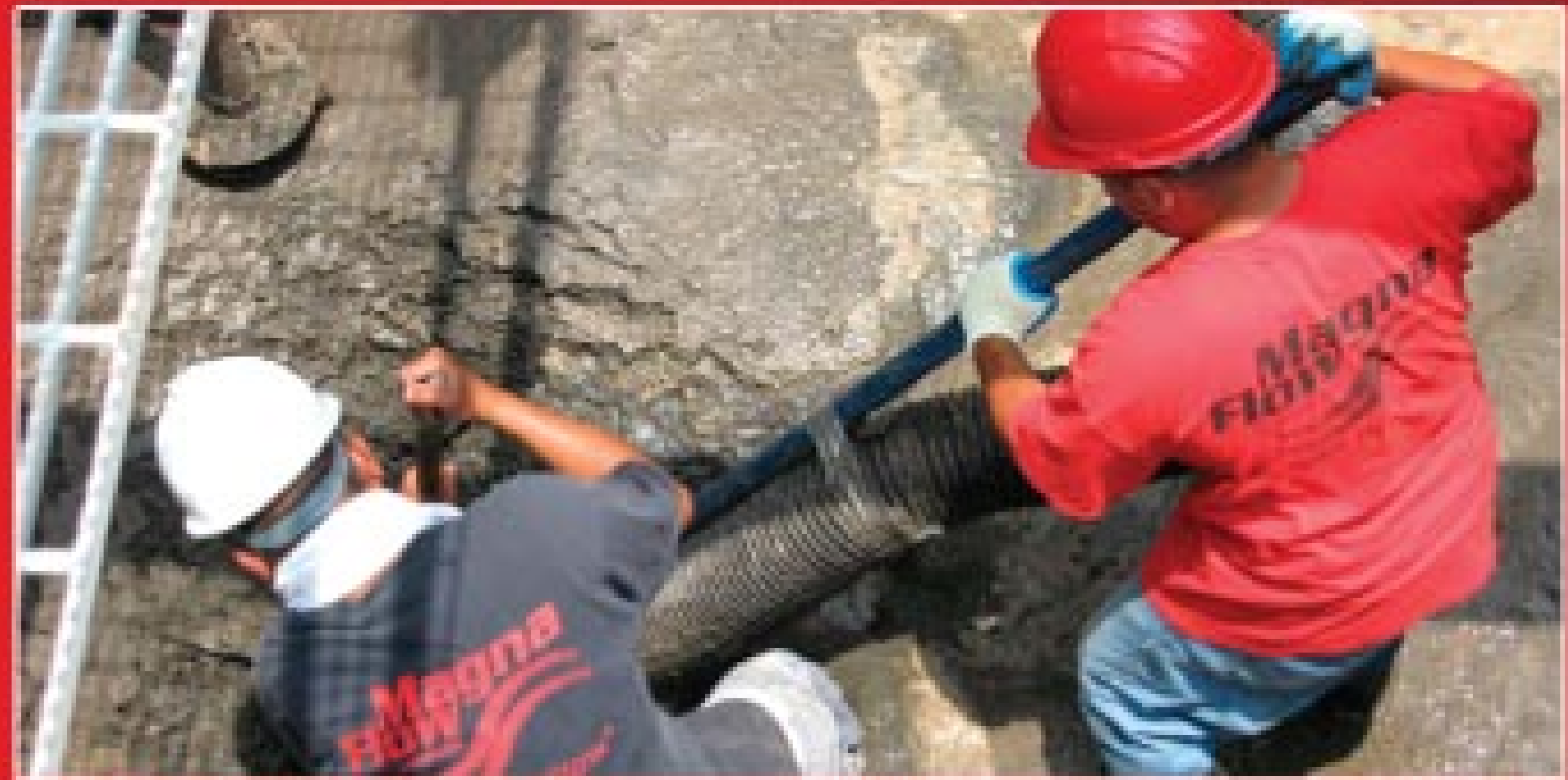
Total Plant Cleanouts
