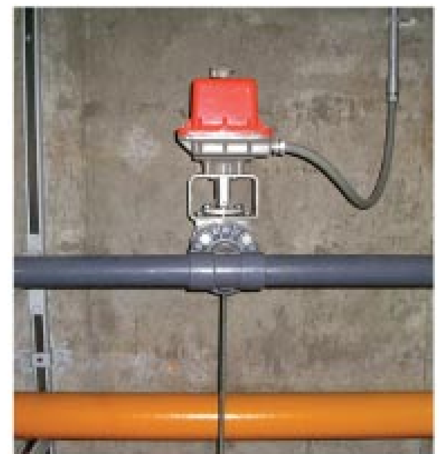
Each sampling point in the ChemScan system has a Bettis electric valve from Emerson Process Management Valve Automation.
