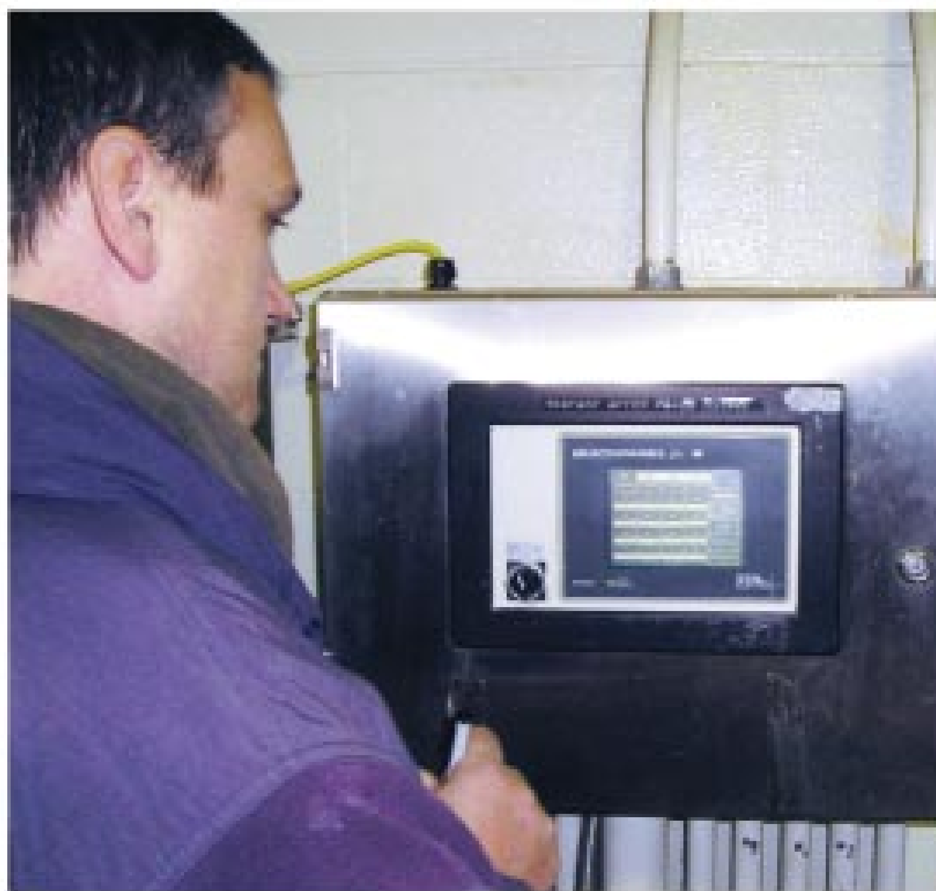
Plant operator David Adamovich records readings from the ChemScan system.
