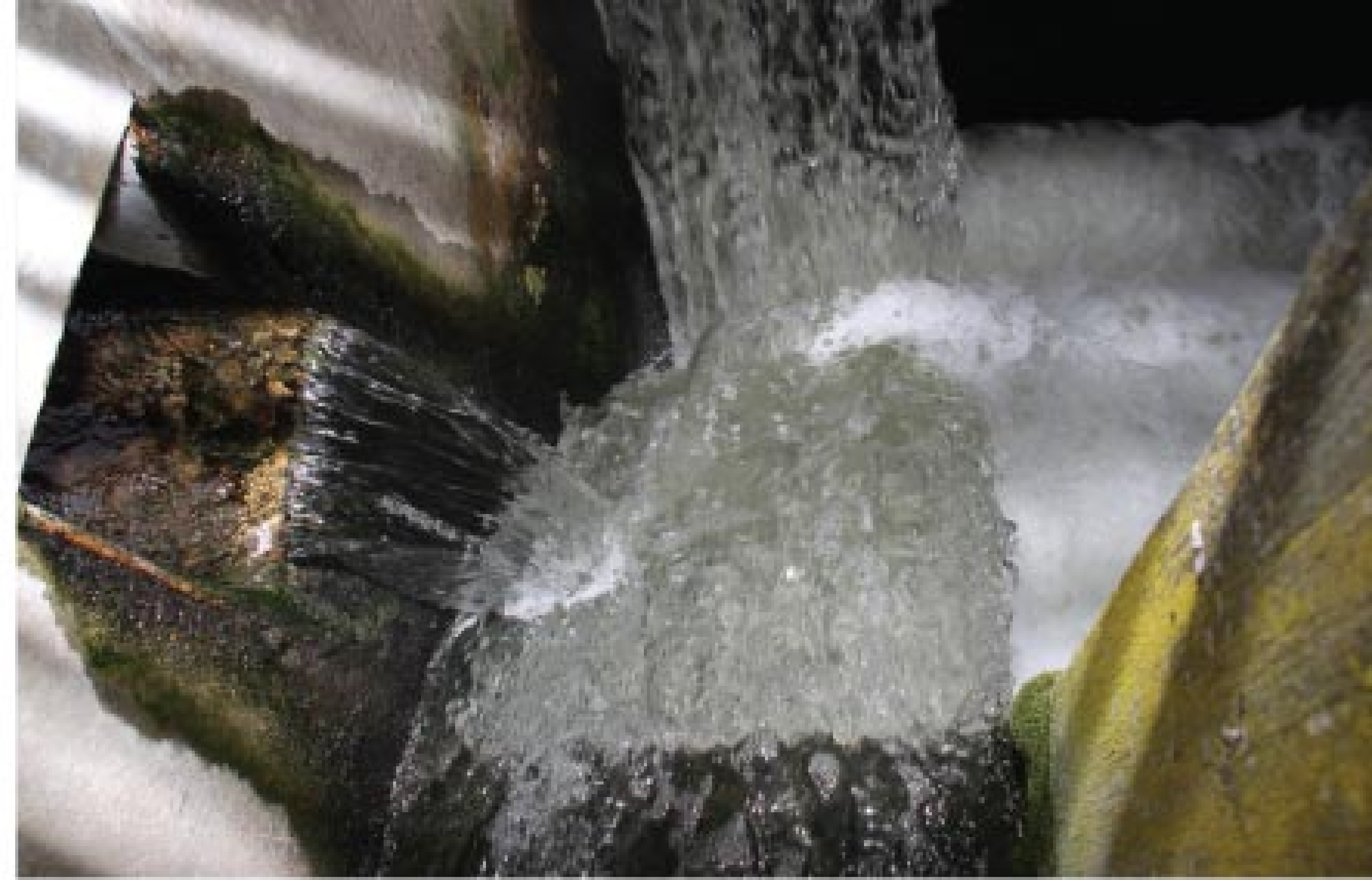
Water leaves the final clarifier at the Wyoming Valley treatment plant.
