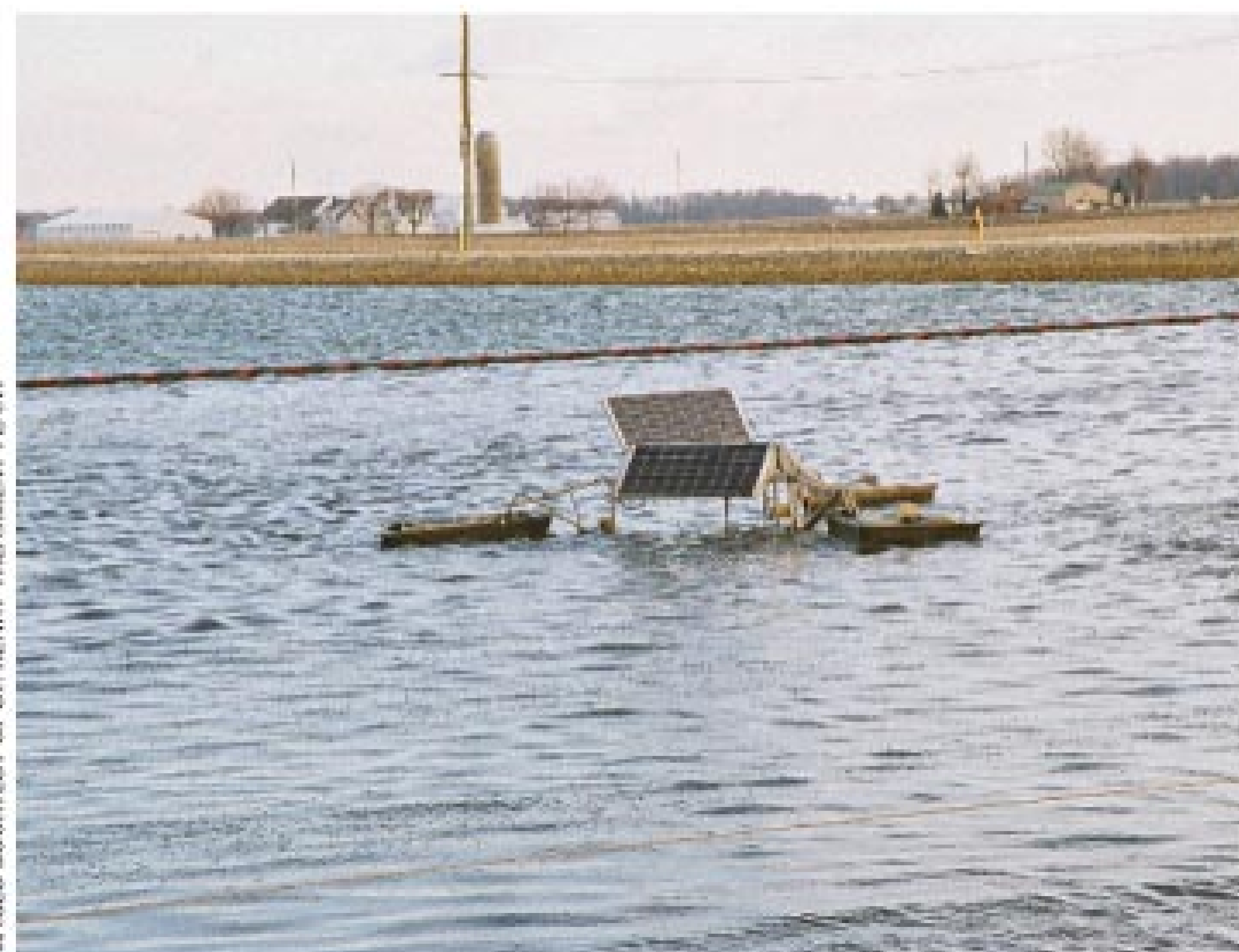
IMAGES COURTESY OF ST. HENRY TREATMENT PLANT
