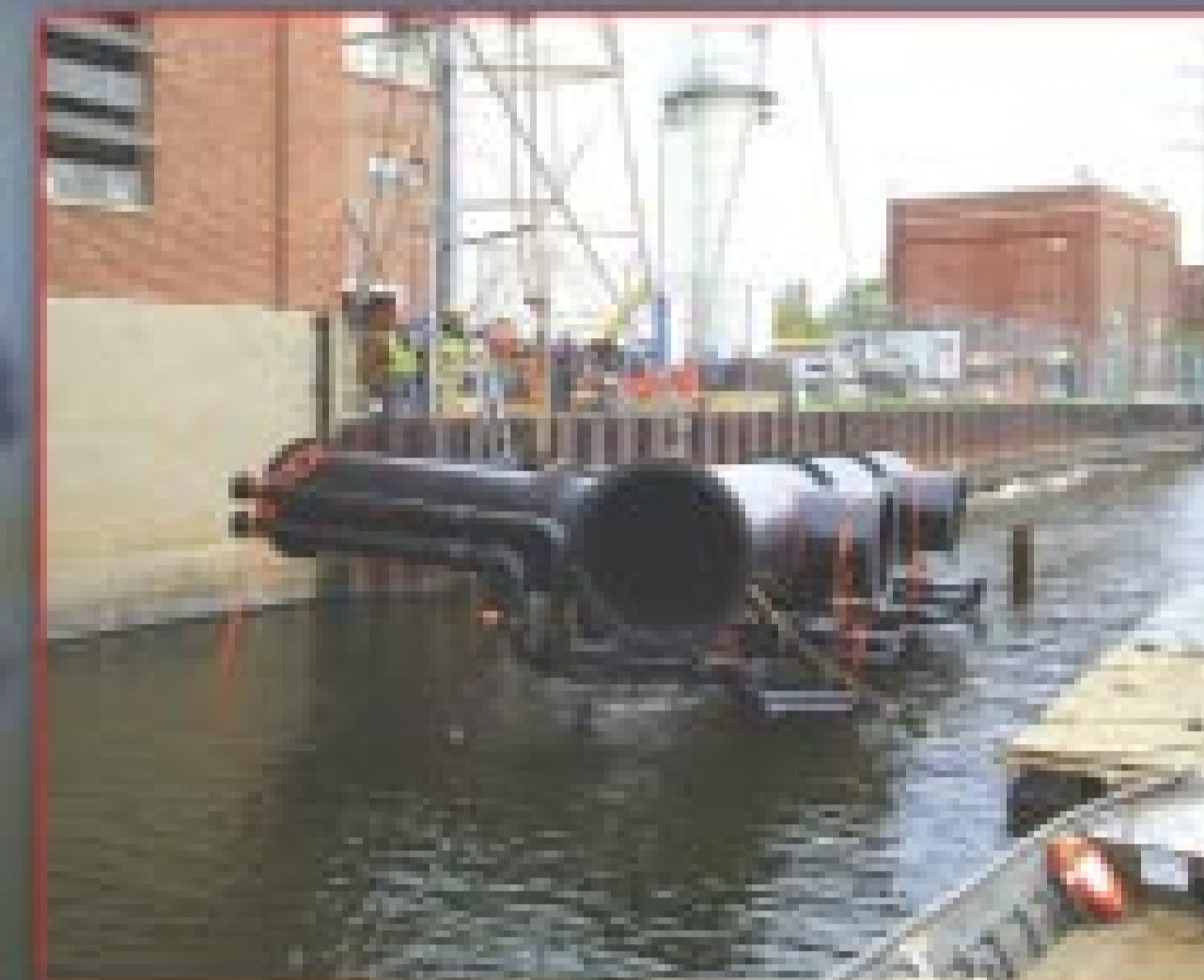
Intake Circulating Water Pipe - Xcel Energy, MN
