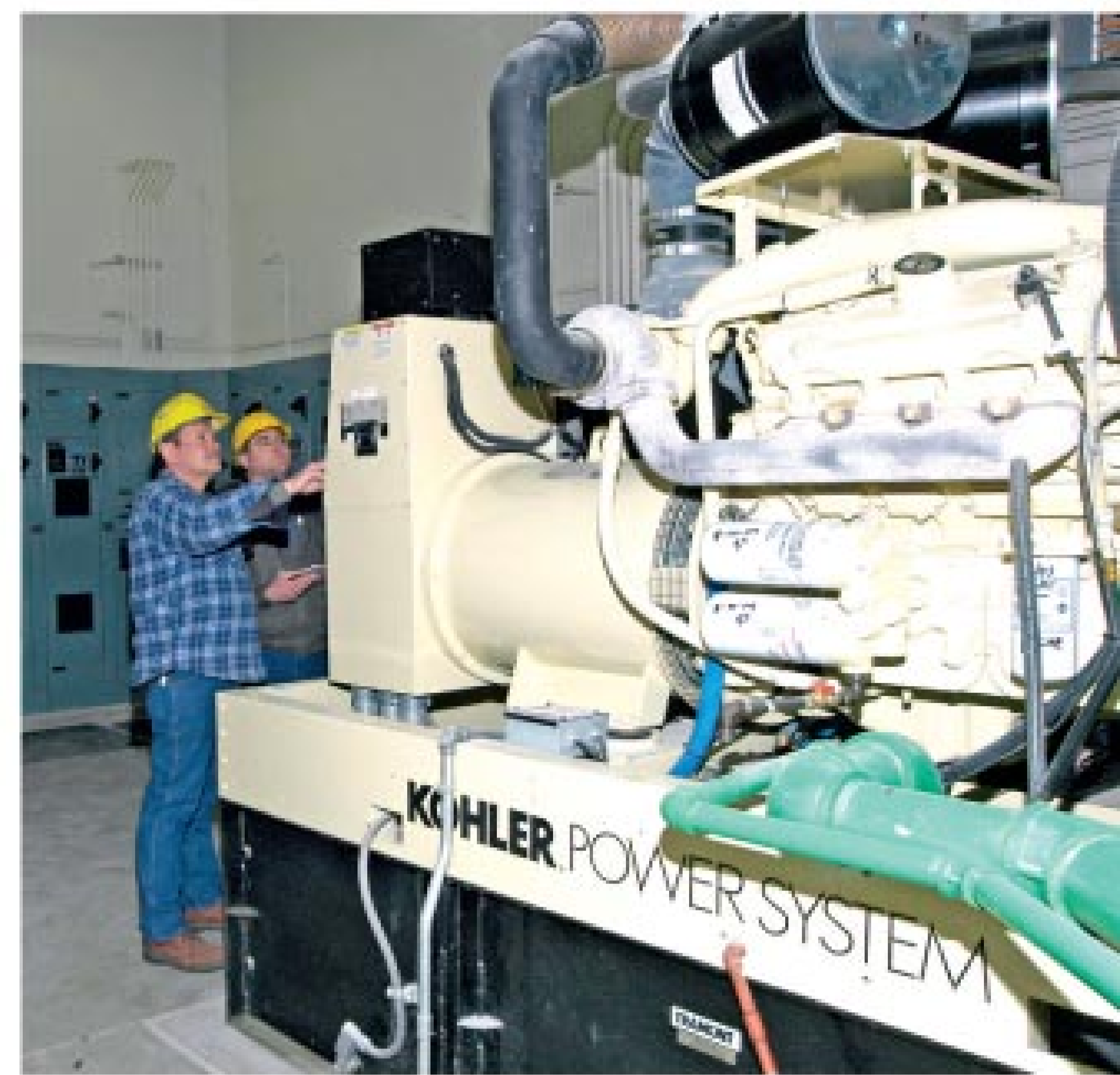
Operators Mike Wetzel and Brad Noth check the backup generator (Kohler Power) for the liquid/dry polymer mixing machine.
