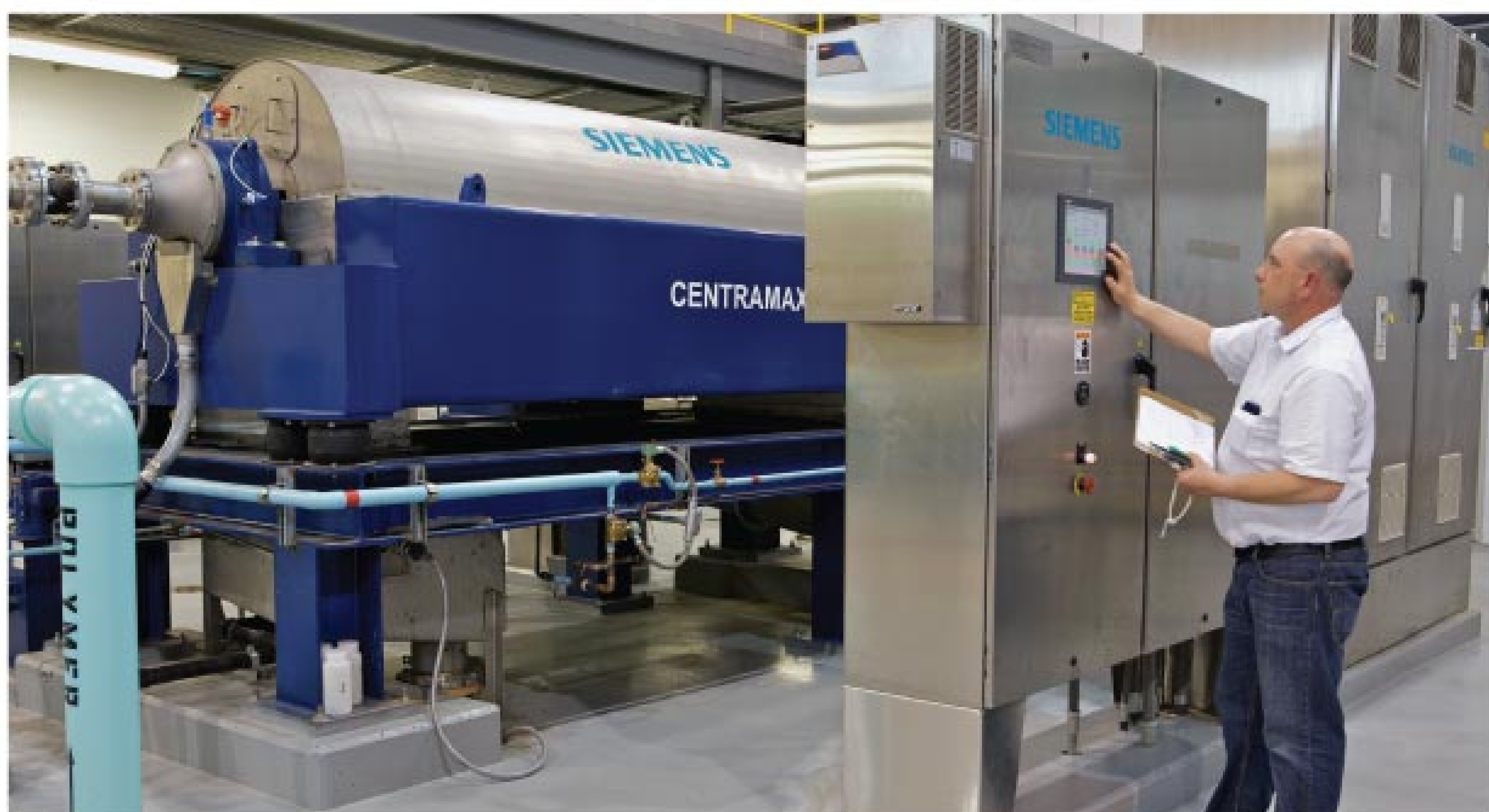
Dave Harris, utility supervisor of operations, makes adjustments to a centrifuge from Siemens Water Technologies at the Grand Rapids facility.
