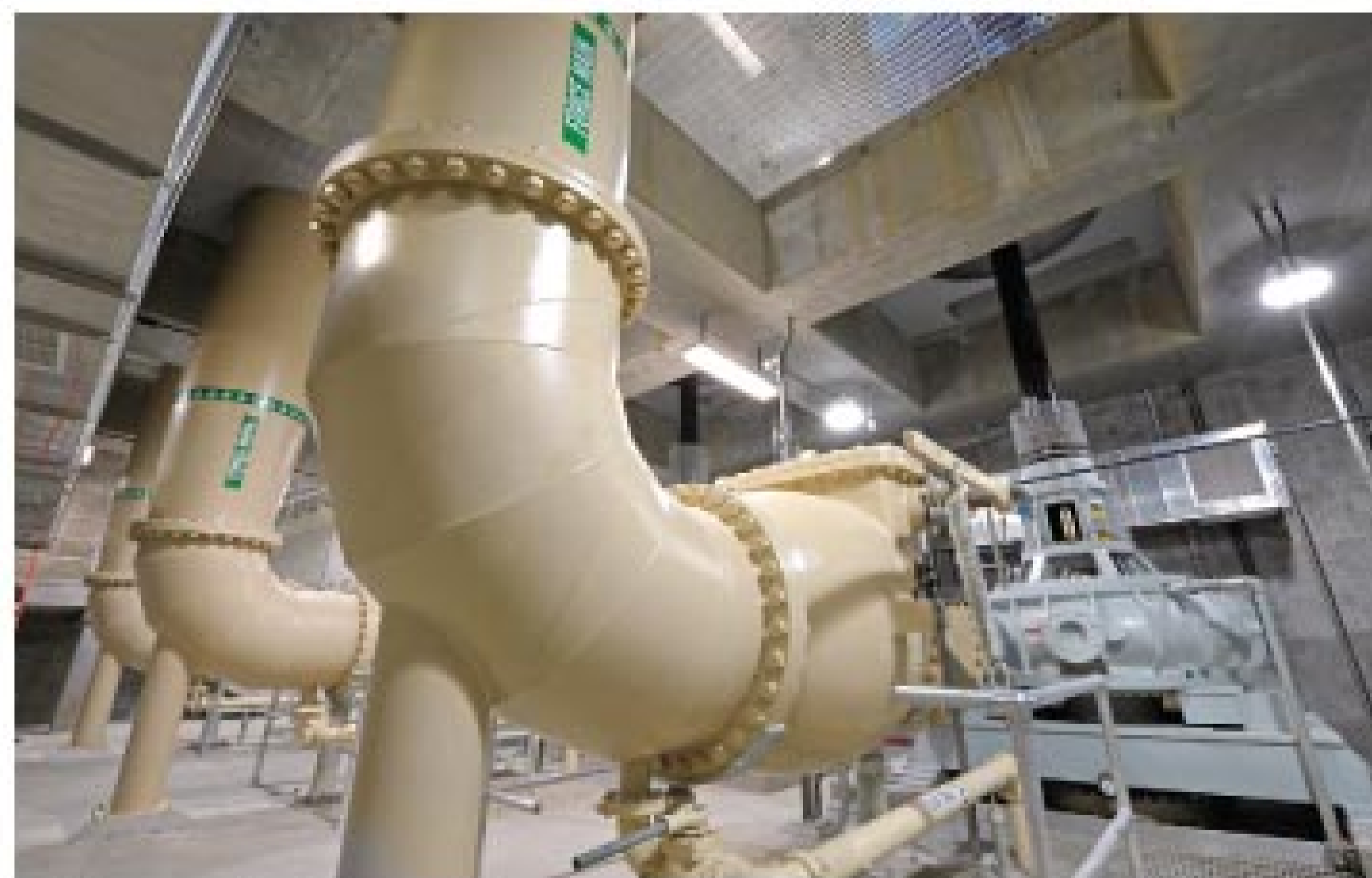
Discharge piping conveys flow from one of six large pumps from ITT Flygt.
