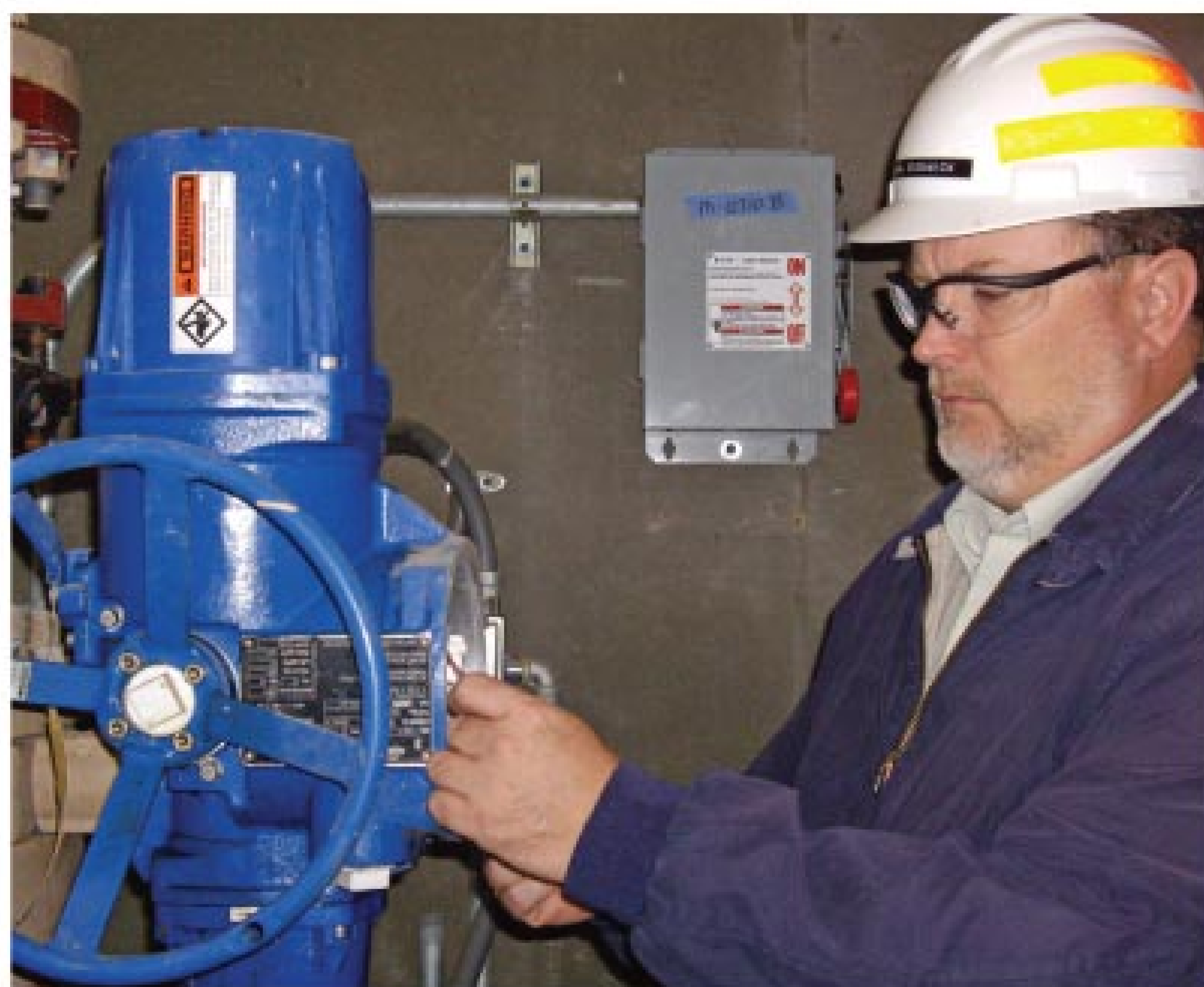
James Didawick inspects wiring in an electric valve.
