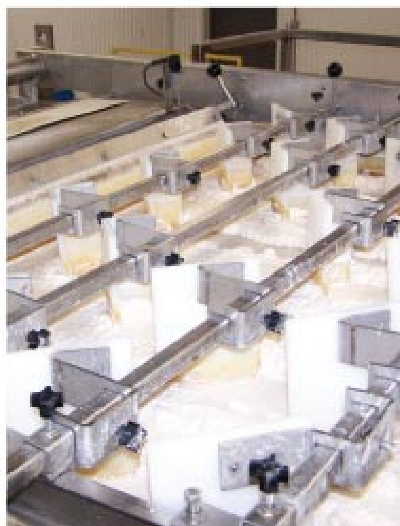
The belt filter press gravity deck in operation.
