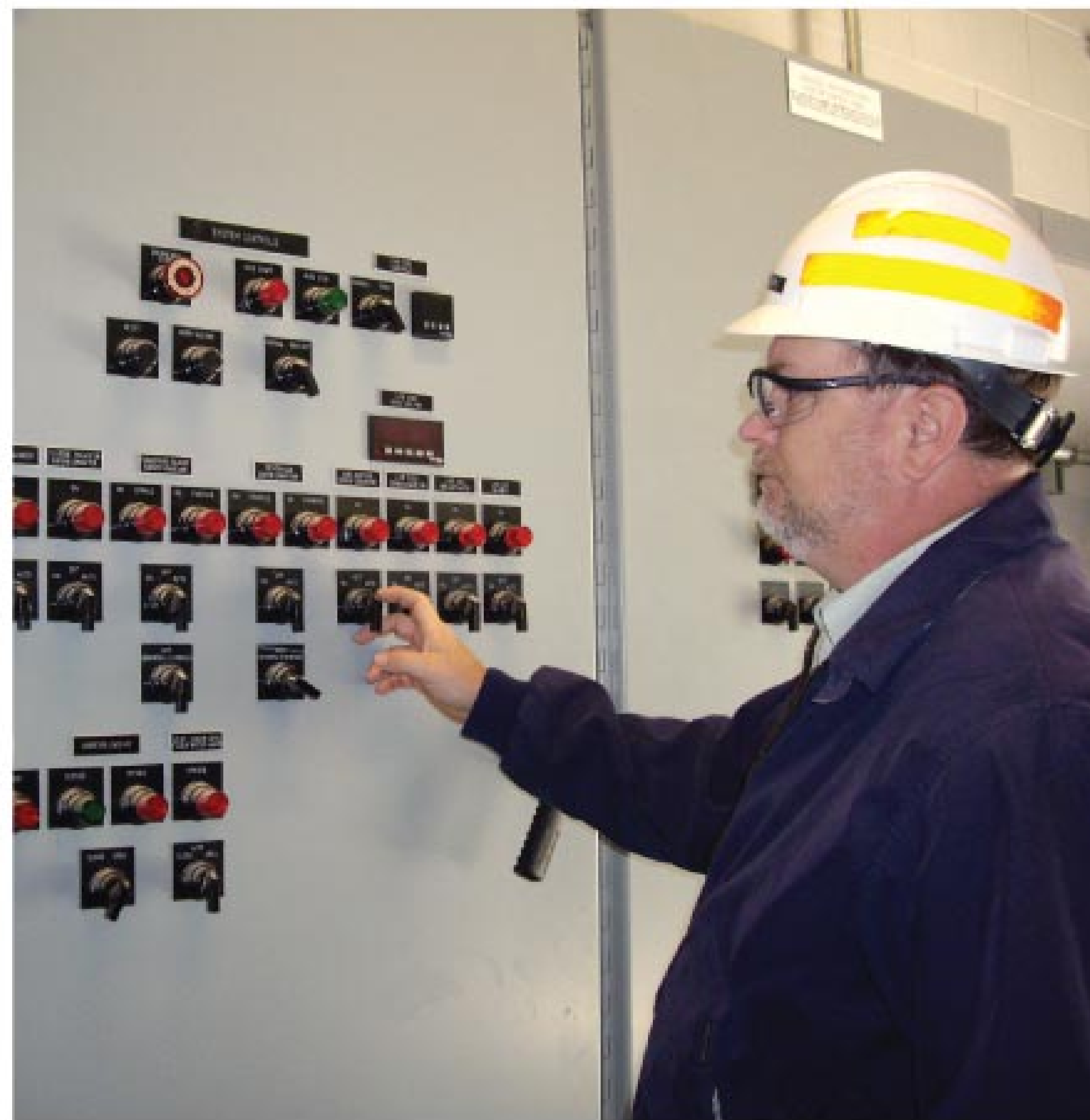
Public Works superintendent James Didawick checks the system control panel in the solids handling building.
