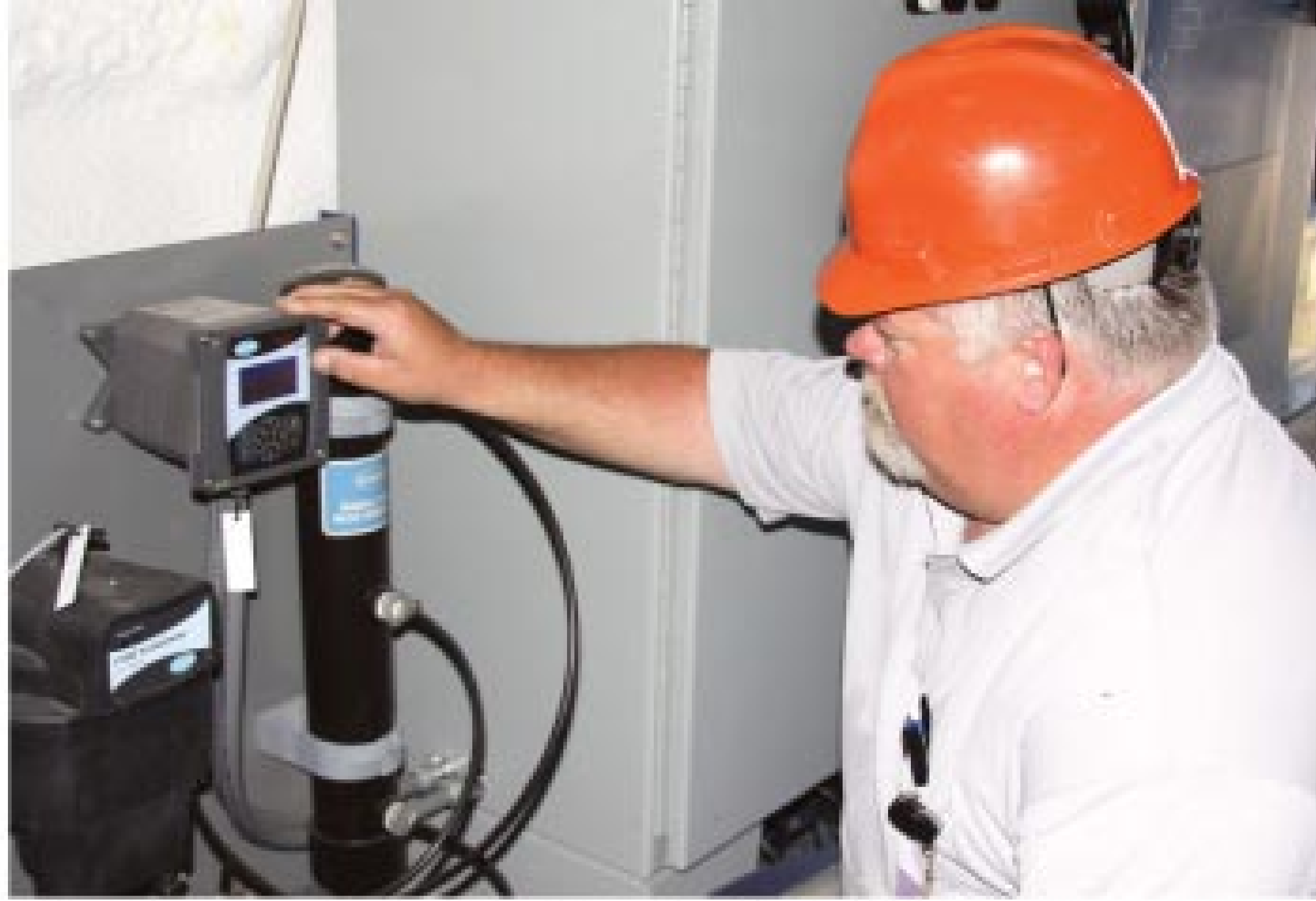
Allen Rhue checks the Turbidometer (Hach) in the main control room for the Summerhouse facility.
