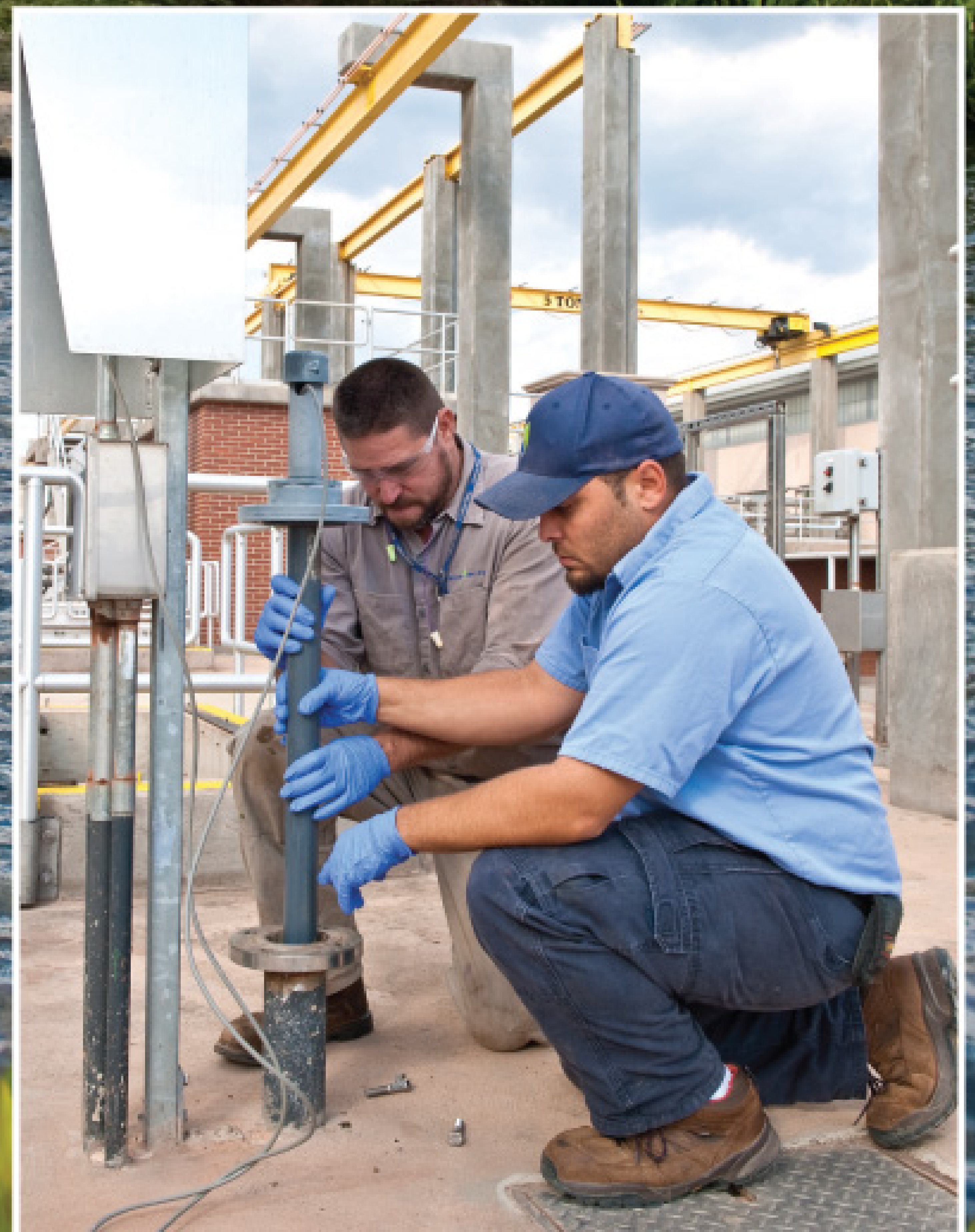
James Marrone and Curt Moore perform maintenance on the plant's five-stage Bardenpho process (Eimco Water Technologies).
