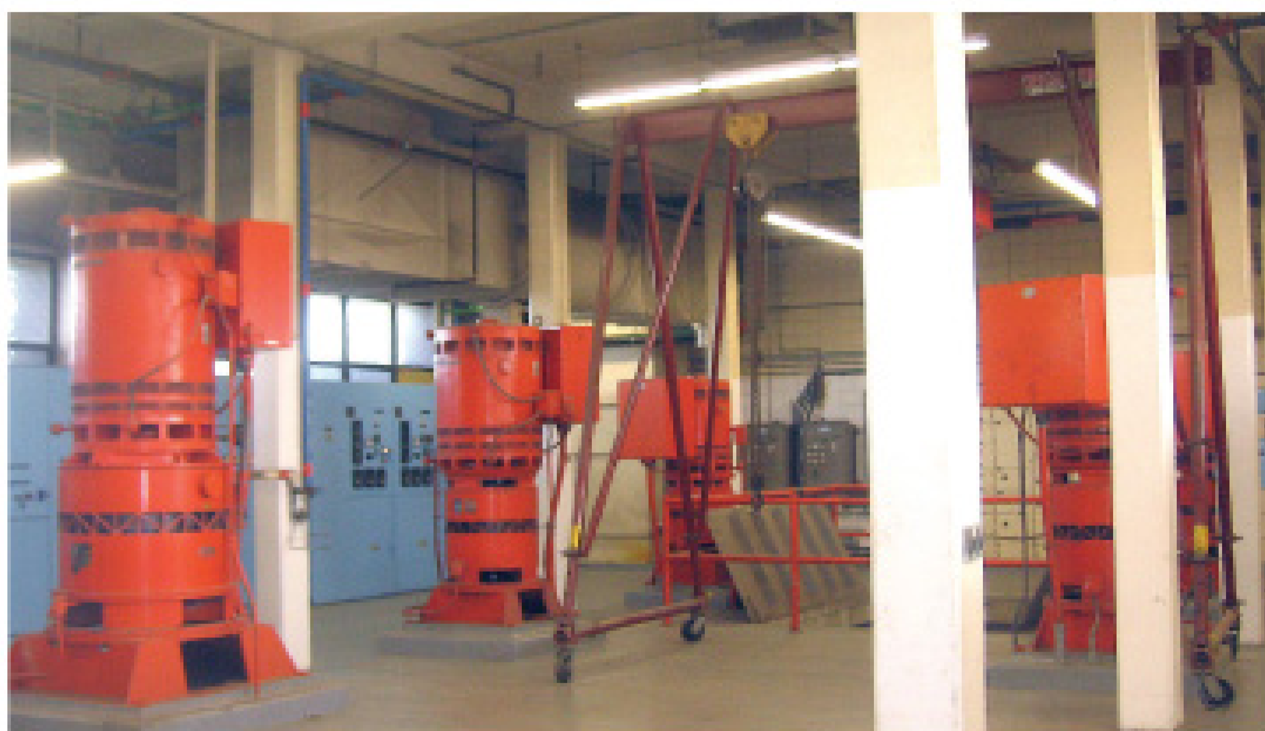
The influent pump room houses five pumps with 60-mgd capacity.
