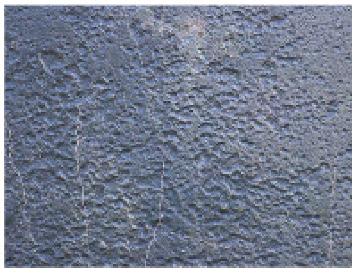
Figure 3: Pump impeller surface showing evidence of cavitation erosion.
