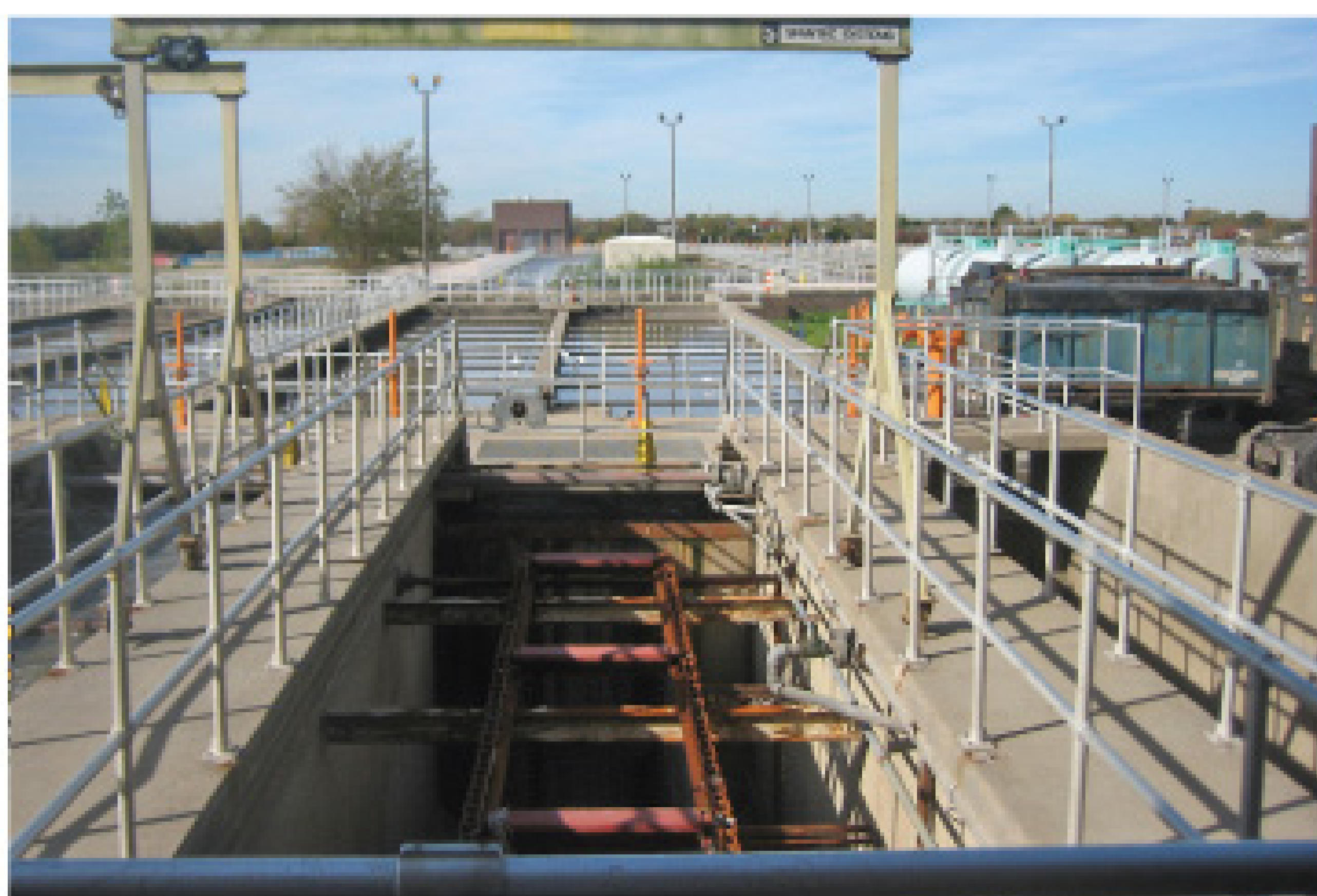
A grit chamber at the Bergen Point facility.
