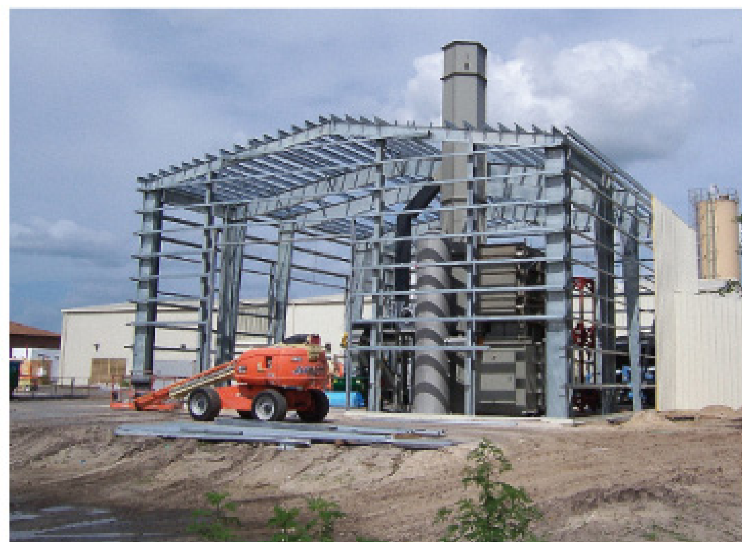
The MaxWest gasification system at the Sanford (Fla.) South Water Resource Center is shown with the enclosure under construction.
