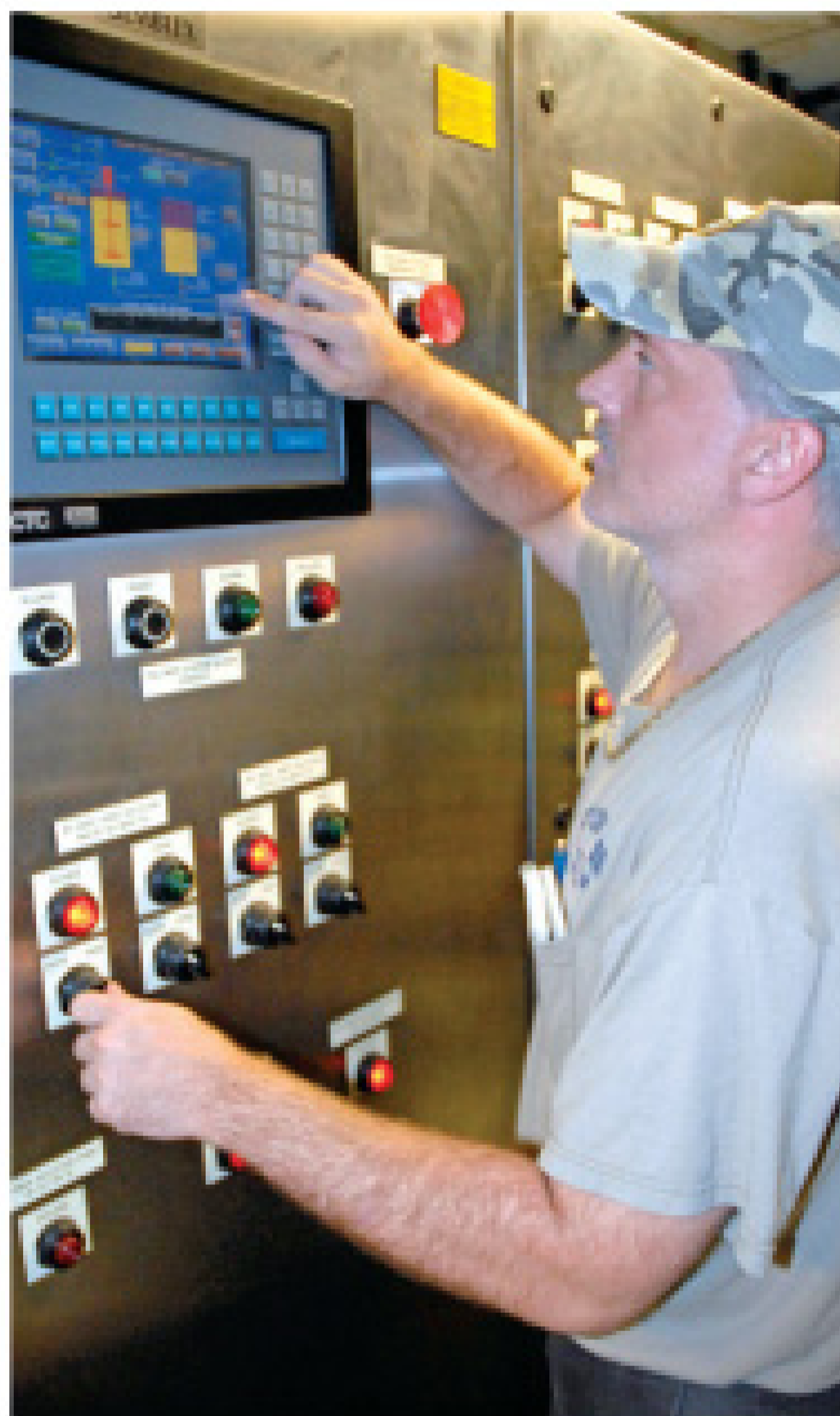
Terry Davis at the centrifuge/polymer control panel.
