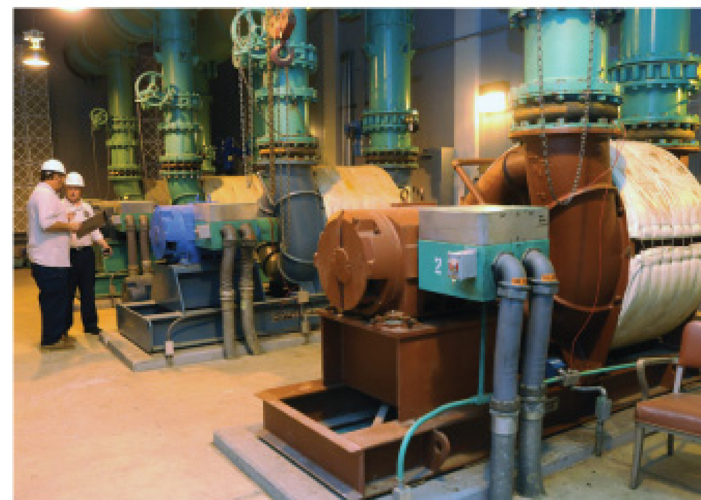
Vincent and Betschel in the treatment plant pump building.
