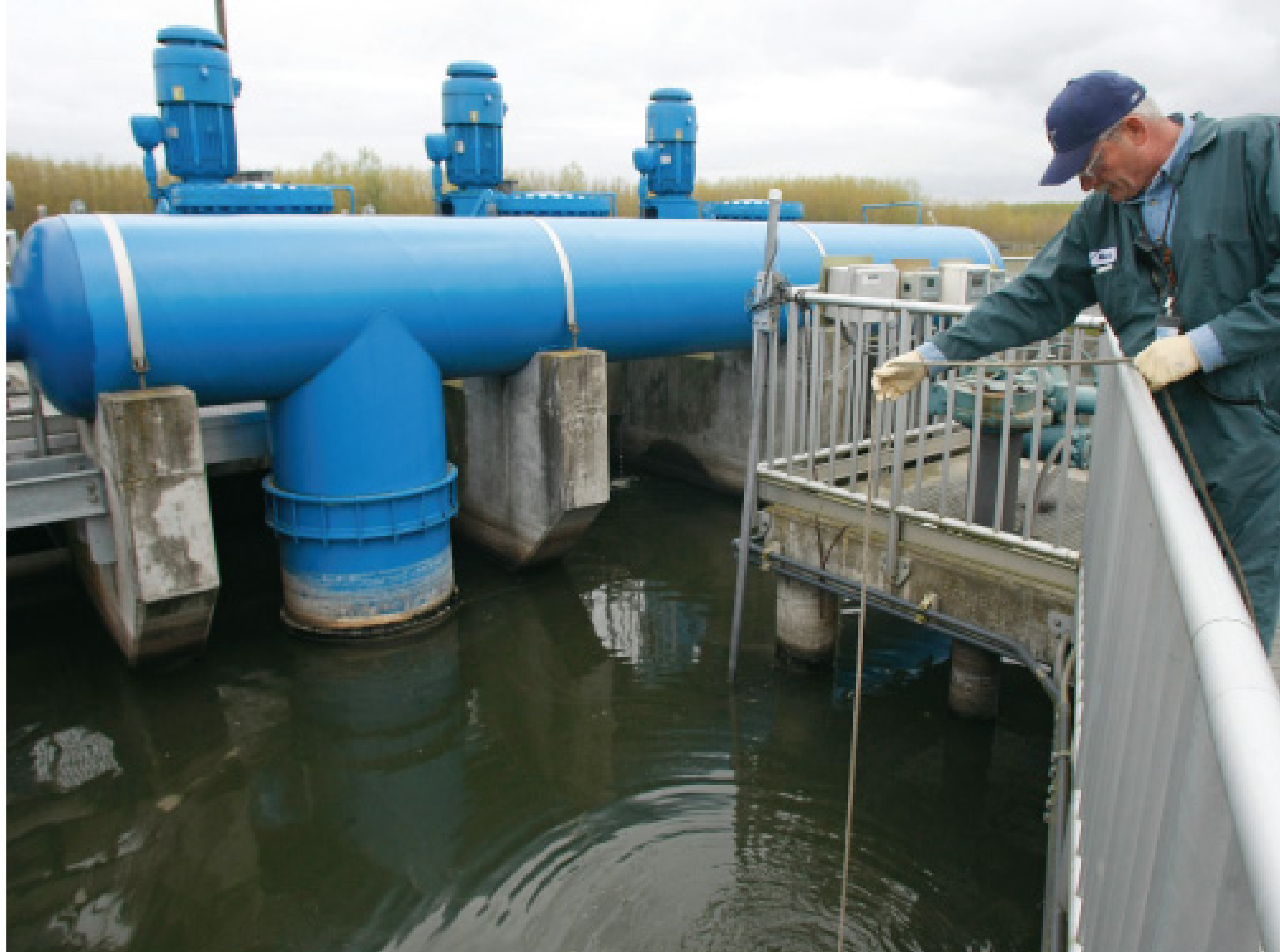
Plant operator Mark Hatzenbuehler takes a one-liter water sample at each pump station, aeration cell, and stage, and verifies the temperature, pH, and DO in the final effluent.
