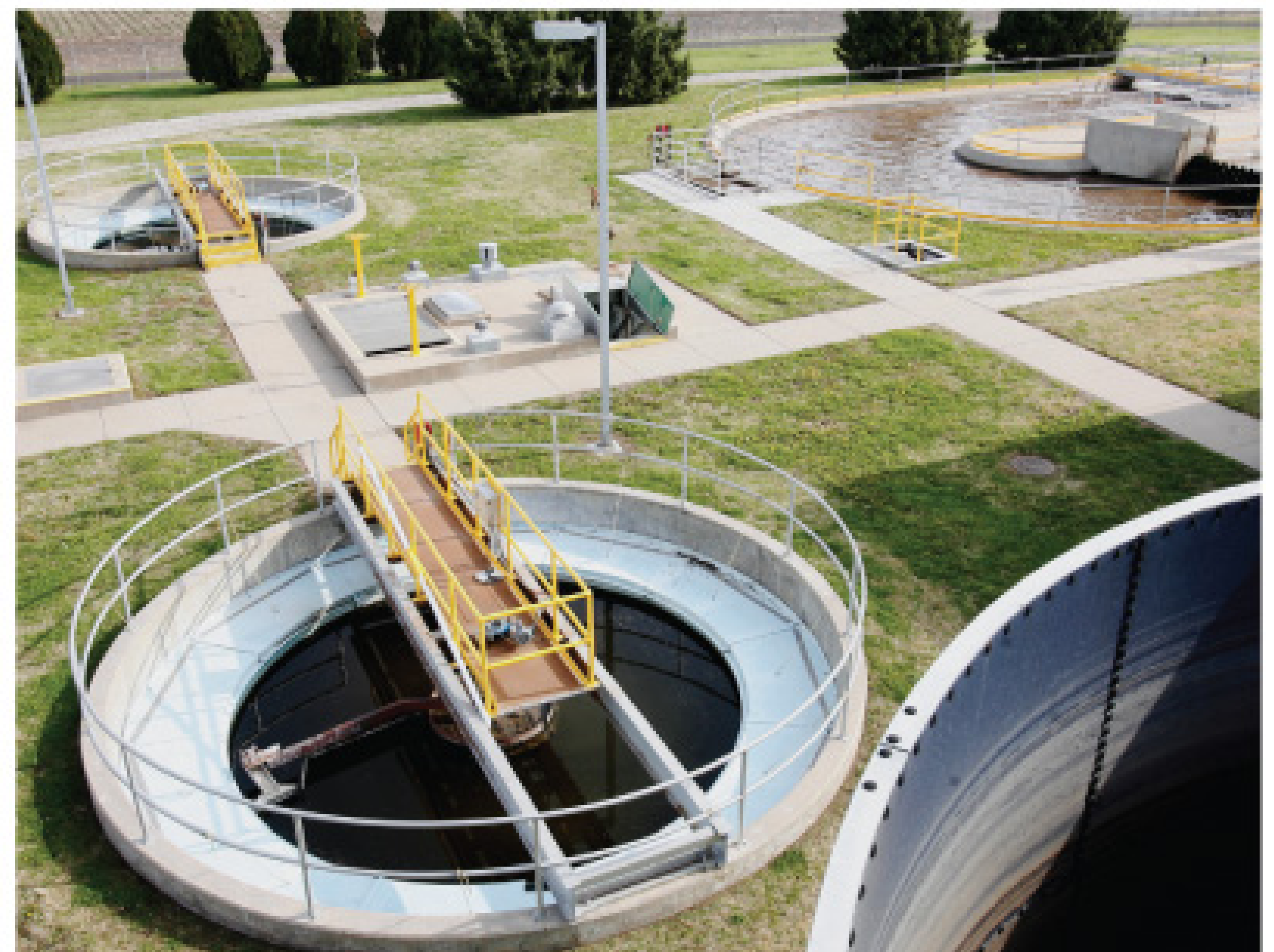
The Sedgwick treatment plant is small, but city officials and plant staff constantly explore measures to enhance its performance.
