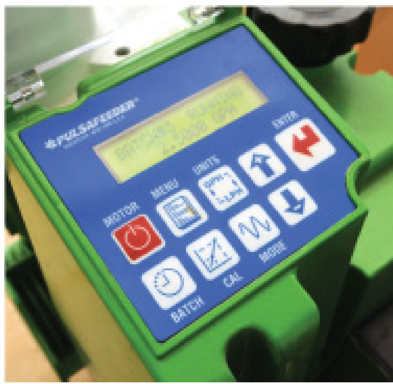
A Pulsafeeder controller (Pulsafeeder Inc.) inside the pumping building.
