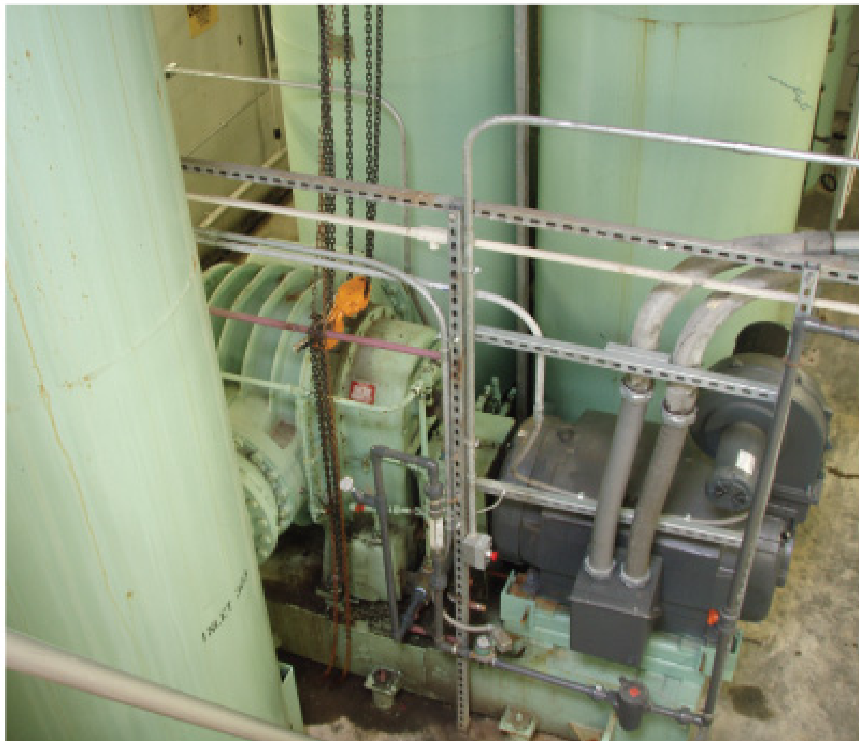
Old motors were replaced with GE high-efficiency motors. Energy-efficient Roots blowers were deployed for the aeration system.
