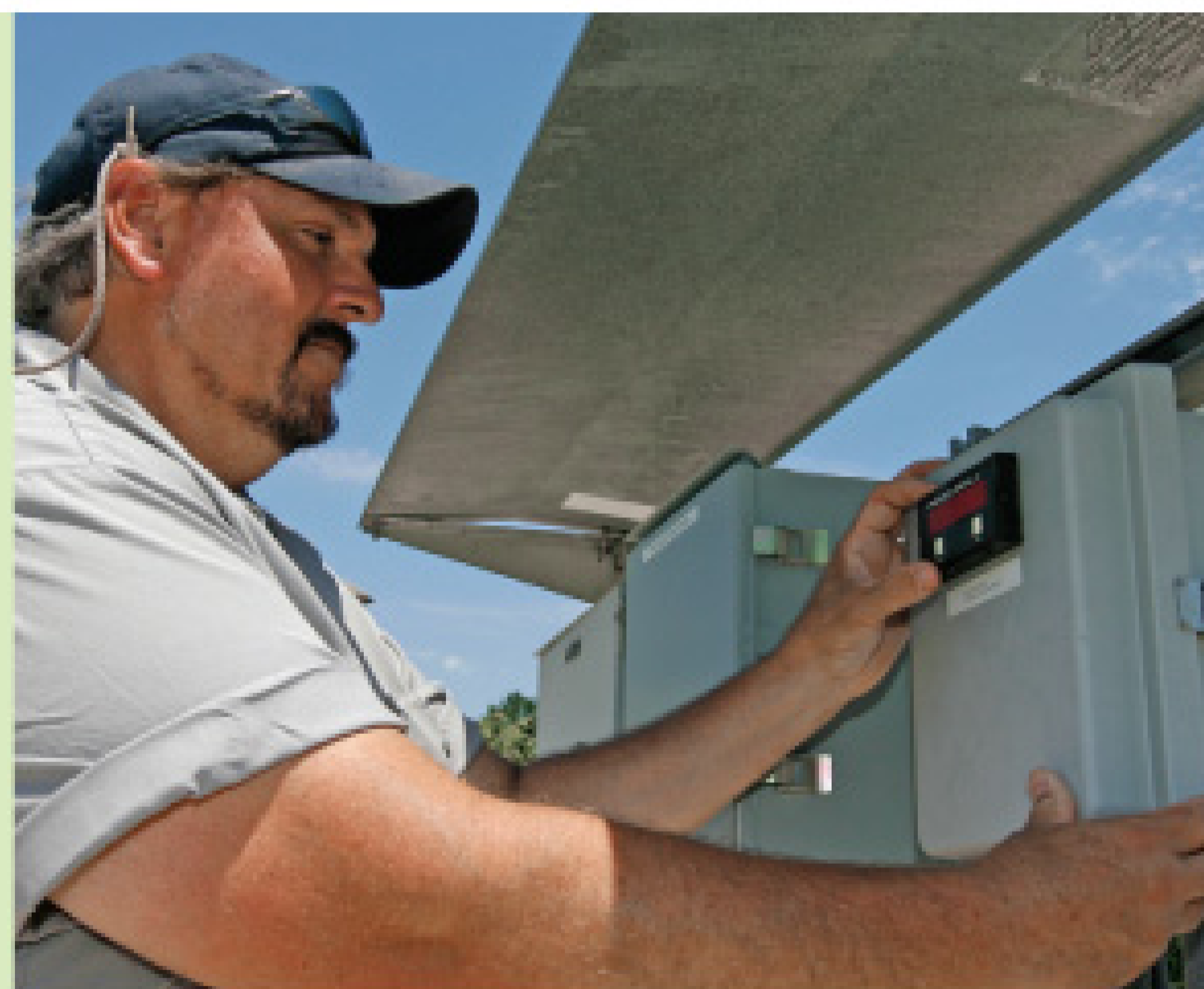
Hricko checks the aeration speed control, a key piece in saving thousands of dollars for the Town of Crewe treatment plant.
