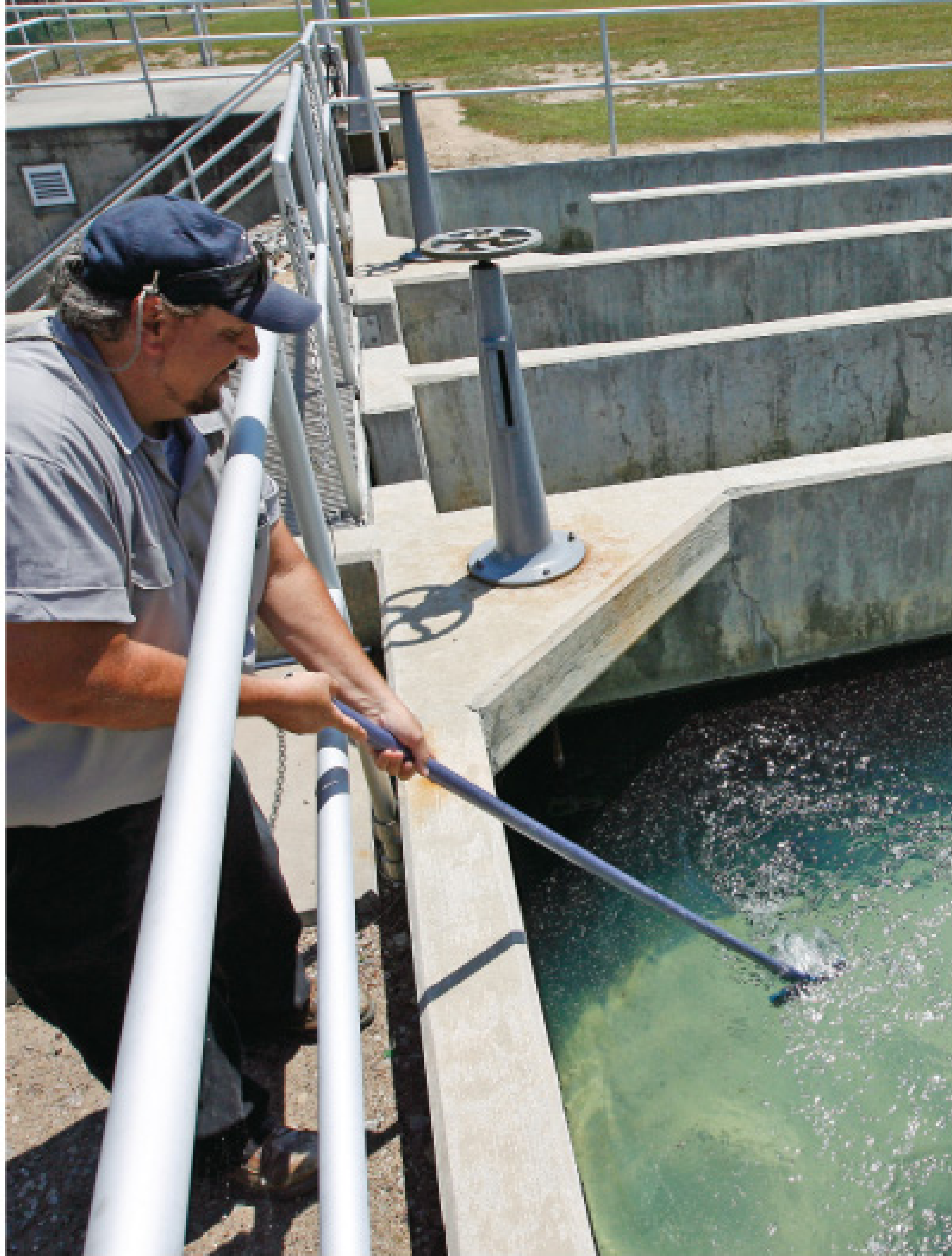
John Hricko shows off the clarity of the water in the chlorine tank.
