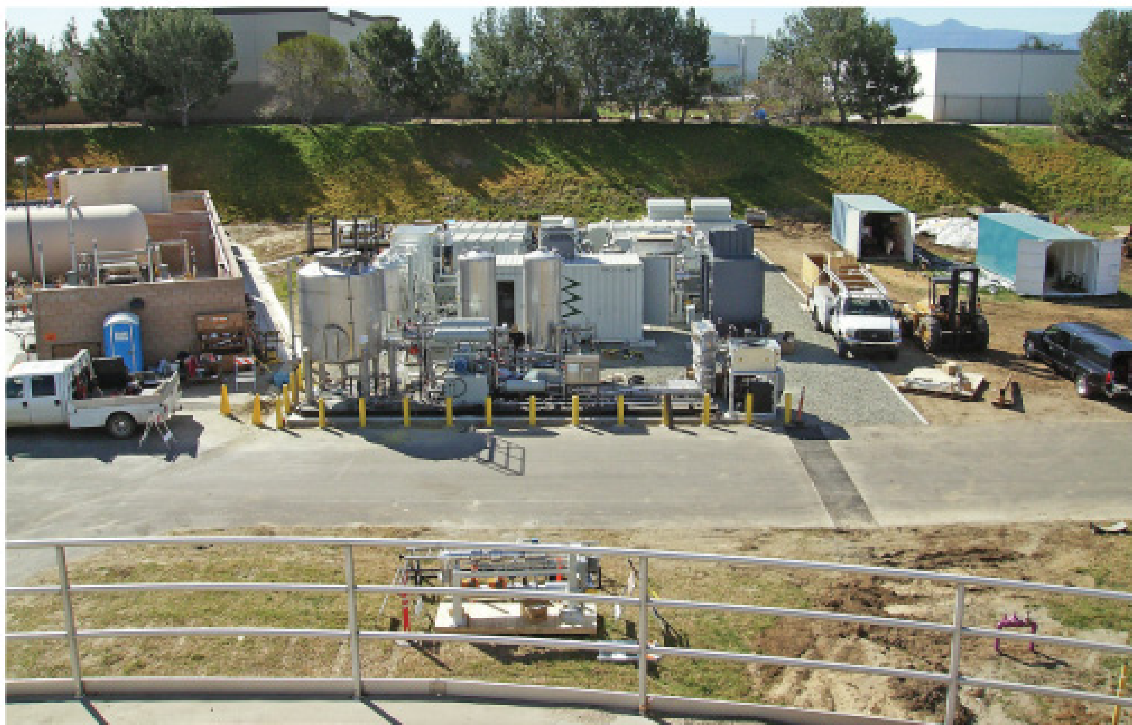
A 1 MW fuel cell cogeneration system, manufactured by FuelCell Energy Inc., went on-line in 2008. The fuel cell runs on 75 percent digester gas and 25 percent natural gas.
