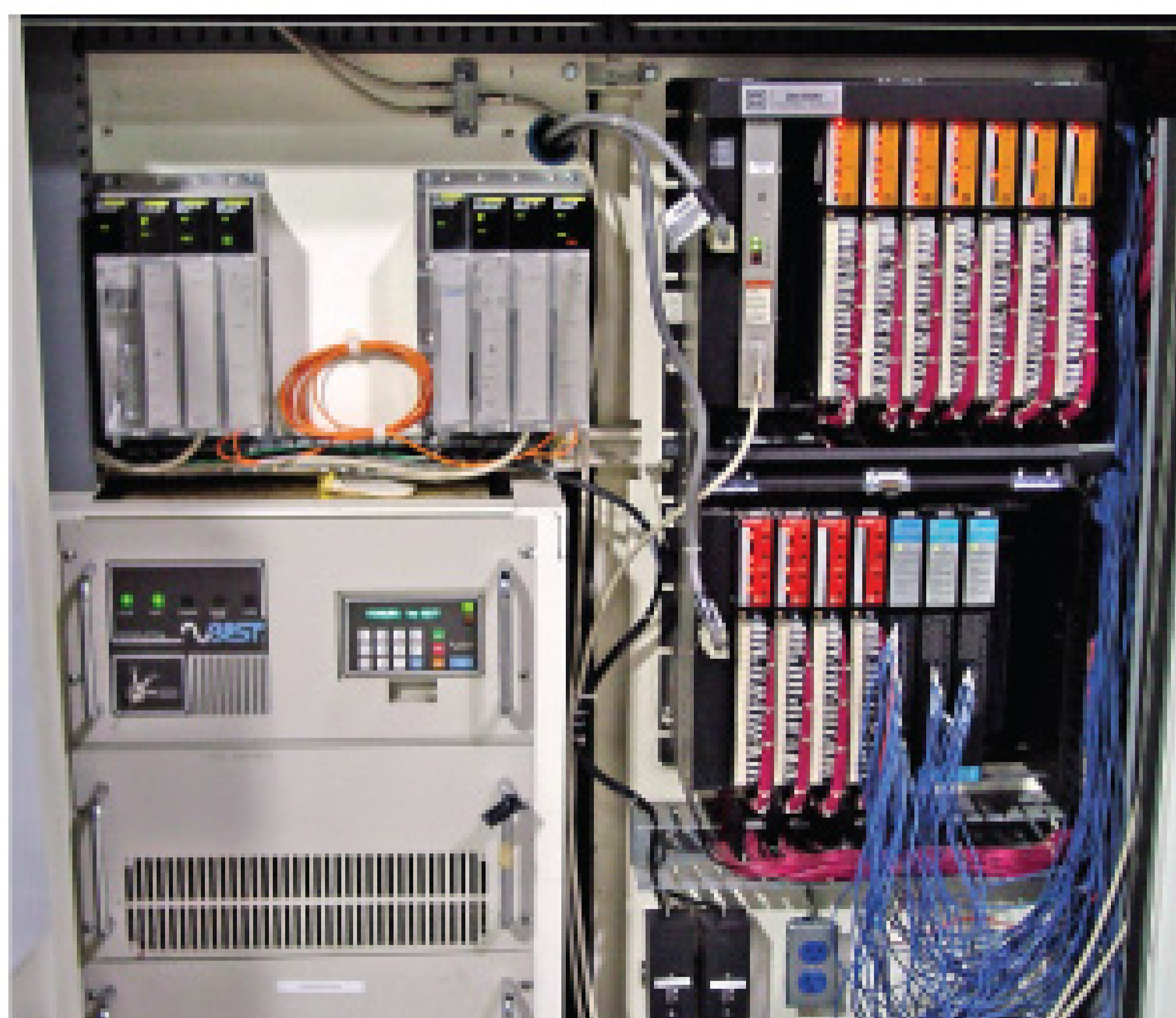
PHOTOS COURTESY OF SCHNEIDER ELECTRIC
