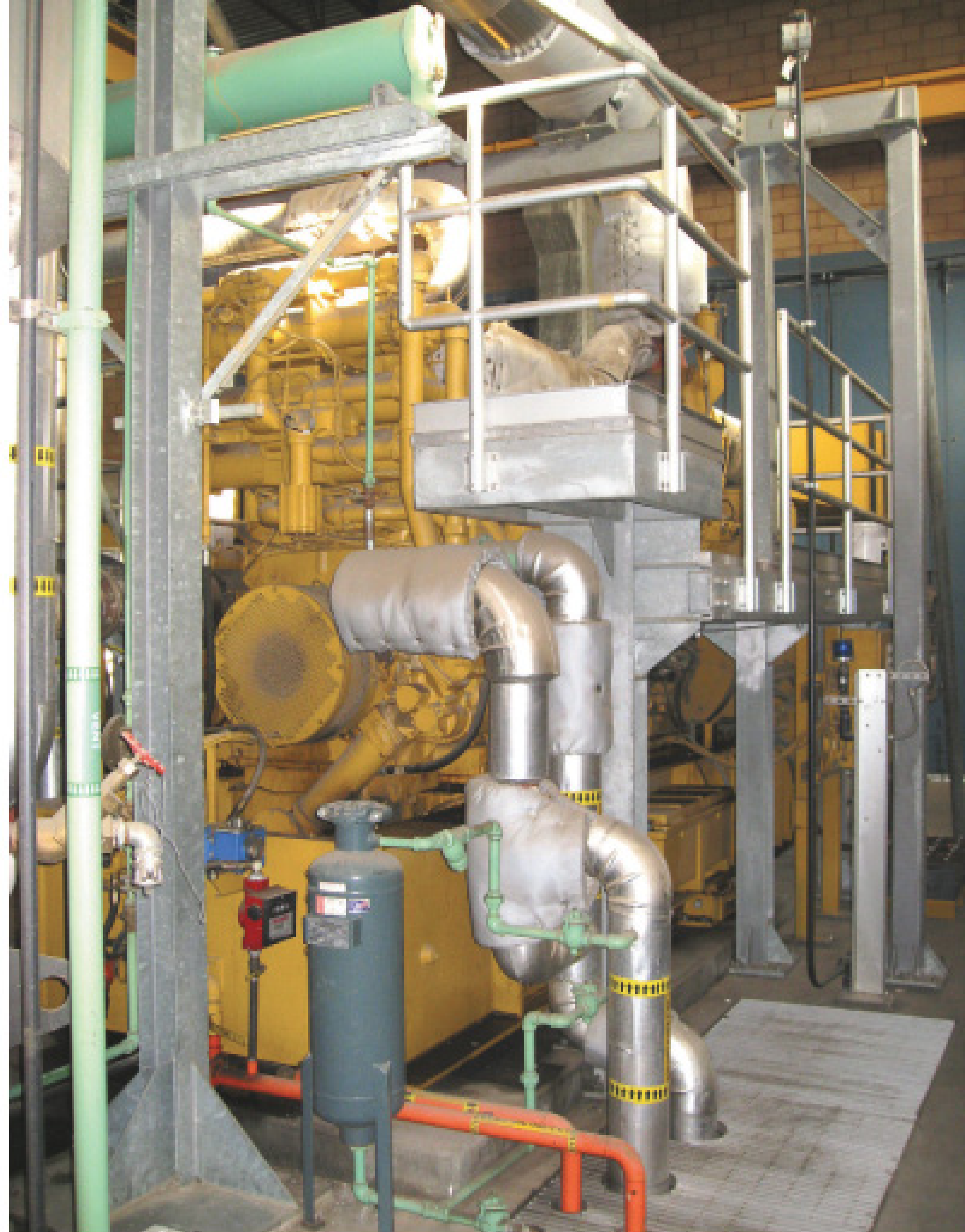
The Riverside plant's combined heat and power facility includes three Caterpillar engine-generator sets, each rated at 1.1 MW. The plant runs two units at near capacity around the clock, and the third serves as a backup. The strategy is to fuel the units with 95 percent digester gas and never more than 5 percent natural gas.
