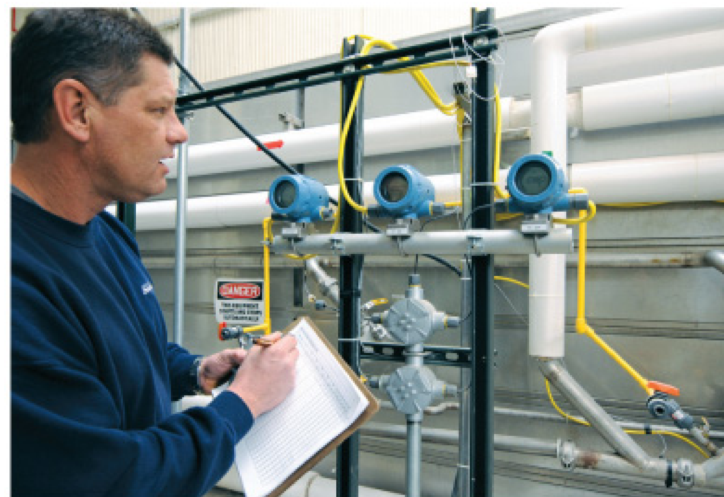
The solids treatment process is highly automated, although assistant plant manager Jordan Kleinsmith and colleagues keep track of process parameters.
