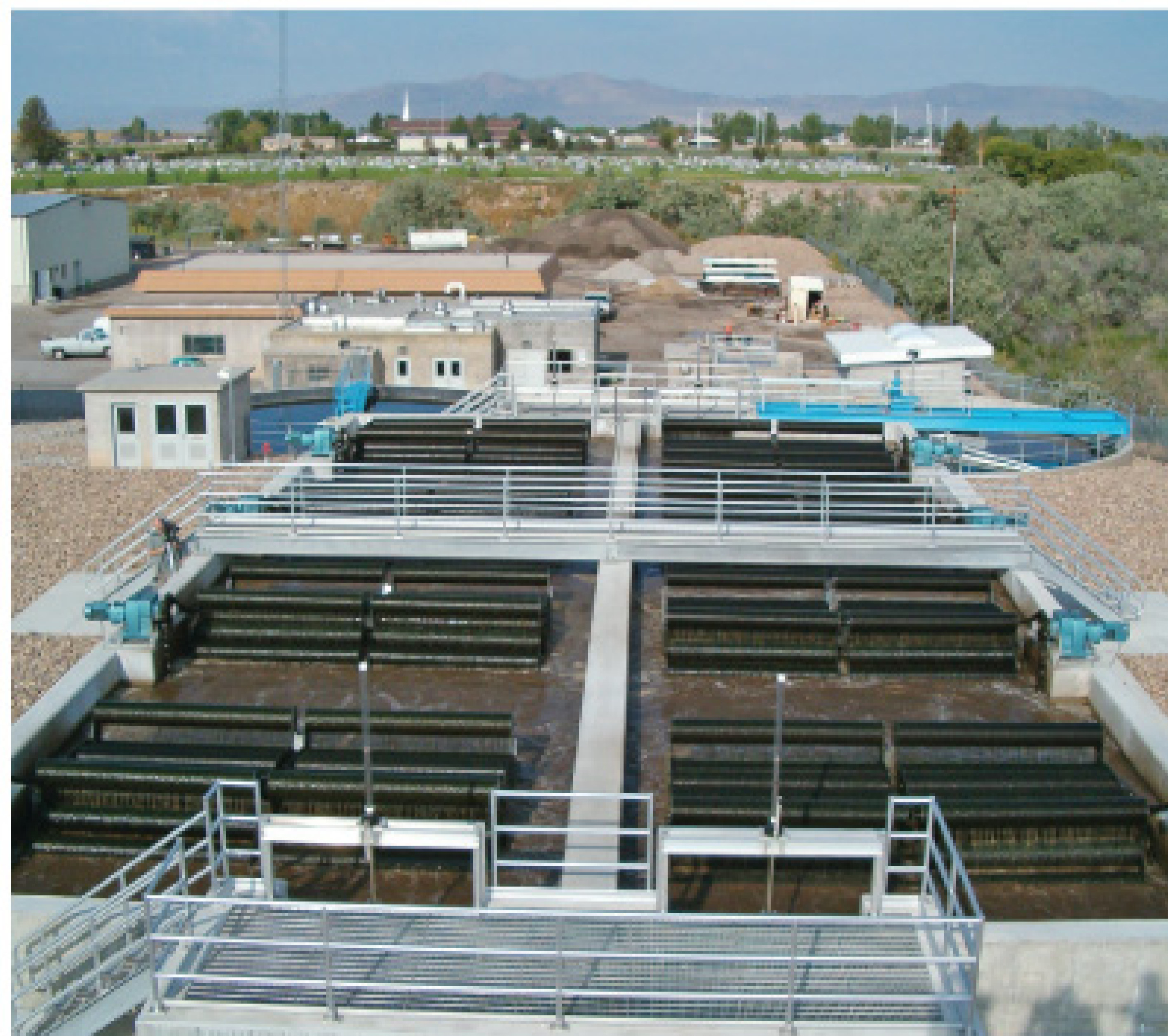
The two 22- by 84- by 17-foot-deep basins containing the STM-Aerotors replaced a 0.5 mgd trickling filter and 1 mgd oxidation ditch.
