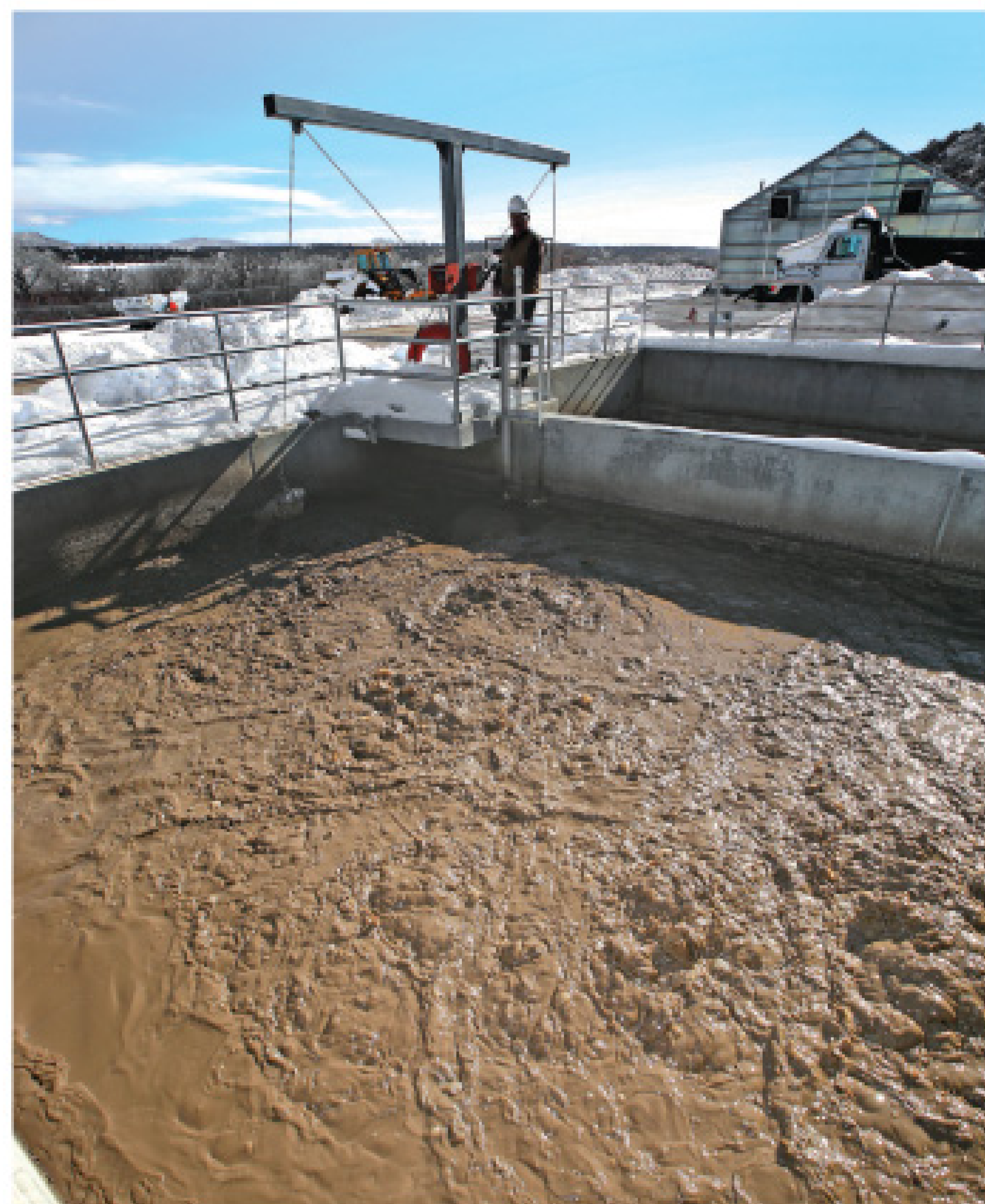
The 130,000 gallons of aerobic digester capacity allows 20 to 40 days of waste activated sludge detention time before dewatering and drying.
