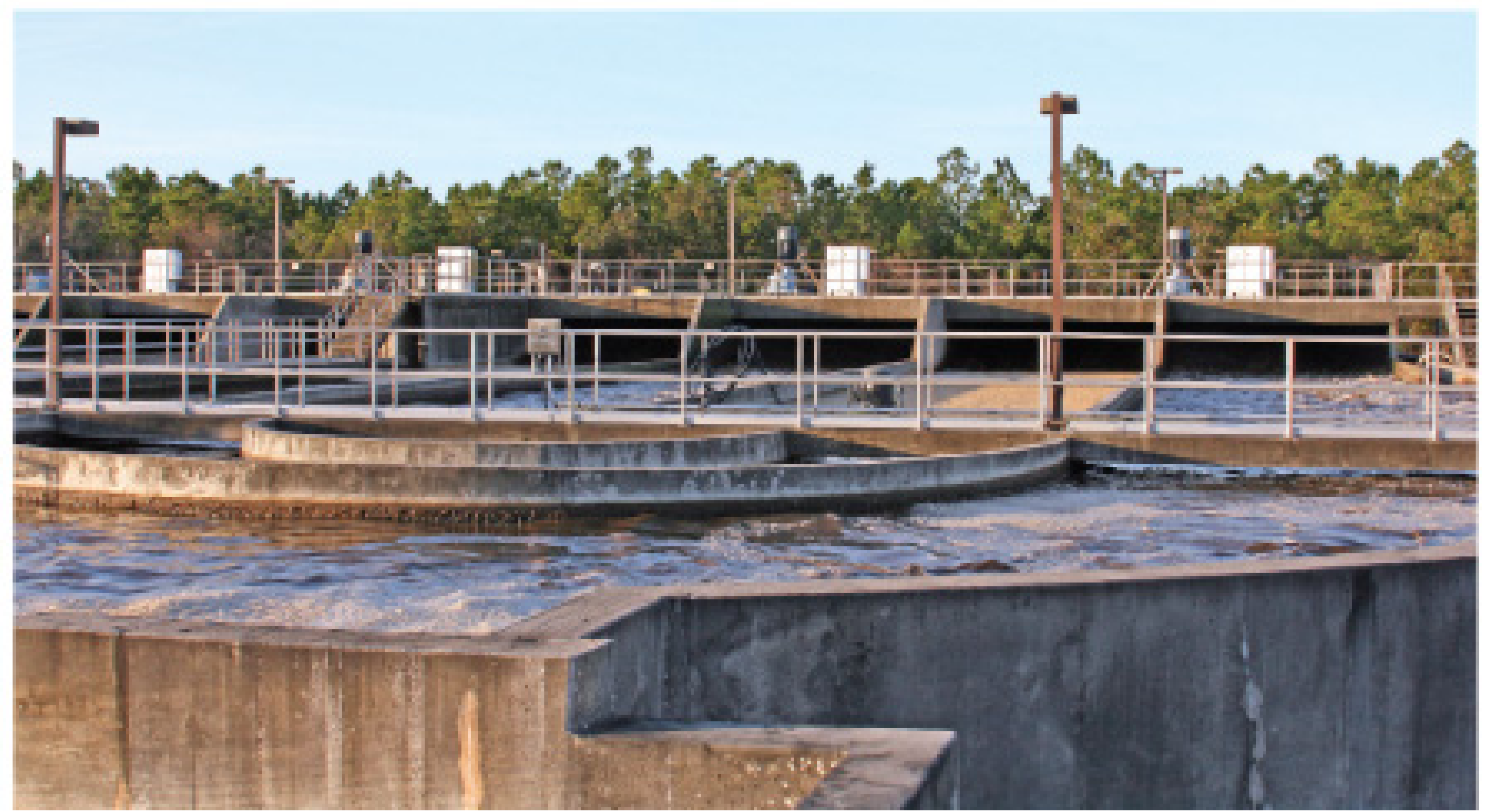
The plant's Eimco carousel oxidation ditch has two independent, four-stage units, each capable of treating 4.1 mgd.
