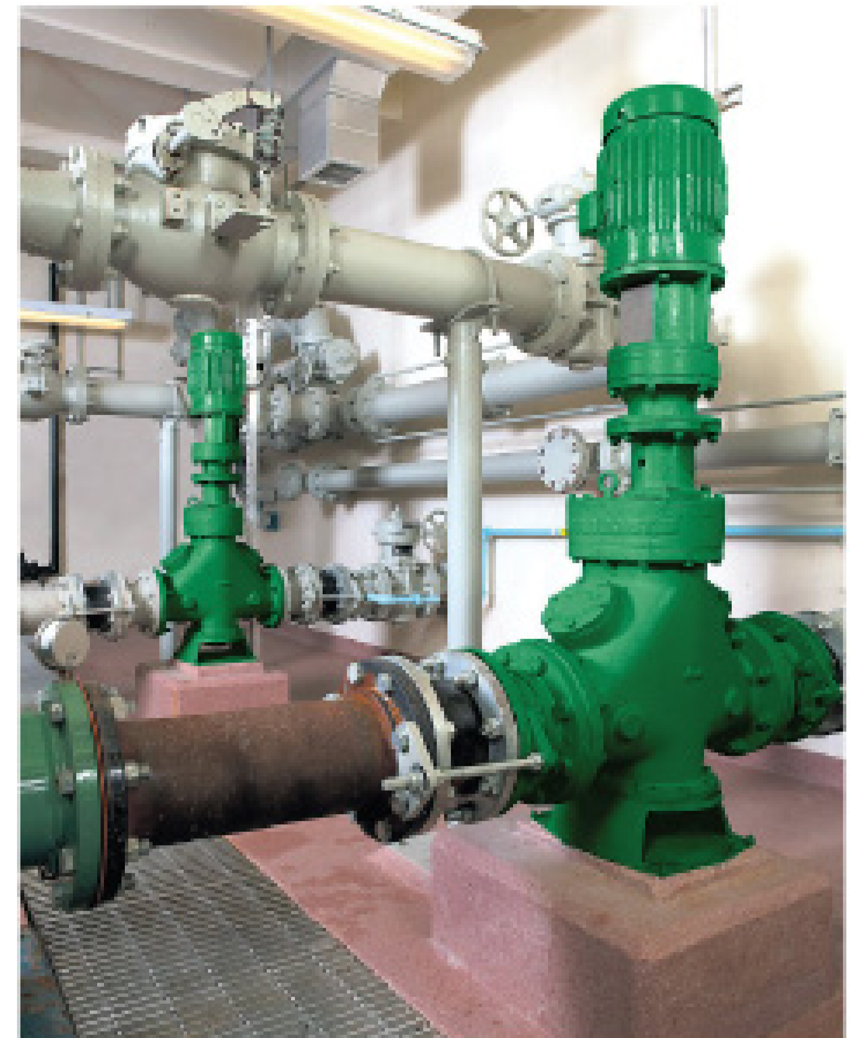
Two Muffin Monster grinders (green) are placed in front of the transfer pumps to grind solids, rags and trash so that they flow harmlessly through pipes and pumps. (Photos courtesy of JWC Environmental)
