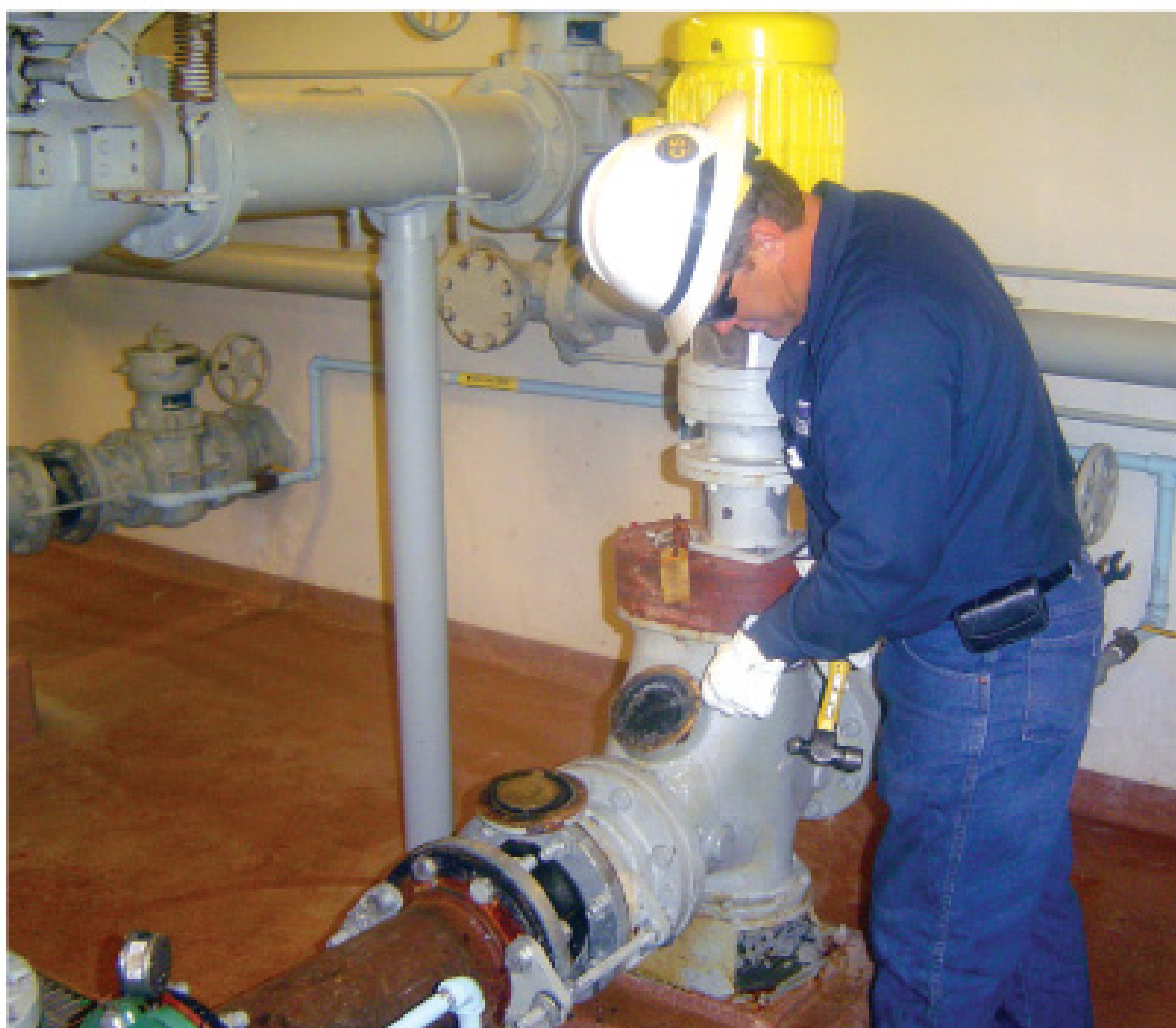
Mechanic Steve Harris works on removing a screwdriver before it enters the blades and causes damage. The grinder unit sounds an alarm during the rare occasions when it cannot grind through an object.
