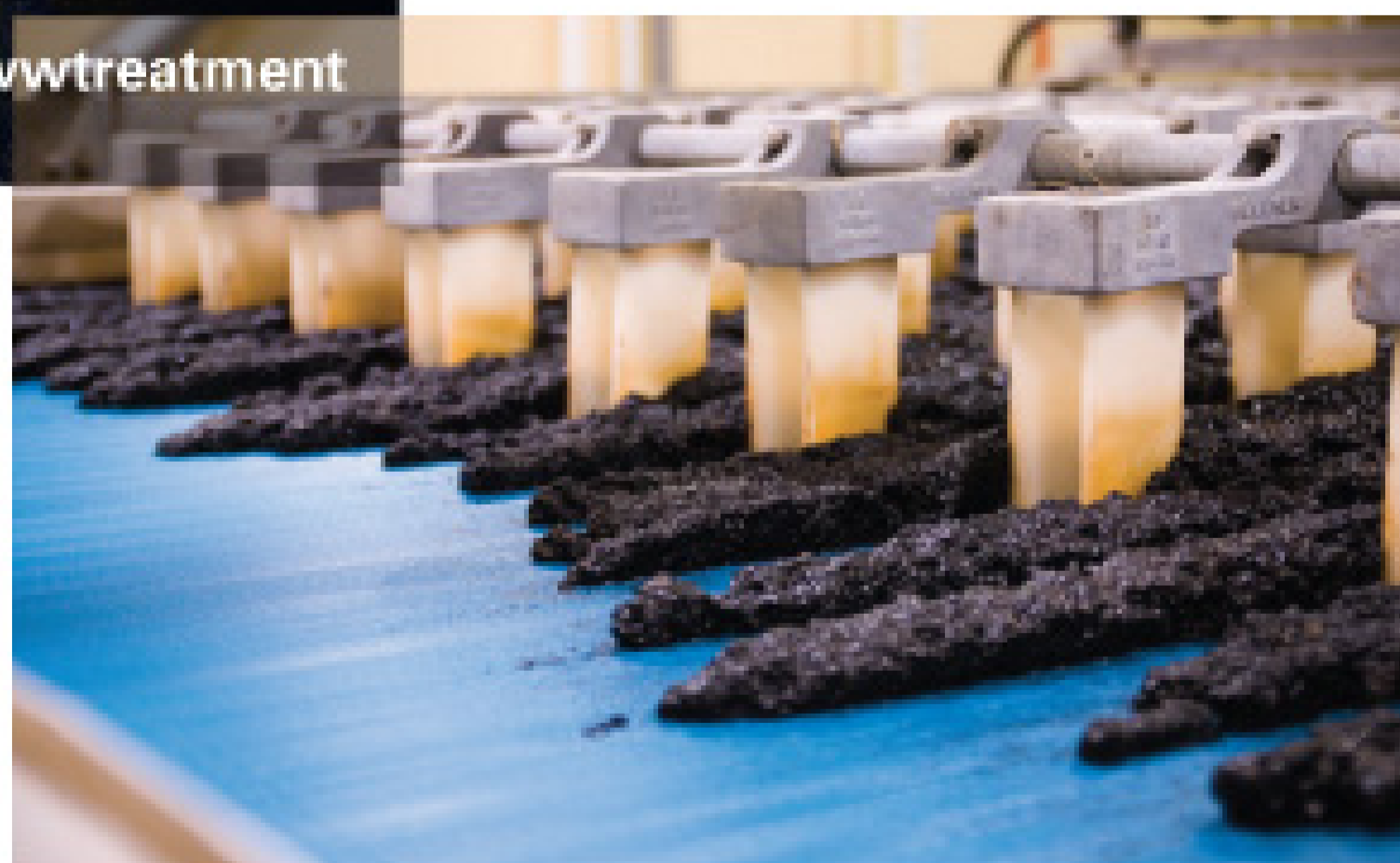
Feed sludge on a belt filter press for dewatering.
