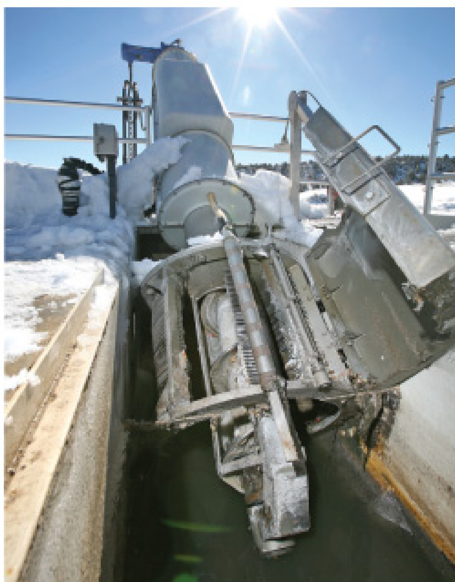
A Rotamat fine screen from Huber Technology does duty at the plant headworks. Large solids are captured on the screen, then washed off and deposited in a trash bin.
