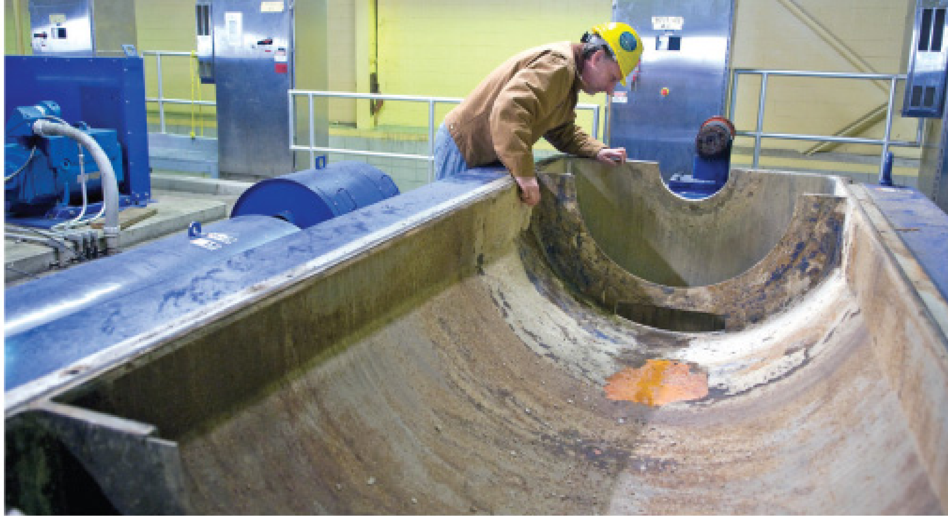
Robert Bates, wastewater process manager-biosolids, inspects a centrifuge that has been dismantled for repair.
