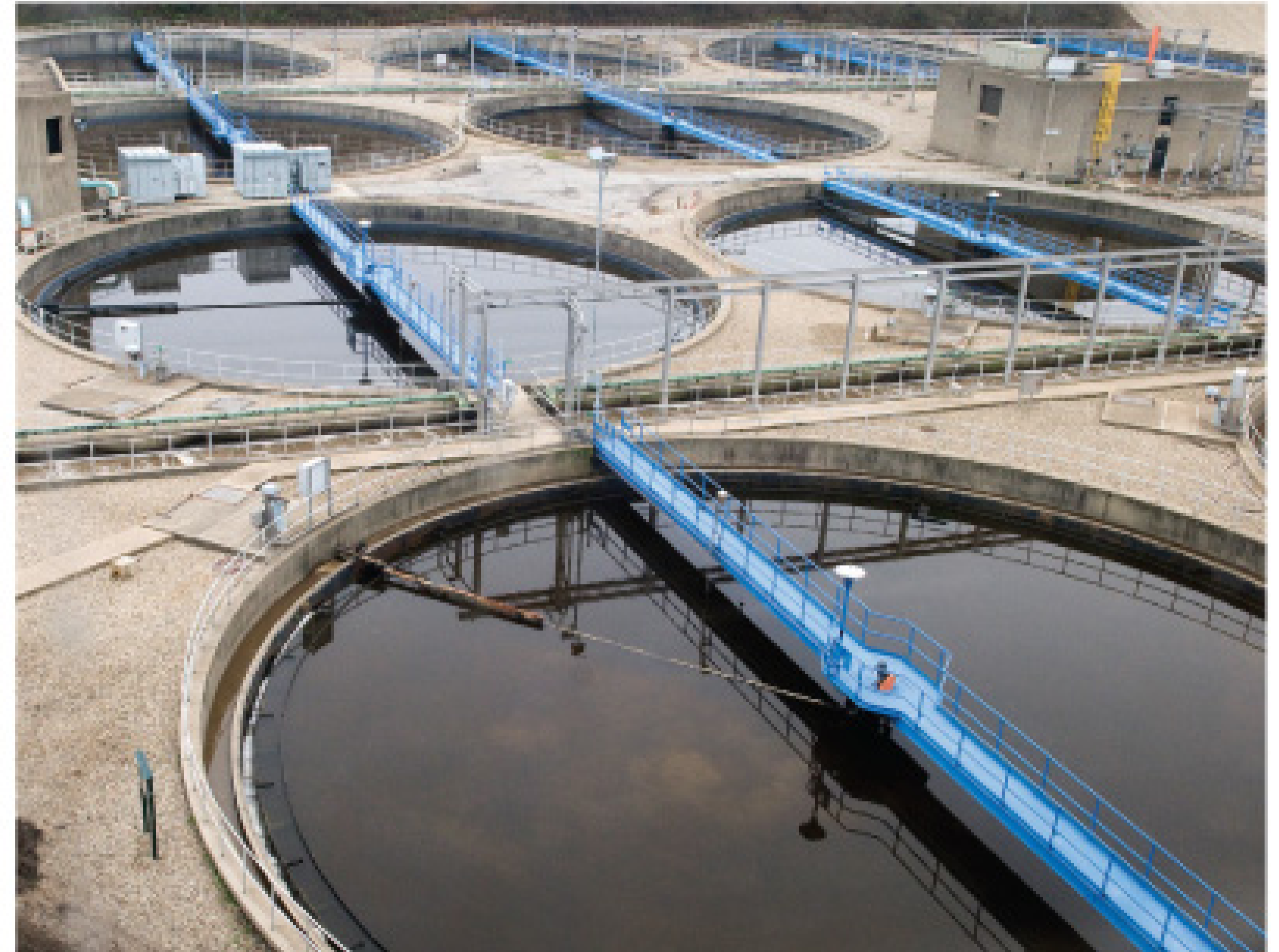
Secondary clarifiers at the Morris Forman treatment facility in Louisville.
