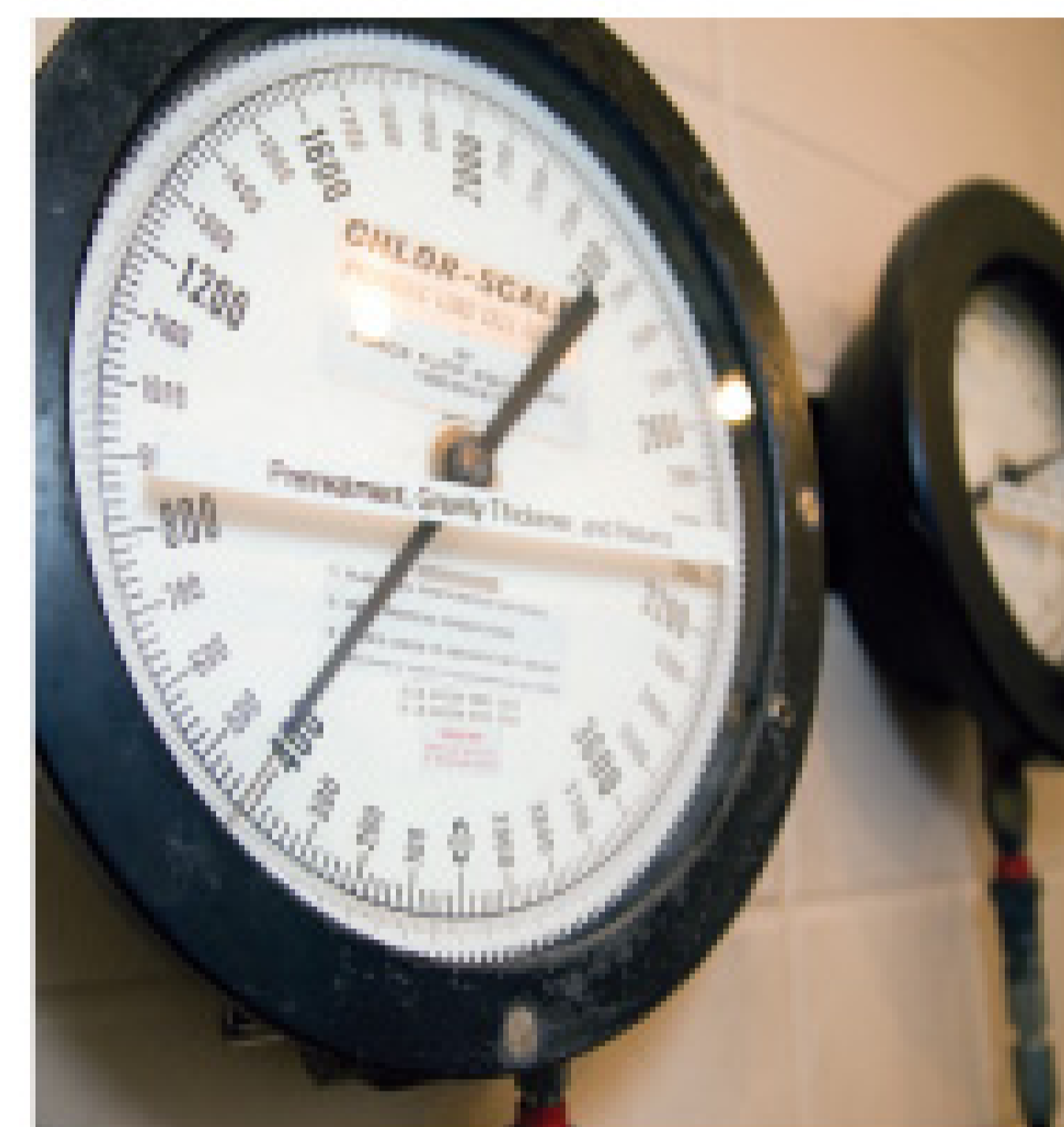
A scale from Force Flow Inc. is used to measure the chlorine gas in cylinders.
