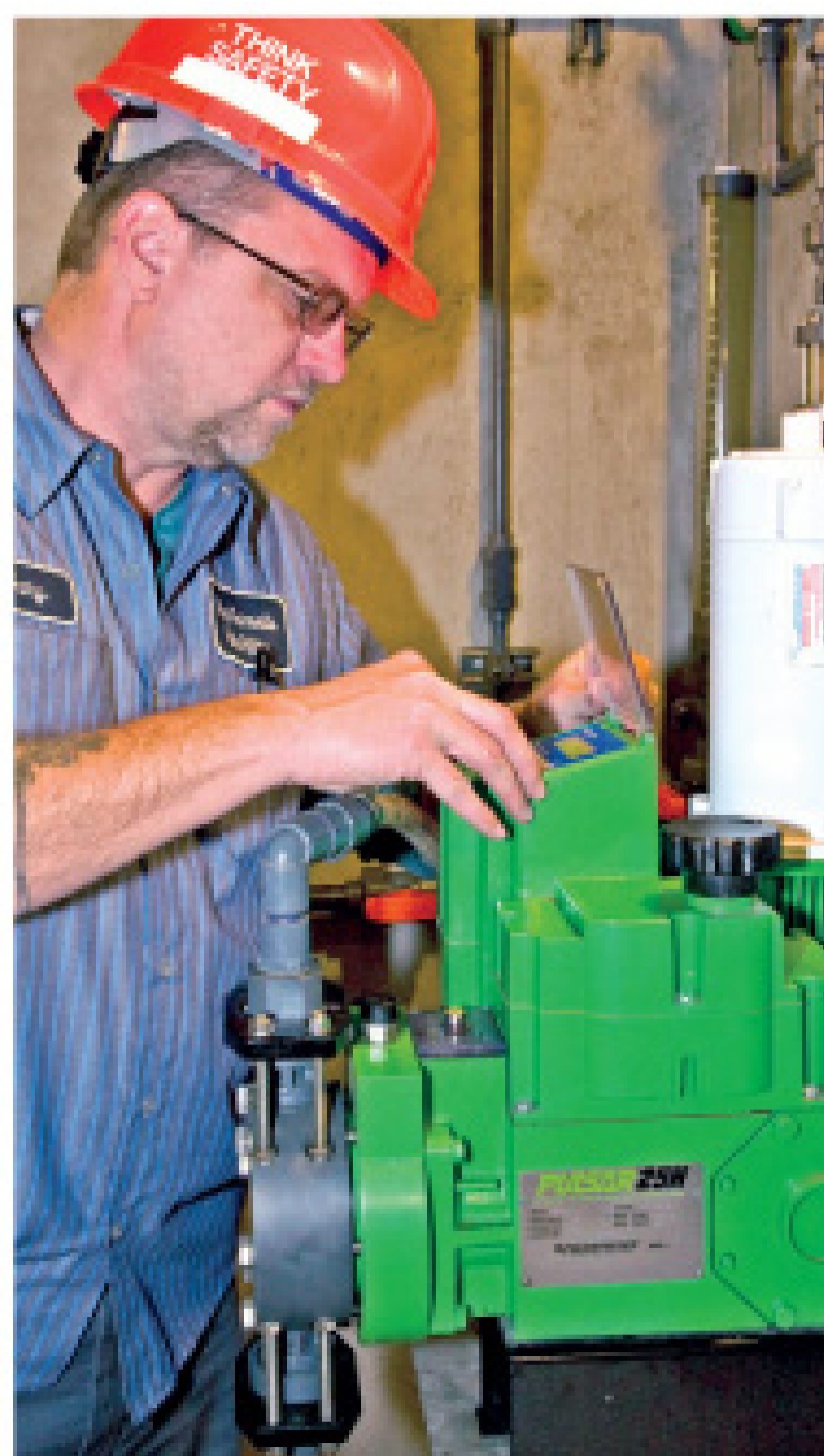
Gary Ford, lift station technician from the maintenance division, checks chemical pump operation on a Pulsafeeder hydraulic diaphragm metering pump at lift station 14.
