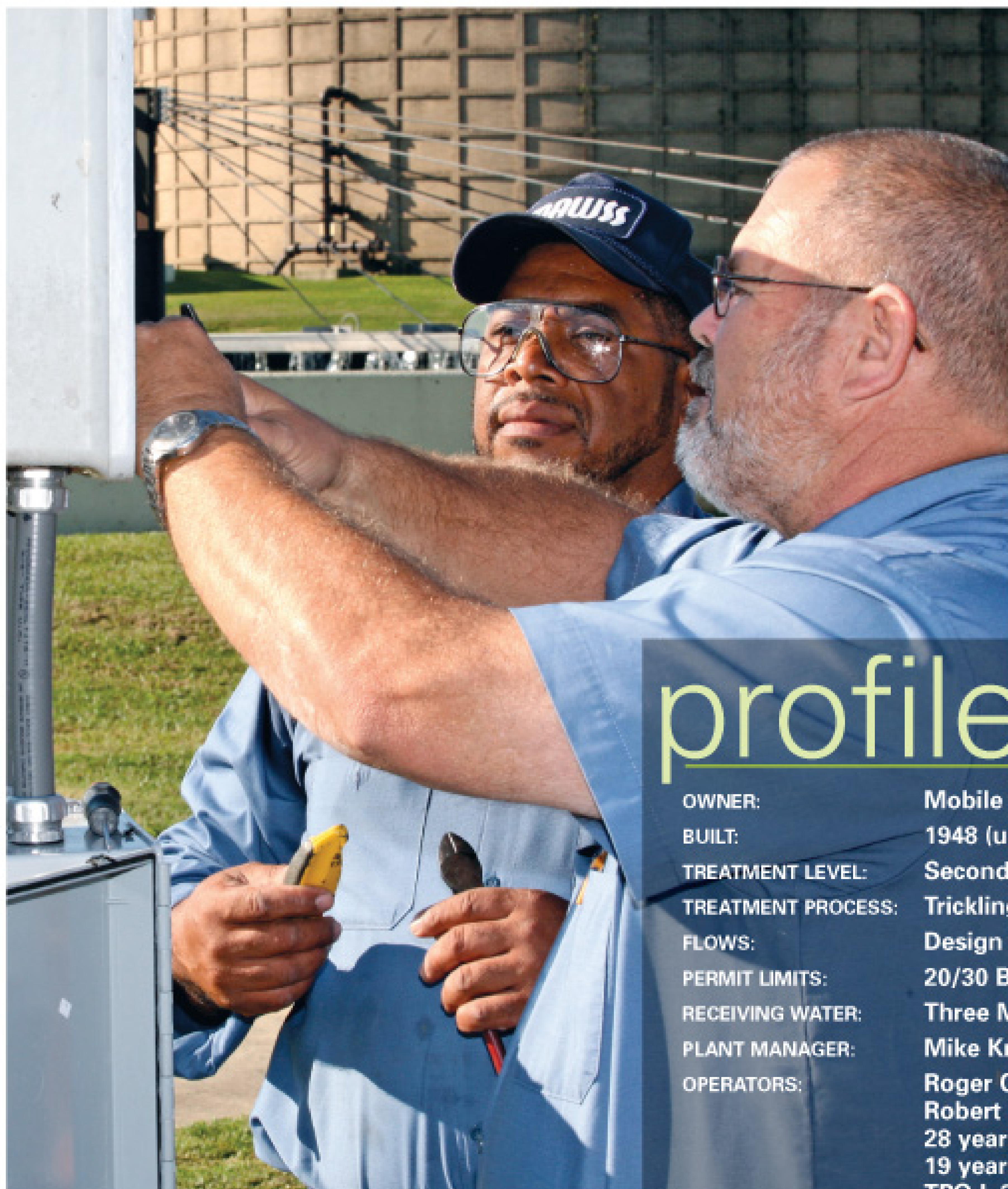
Wallace Bettis (left) and Roger Carlisle install a surge protector on a flow meter. (Photography by Lyle Ratliff)
